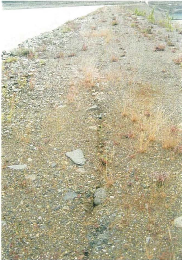
Above: Tension crack near centreline of Intermediate Dam.
