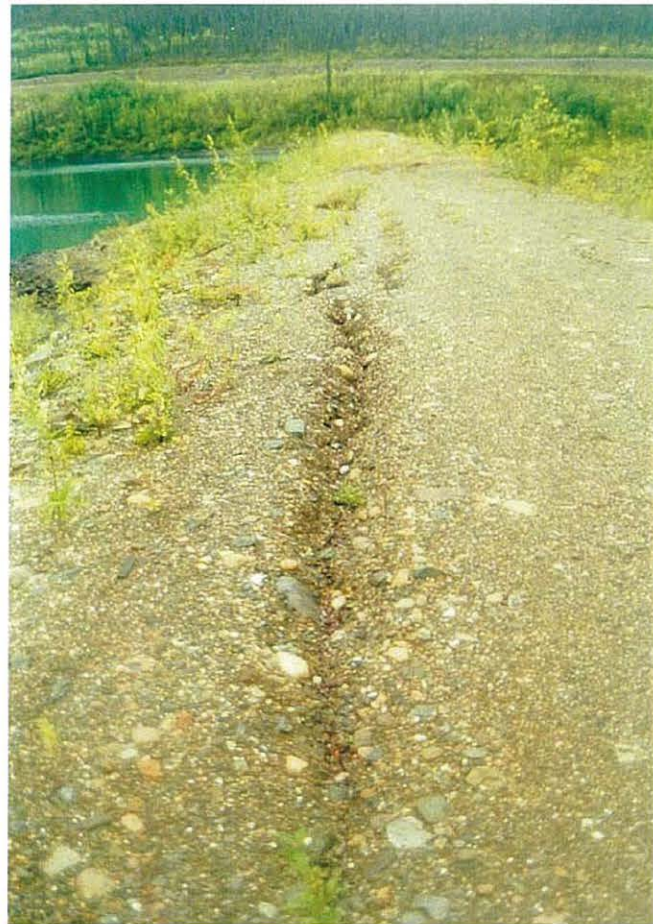
View of settlement trough in crest of Cross Valley Dam.
