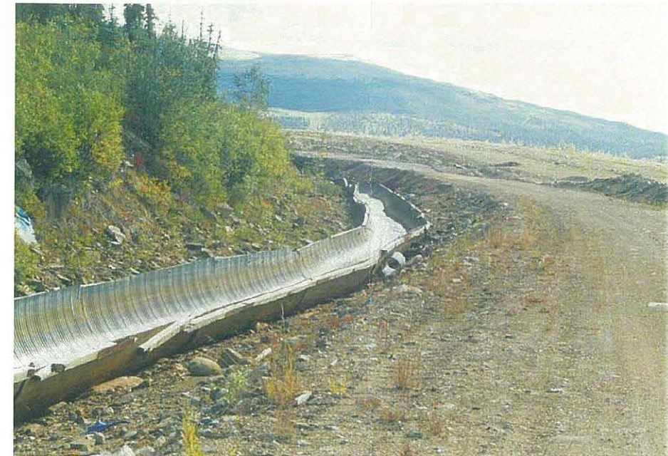
View of the Faro Creek Diversion Channel. Note the state of the half culvert channel liner.
