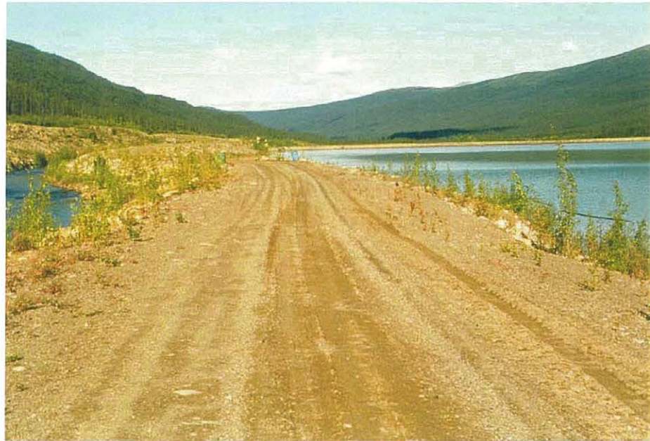
Area of settlement on the crest of the canal dike approximately 50 m west of CD-20. Magnitude of settlement estimated at 0.4m to 0.5 m.
