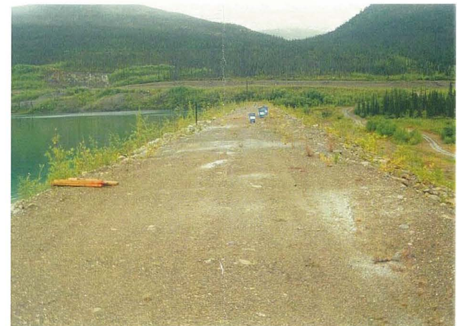
View of crest of Cross Valley Dam looking towards the south abutment.
