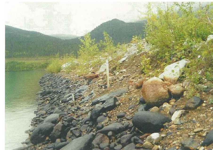
View of the exposed portion of the upstream face of the Cross Valley Dam.
