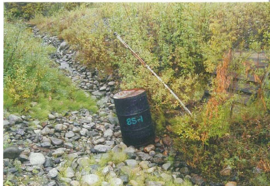
View of seepage collection trench at installation 85-1. Note seepage in trench.
