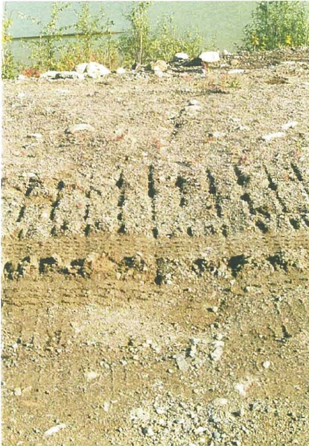
Above: Transverse crack in crest of canal dike near installation CD-21.
