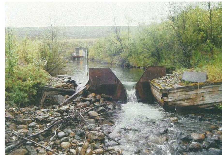
View of seepage weir in channel downstream of valve house. Note seepage flowing around side of weir.
