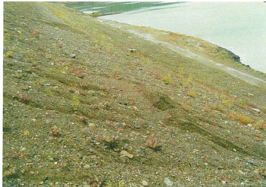
View of a bulge on the face of the Intermediate Dam.
