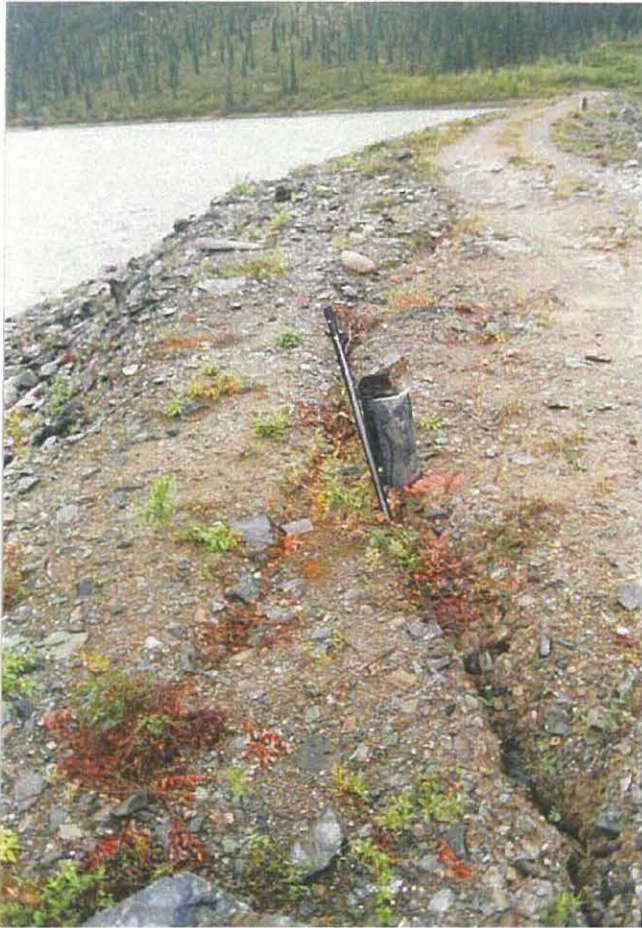
Left: View of the cracking on the crest of the FWSD. Approximate location is near installation 85-5.
