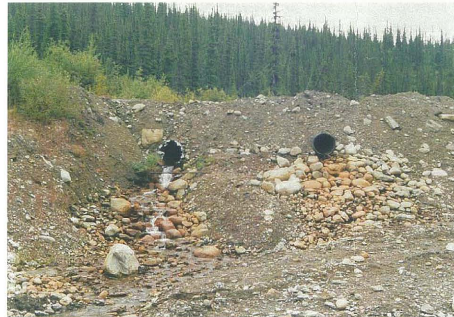
View of the downstream end of the two culverts which run under the main access road and drain into the outfall section of the North Valley Interceptor Ditch.
