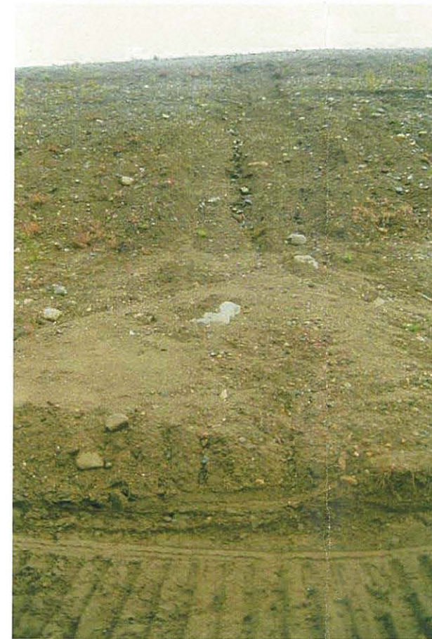
Debris cone at the base of an erosional rill located on the downstream face of the Intermediate Dam.
