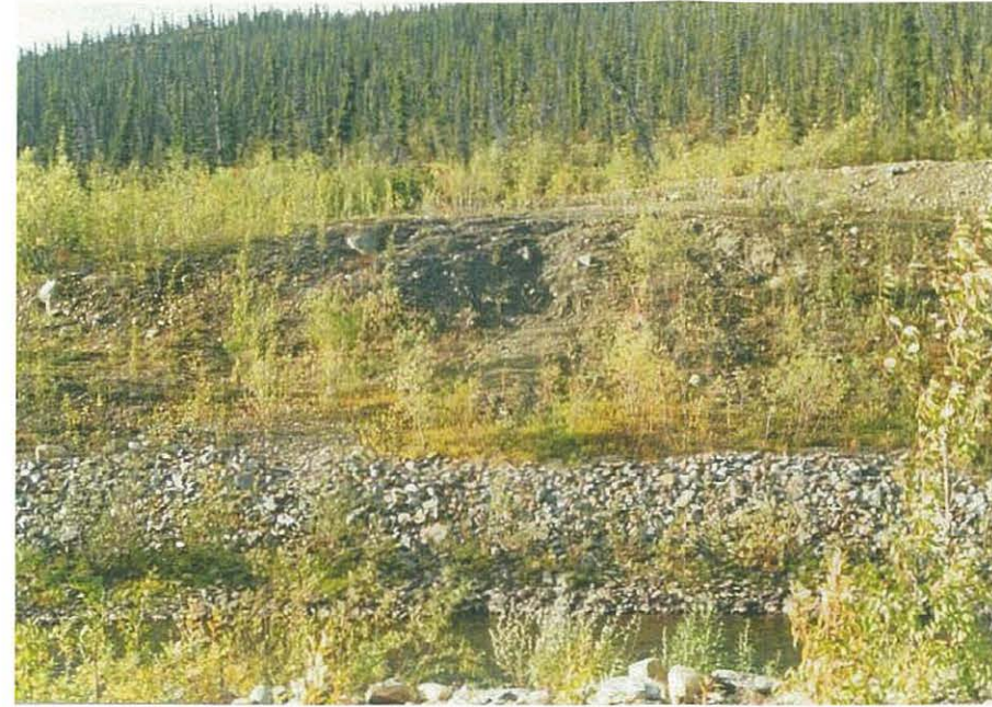
View of the face of the back slope of the canal dike. Note the surficial erosion of the face. Location is proximal to the old slide area at 2+000.
