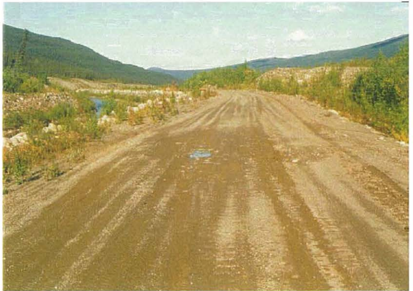
Below: A slight pot hole depression and some standing water situated approximately 50 m west of CD-13.
