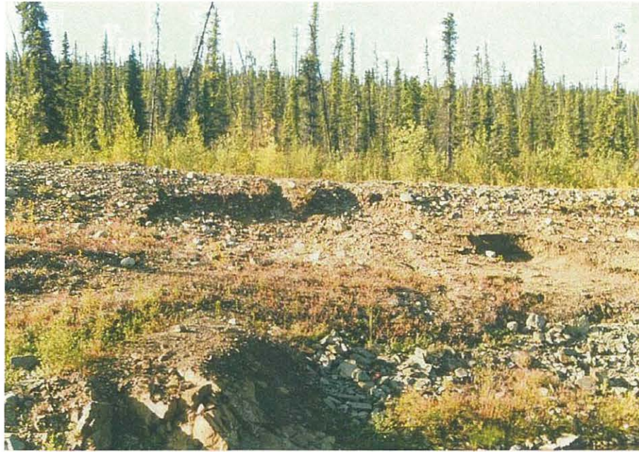
Frontal view of failure in canal dike back slope. Located at the entrance to the diversion canal.
