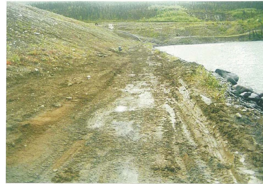
View of standing water and wet softened area at the toe of the Intermediate Dam.
