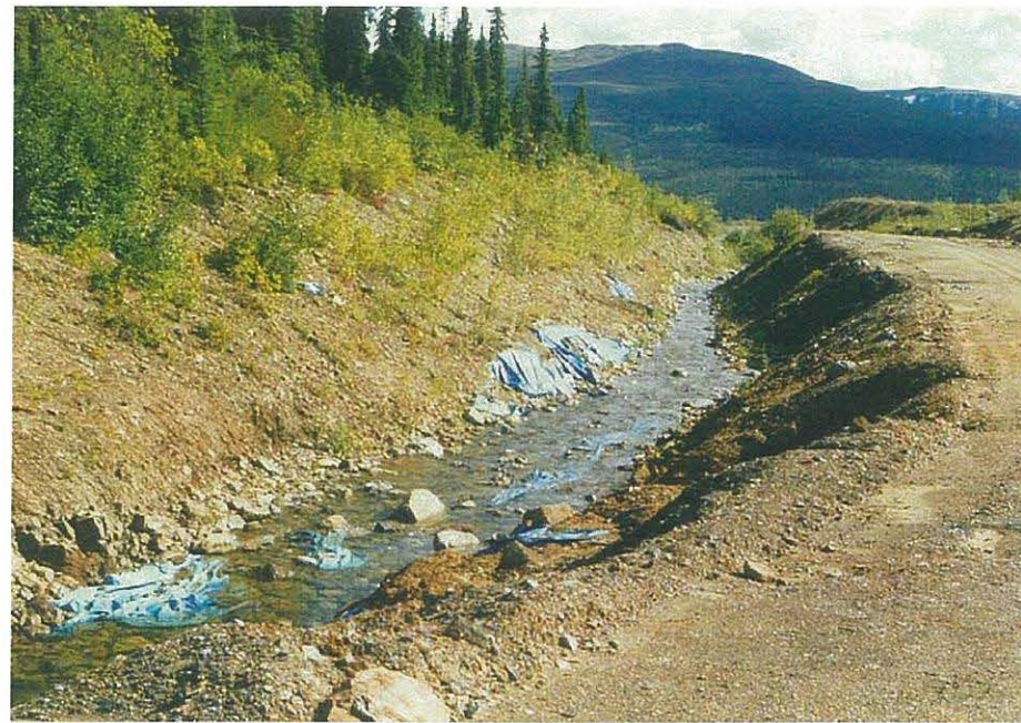
View of the Faro Creek Diversion Channel above the Faro Pit. Note the poor state of the blue channel liner.
