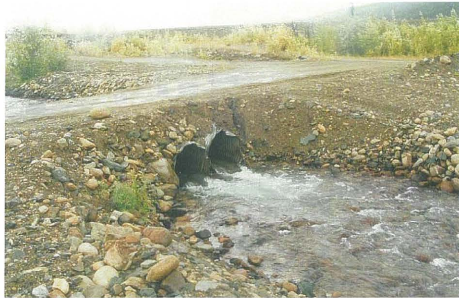
View of outlet side of culverts used to pass water beneath the access road to the Cross Valley Dam which crosses the channel. Note the disturbance to the protective rip rap.
