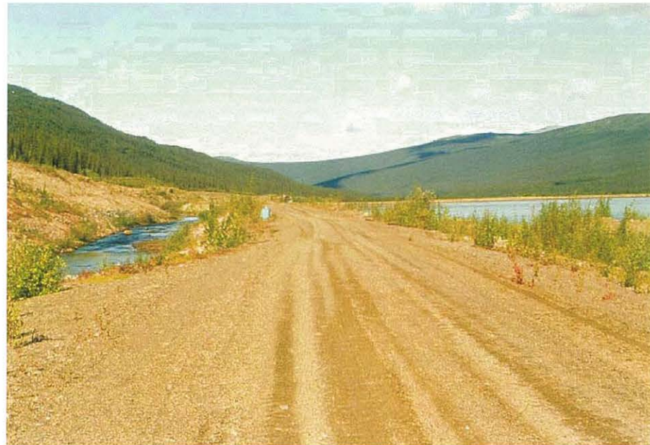
Crest of canal dike looking west as seen from installation CD-18. Note the undulations in the crest.
