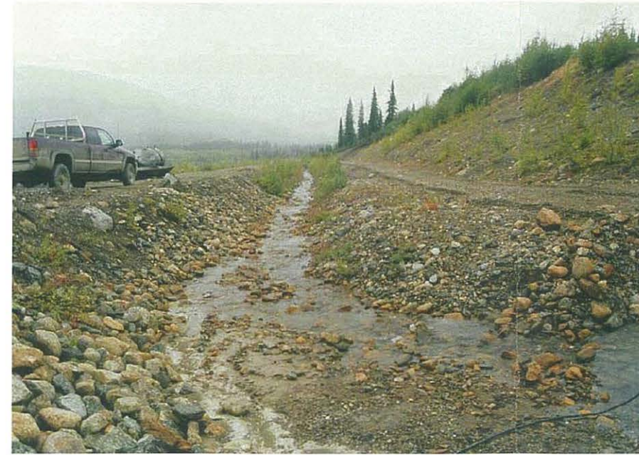
View looking downstream at the channel outflow section adjacent to the Cross Valley Dam. Note the apparent equal elevation of the top of the road on the left and right side of the channel.
