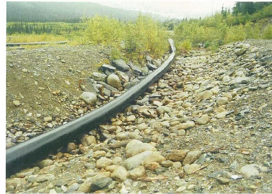
View of the pilot channel adjacent to the Cross Valley Dam Spillway.
