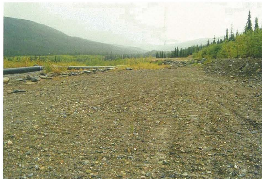
View of the bottom of the emergency spillway of the Cross Valley Dam.
