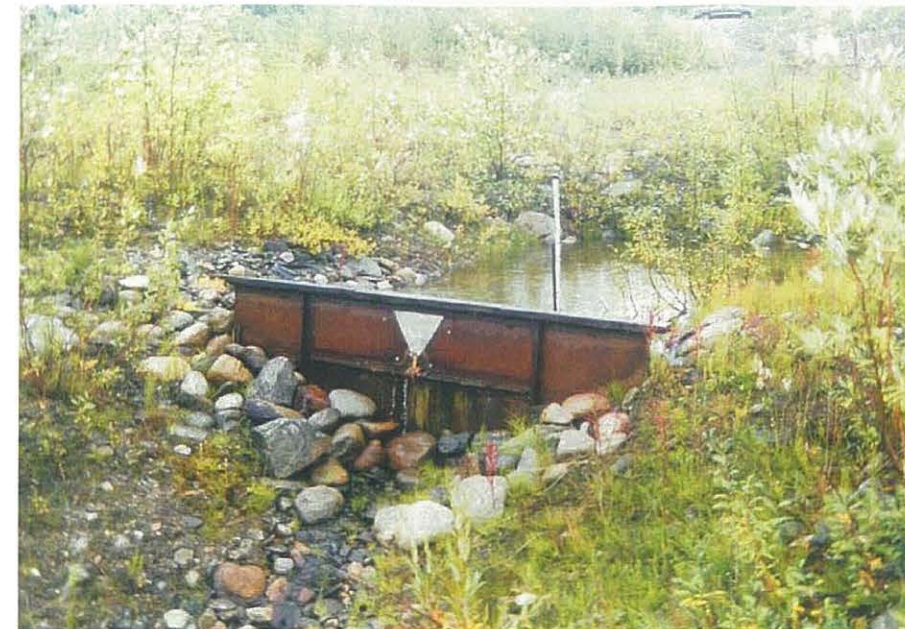
A seepage weir situated near the north limit of the collection trench.
