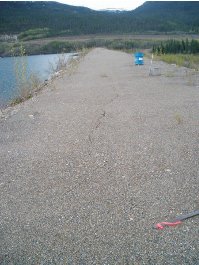
May: Photo shows a crack located on the upstream side.
