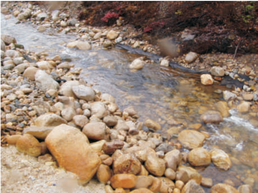
September: Photo shows an exposure of geotextile located under the riprap. This exposure is located several hundred metres before the bend in the Diversion Channel before it heads towards the east.
