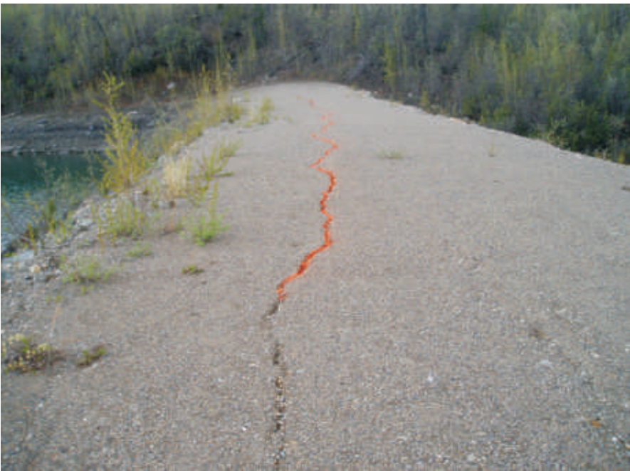
May: Photo shows an orange painted crack which progresses all the way to the south abutment of this dam. Water infiltration is leading to subsidence directly proximal to the crack.
