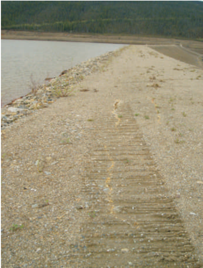
May: Photo shows some longitudinal cracks on the crest. These cracks progress further into the background of the photo as well along the crest. This is in the area where historically cracking has always been seen.
