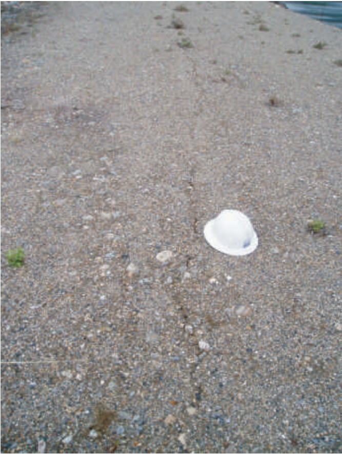
May: Photo shows some thin cracking located in the centre of the crest just immediately to the left of the hard hat.
