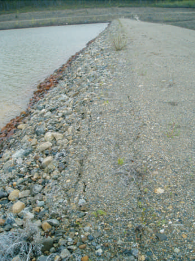
May: Photo shows some minor crest edge cracking on the upstream side, proximal to the riprap.
