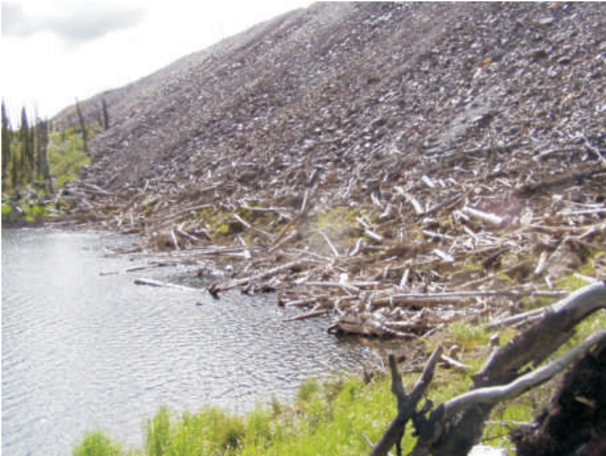
August: Photo looking along the upstream toe of the Rock Drain. Note the woody debris and grass growing on the face of the drain.
