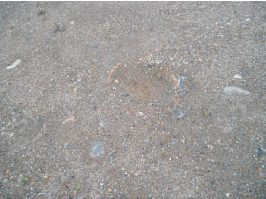
May: Photo shows one small sinkhole approximately 40 cm in diameter located on the crest. This sinkhole was marked last year. It does not appear to be getting much larger.
