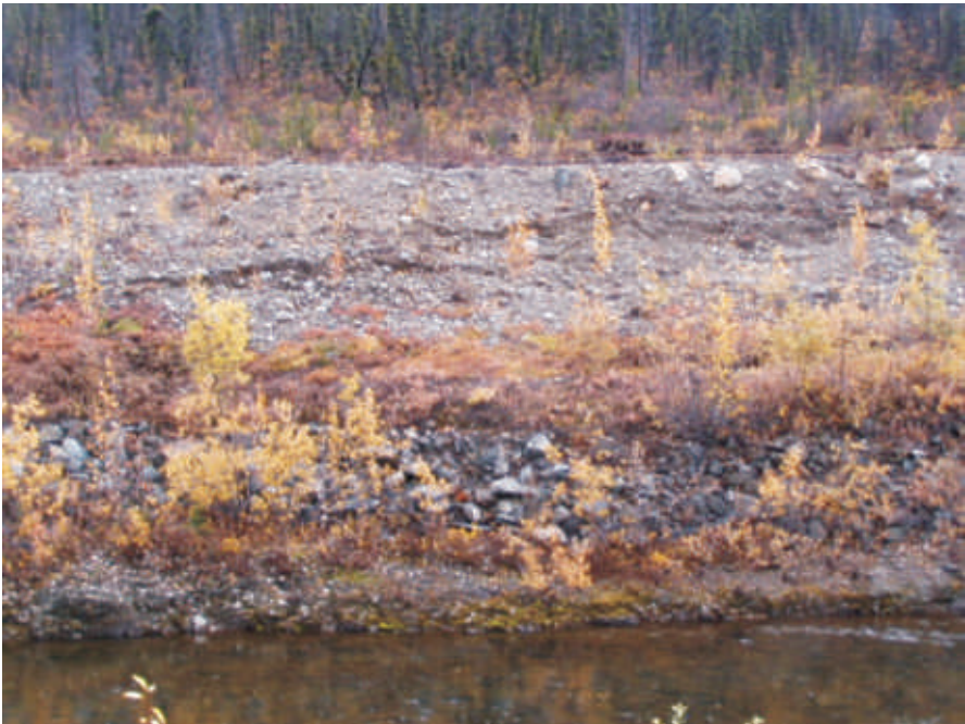
Photo shows some minor sloughing and a small scarp which is located on the backslope.
