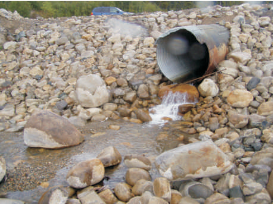
August: Photo shows a view of the outlet end of the culvert as the water cascades on top of the first rock. The large boulders which formed a break to water flow should be placed back into position.
