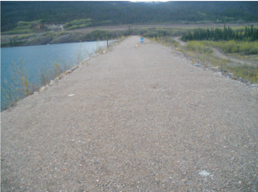
May: Photo shows the crest looking towards the south abutment. Within this area there is some minor cracking near the upstream side.
