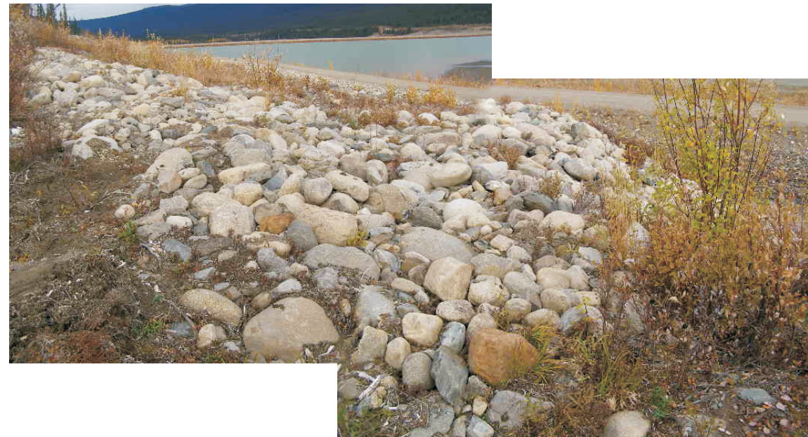
September: shows the placed riprap blanket which was placed on an old slough on the backslope.
