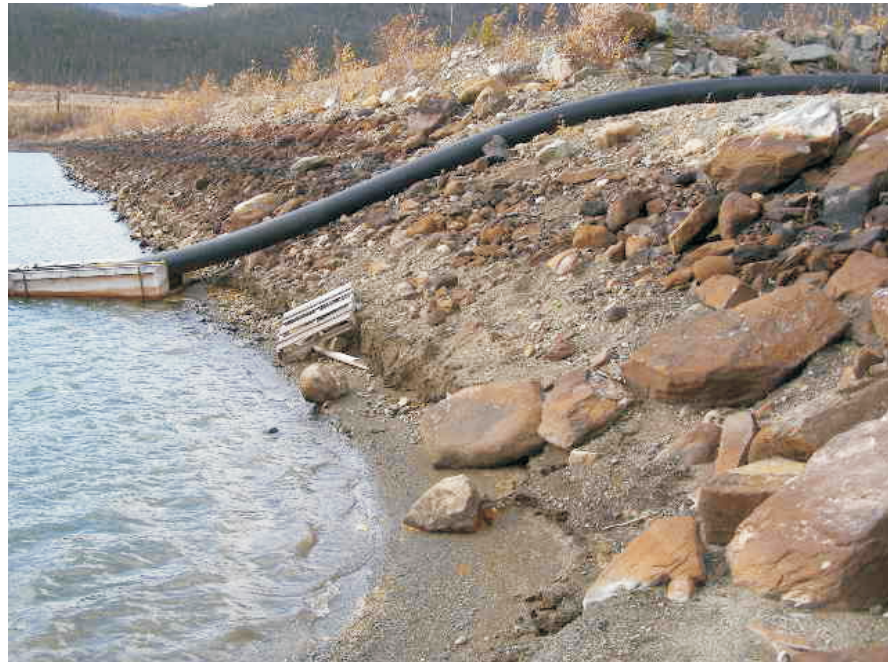
September: shows a view of the riprap on the upstream side. A small scarp which has formed at the pond level due to the lack of riprap.
