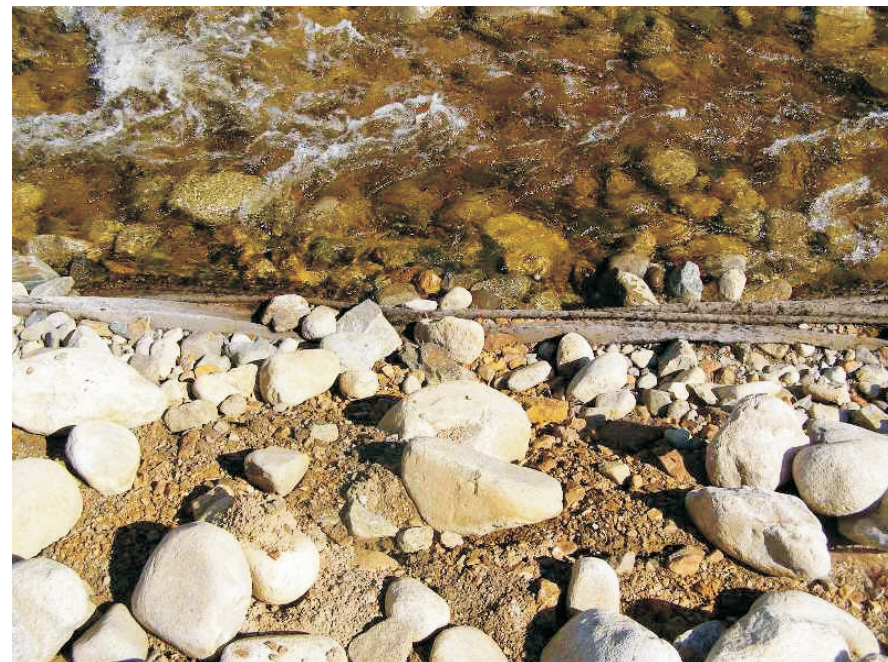
June: Note the exposed geotextile in the channel bottom. This was repaired prior to the August inspection.
