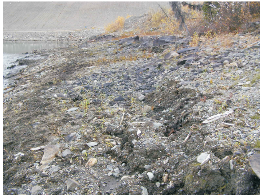
September: headscarp in seepage area on the southern limit of the Polishing Pond.
