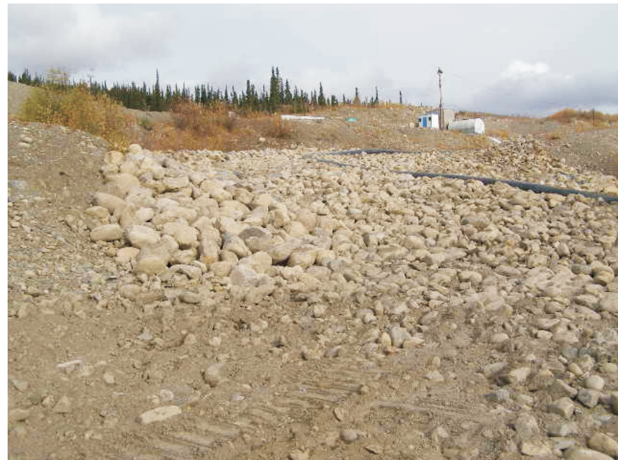
September: looking upstream in the spillway at the recent completed regrading of the riprap.
