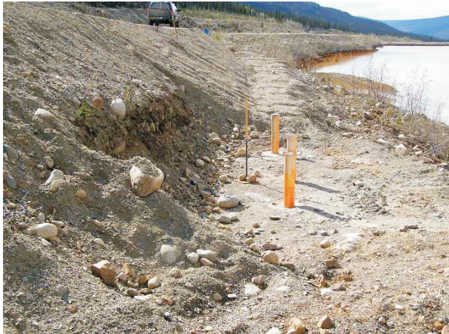
June: A view of three instruments installed in 2005. The oversteepened slope in this area should be backfilled to buttress the slope.
