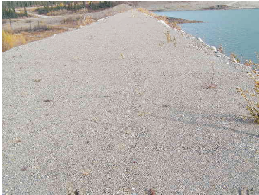
September: shows a very subtle manifestation of some previously existing cracks in the crest. The outline of a small trace of a settlement trough can be seen in this photo.
