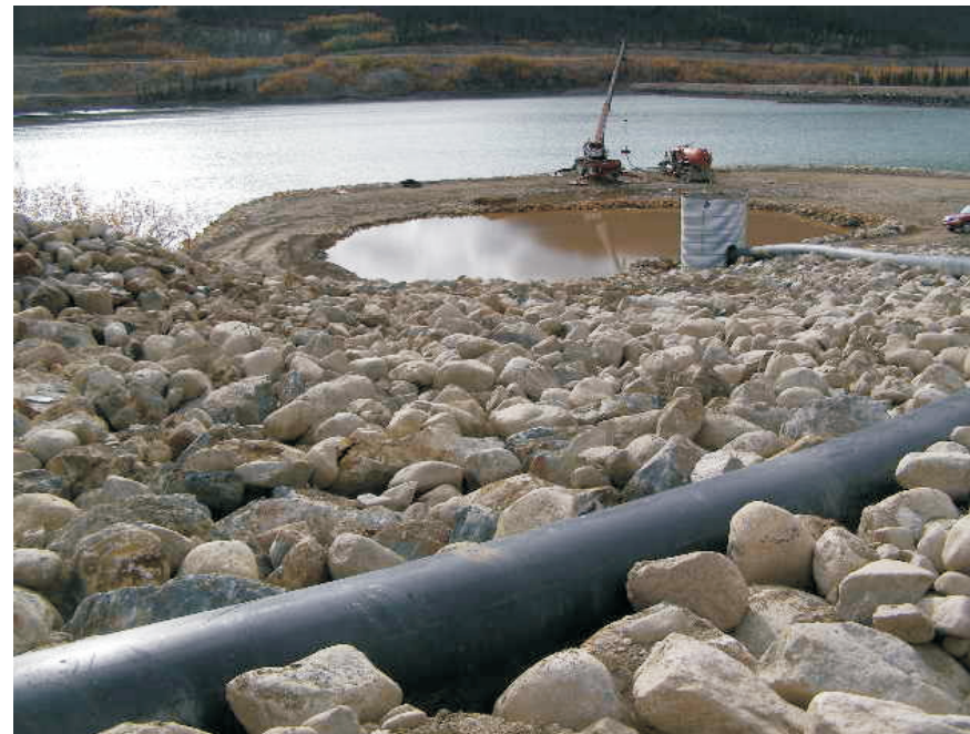
September: overlooking the sludge collection area. Looking at the riprap apron that was repaired by removing the riffle/pool arrangement between August and September 2007.
