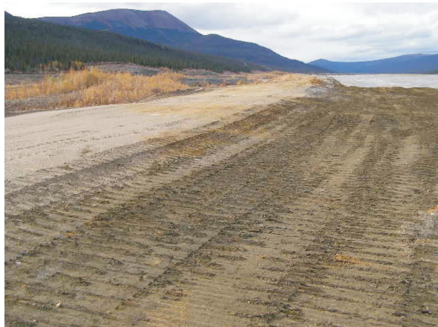
September: shows the re-graded crest on the Secondary Impoundment Dike where, it connects to the road coming from the Diversion Dam. The ditch line that was in here has now been backfilled over with sand and gravel.
