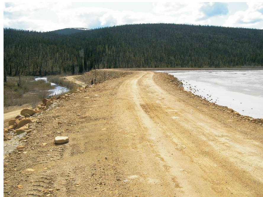
June: shows a view of the crest of the dike the Secondary Tailings Dam looking towards the south. This shows the location where the North Fork Rose Creek Diversion flows near the toe of the dam.
