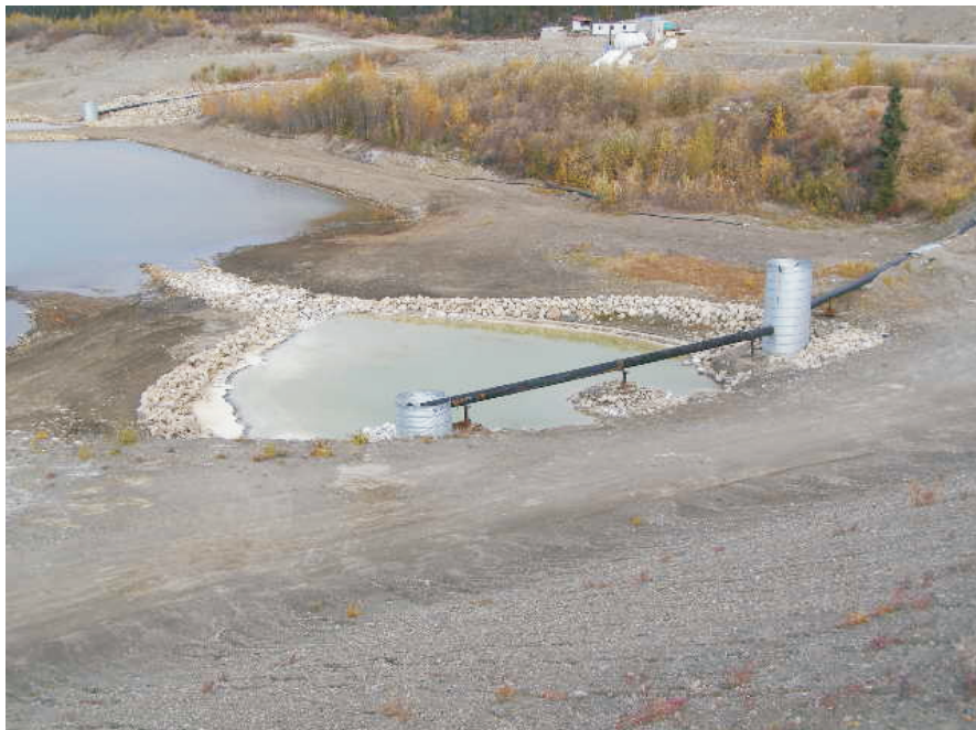
September: shows the sump arrangement located at the toe of the north abutment of the Intermediate Dam.
