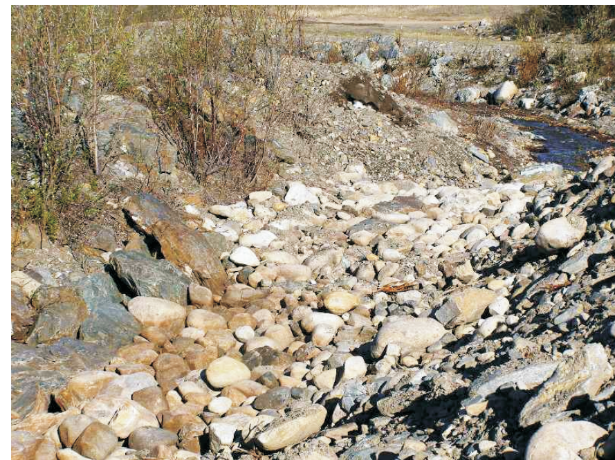
June: View of riprap in the decant of the Cross Valley Dam spillway.
