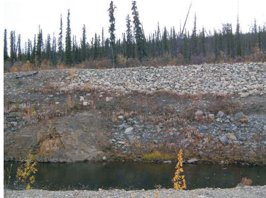
September: view of the riprapped area shown from the crest of the backslope in the bottom right photograph on Figure 7.
