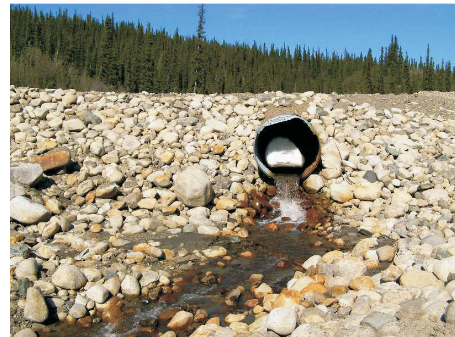
June: Culvert outlet, note the ice partly plugging the culvert.
