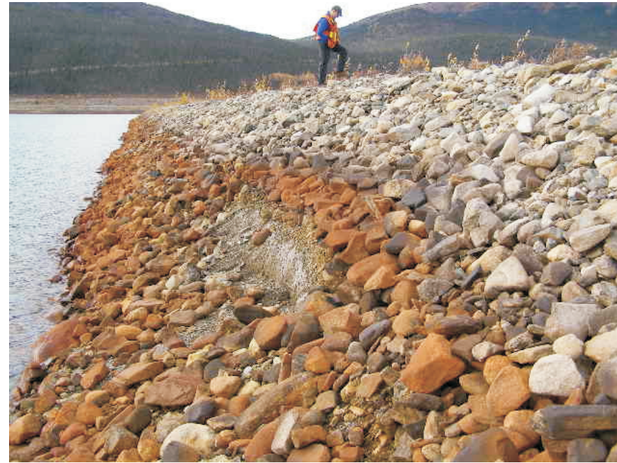
September: shows a small scarp formed on the riprap.
