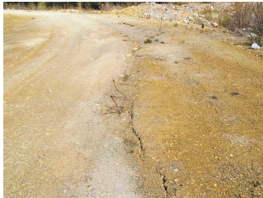
June: shows a view of a settlement trough crack along the edge of the lower road. This is near the entrance to the Diversion Canal.
