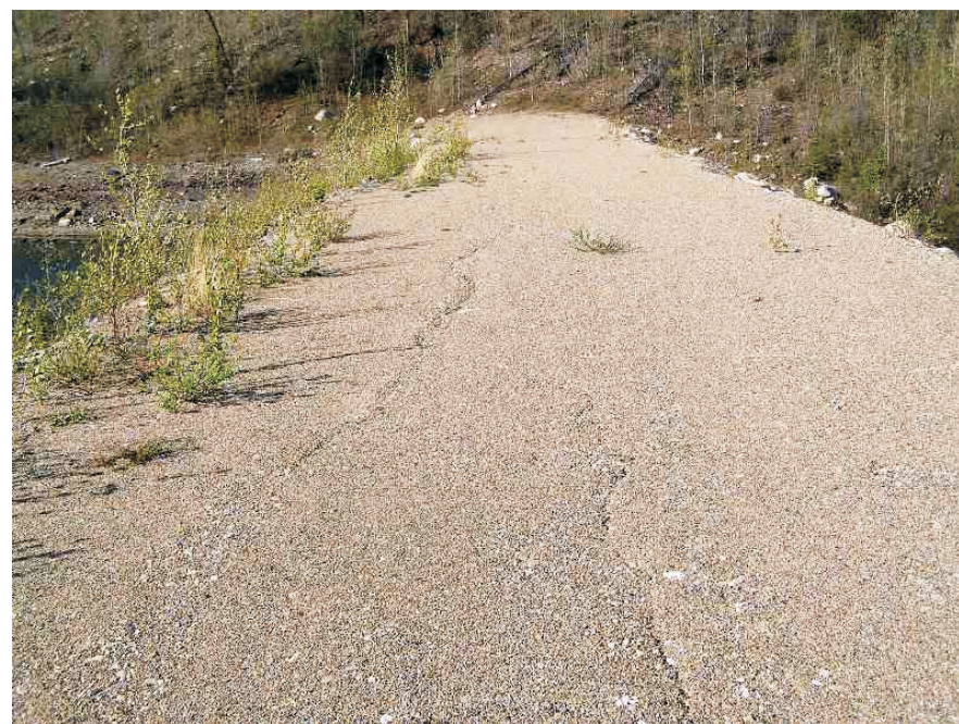
June: Nearing the south abutment, with a faint crack on the crest of the dam.
