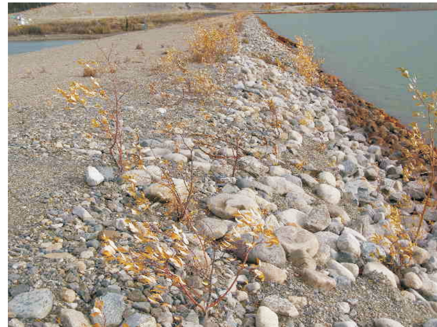
September: view of the upstream side of the crest. Vegetation which is catching on and should be removed.
