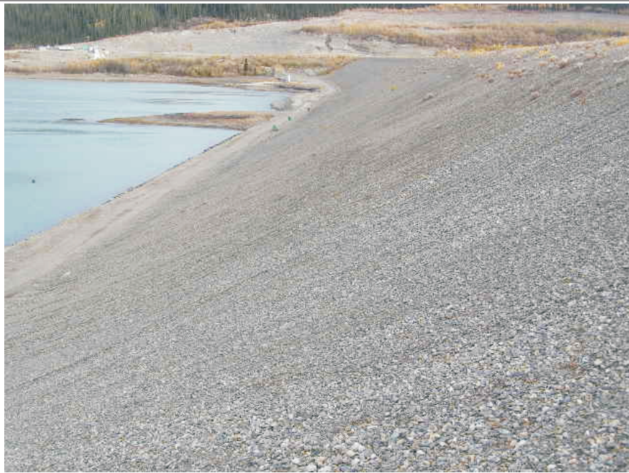
September: a view of the downstream side of the dam. The slope has a good, even, consistent grade with no signs of bulging, deformation or erosion. Minor amount of vegetation catching on upper portion of the slope.
