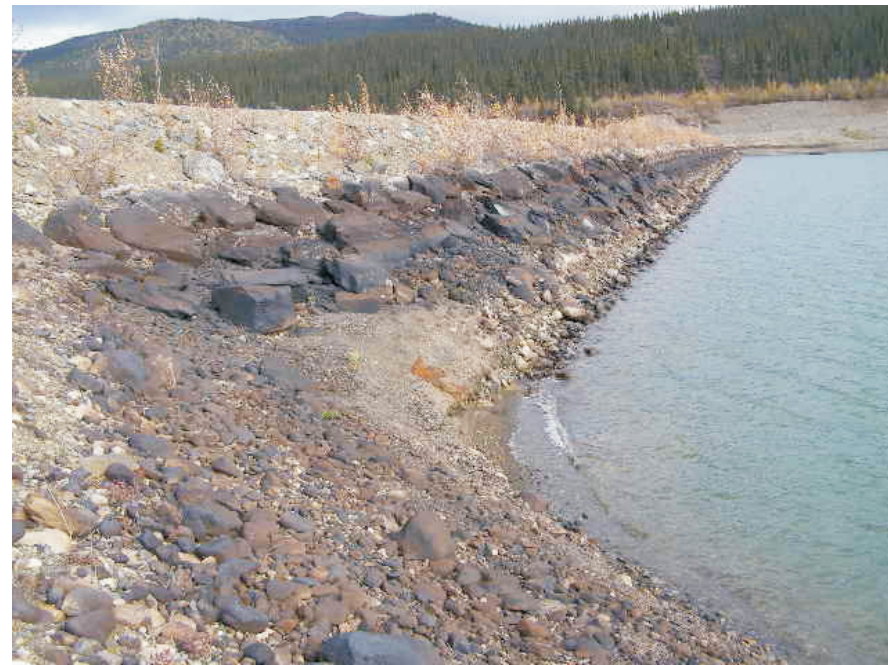
September: shows a view of the upstream side looking towards the north abutment. Some rather large riprap is evident in the mid section of the slope. In the foreground we can see some erosion at the lower pond level, where there is no riprap.
