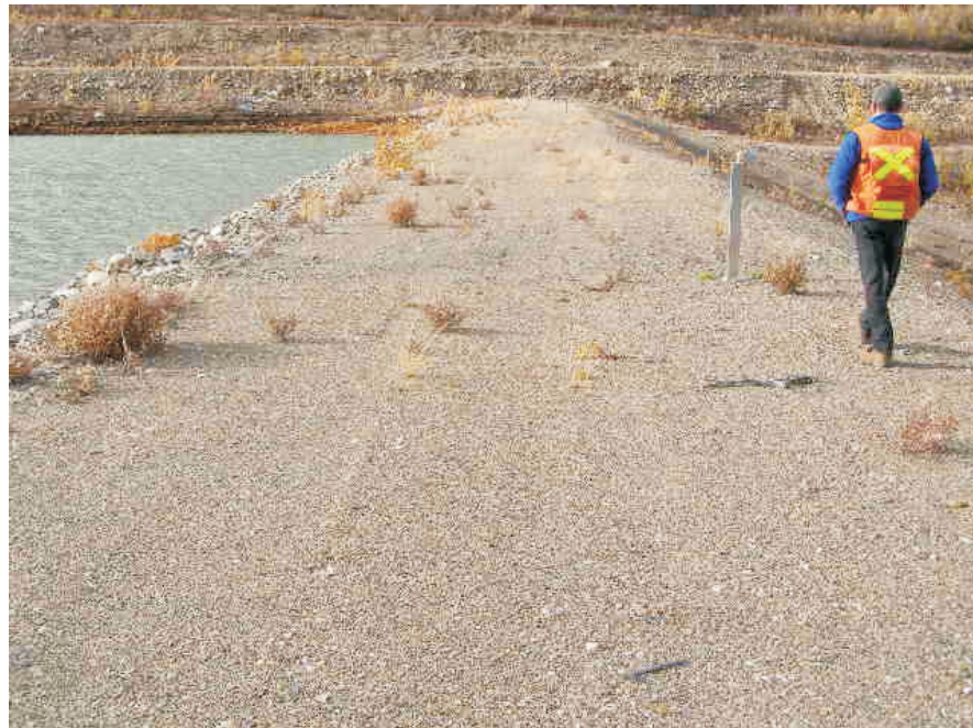
September: view of the crest looking towards the south abutment. No signs of settlement, cracking or deformation have been seen on the crest.
