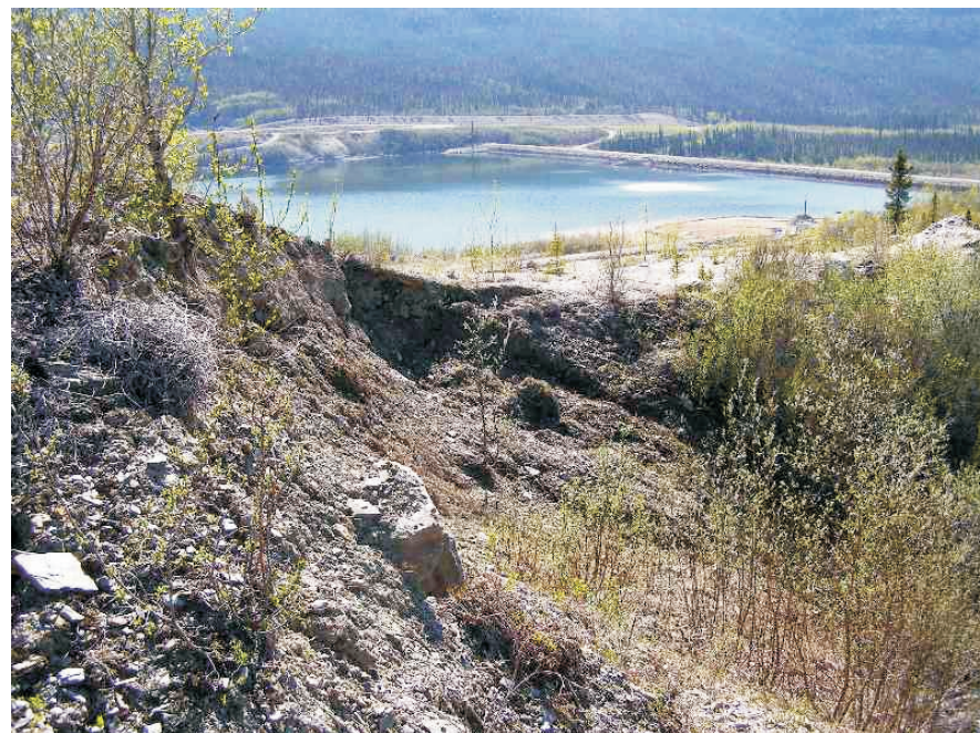
June: Sloughing of the berm near the steep section of the channel upslope from the Intermediate Dam.
