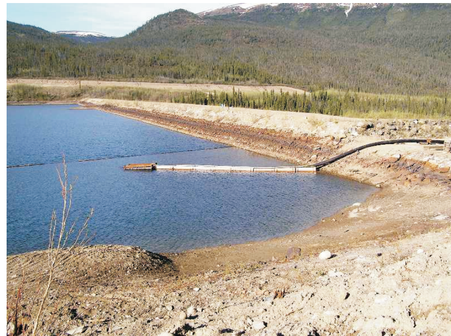
June: Siphon system in the spillway.
