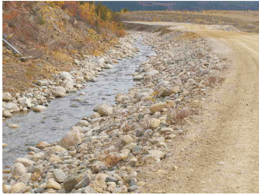
September: shows the continuation of the previously constructed Pilot Channel with the Faro Creek Diversion. The channel appears to be in good condition, no signs of significant erosion or deformation.
