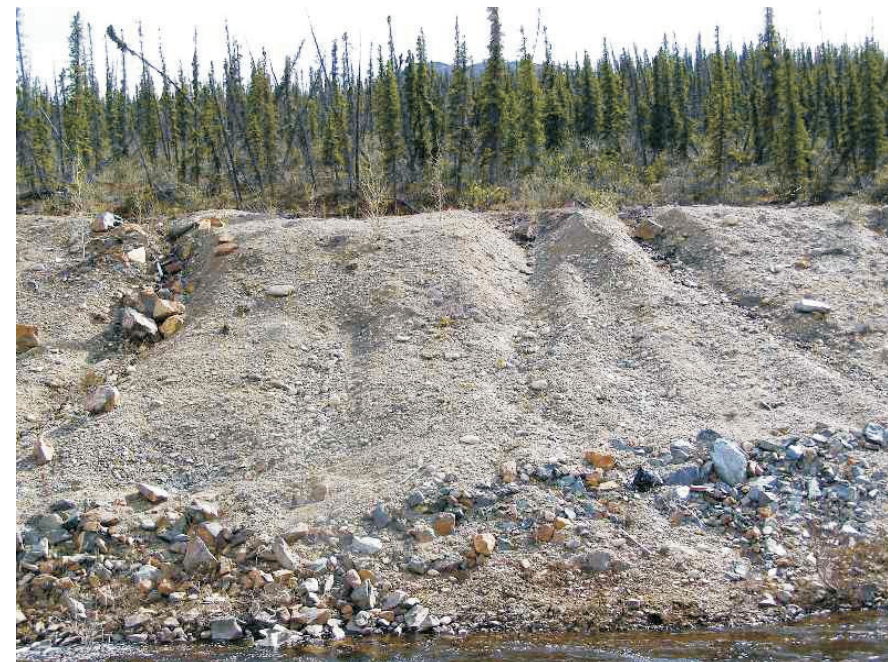
June: Shows the erosion gullies that have formed in the thermal protection berm above the boreholes drilled in 2005.
