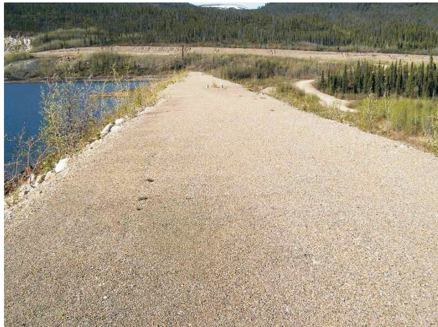
June: Note the faint evidence of past cracking on crest, near the northern quarter point.
