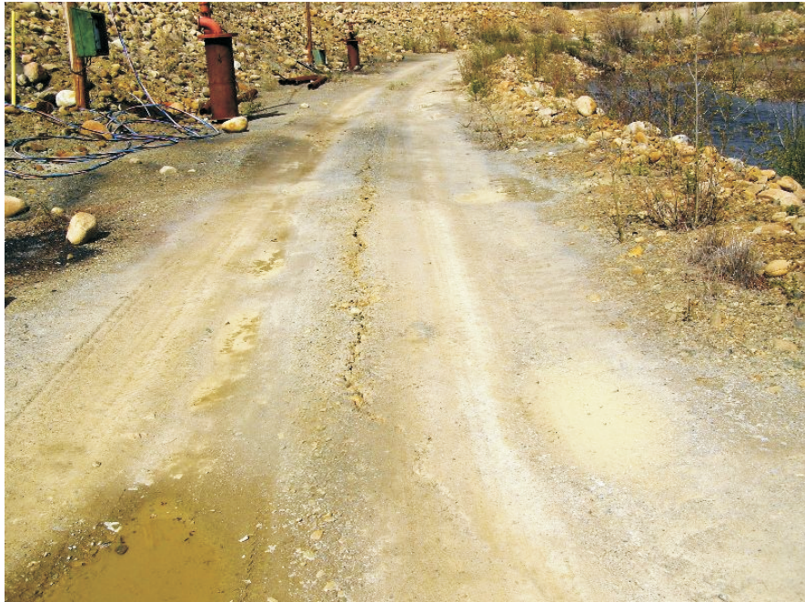
June: shows of the continuing view of the crack on the lower road of the Secondary Tailings Dam, just near the area of the pumping wells.
