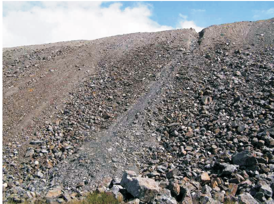
June: shows a view of the upper portion of the downstream face. Note the two areas with finer grained material covering coarser rock. This is due to erosion gullies coming off the haul road surface on the crest.
