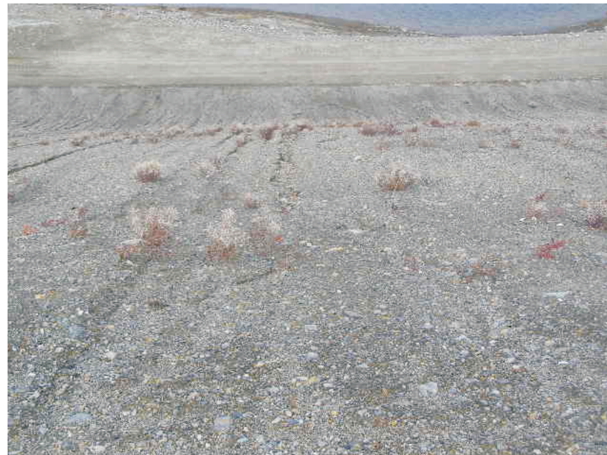
September: shows the minor erosional rills located on the downstream face.
