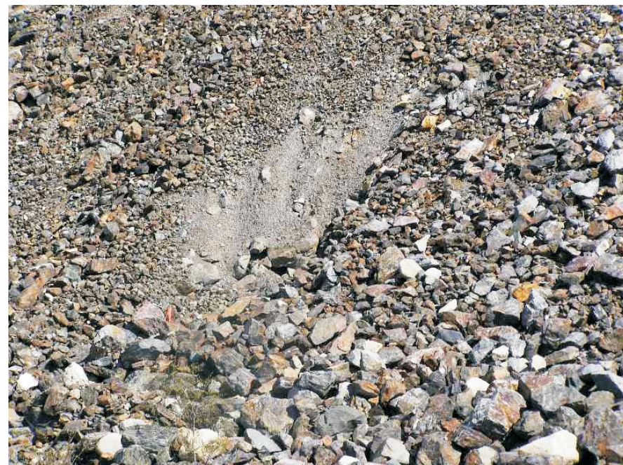
June: shows a close up view of the area noted last year as being eroded out. It is almost in the centre of the Rock Drain.
