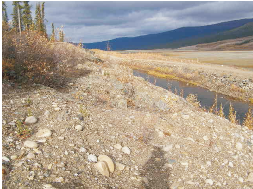
September: shows the erosional gullies and small instability which previously occurred on the backslope, just west of Goodall Creek.
