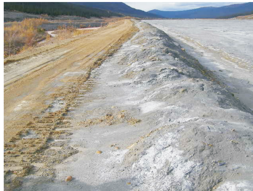
September: photo shows a view of the crest looking towards the west. At the current time there is no standing water on the upstream side.
