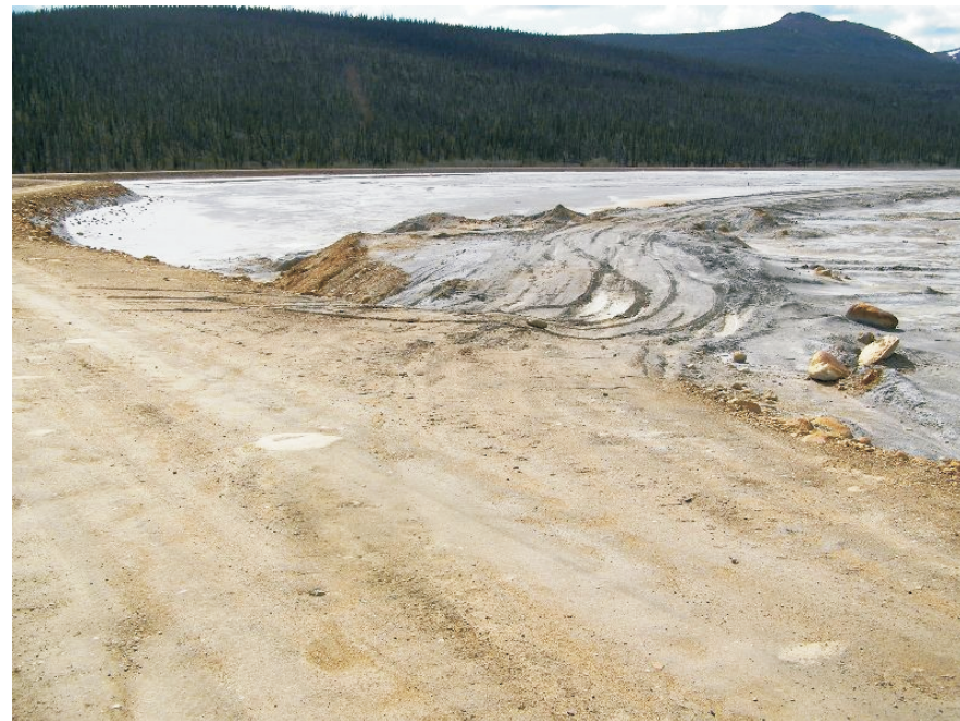
June: shows a view of the Original Tailings Impoundment inside the Secondary Tailings Dike.
