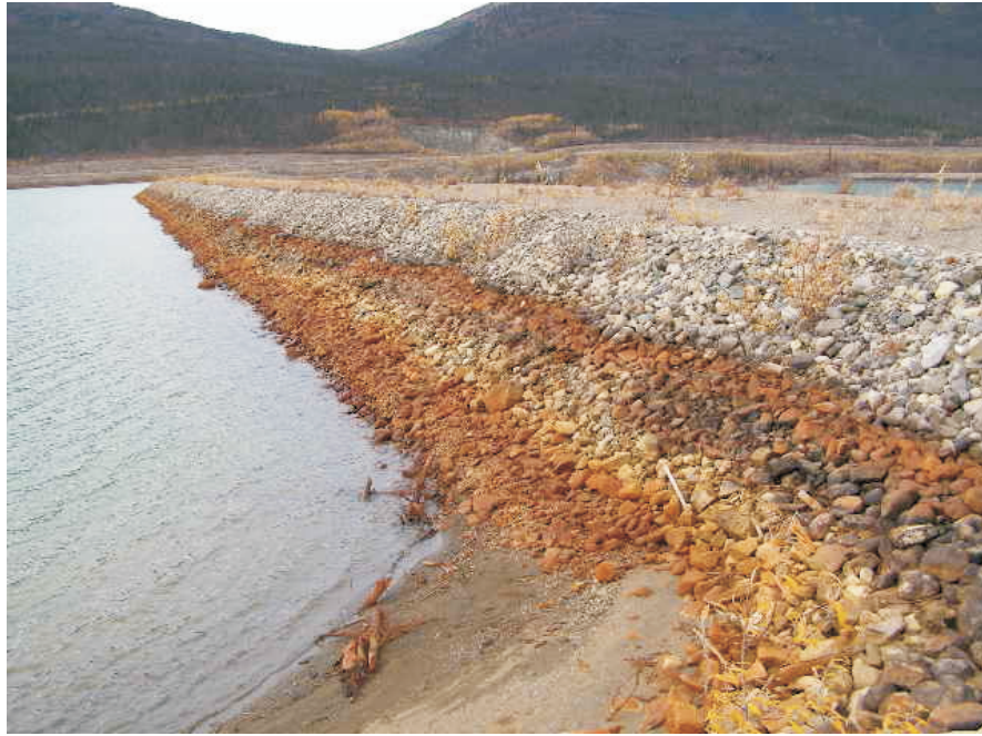
September: Shows the upstream side of the Intermediate Dam including the exposed riprap due to the low level of the pond.
