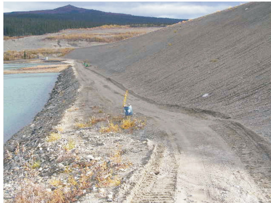
September: taken along the toe looking towards the north abutment. From this perspective, there are no signs of seepage discharge on the toe berm road.
