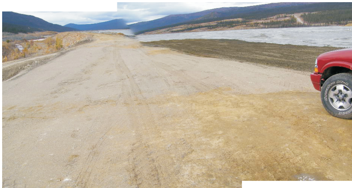
September: a two shot panoramic showing the repair which has been done to the small trench in the crest of the Secondary Impoundment Dike, (see first photo).
