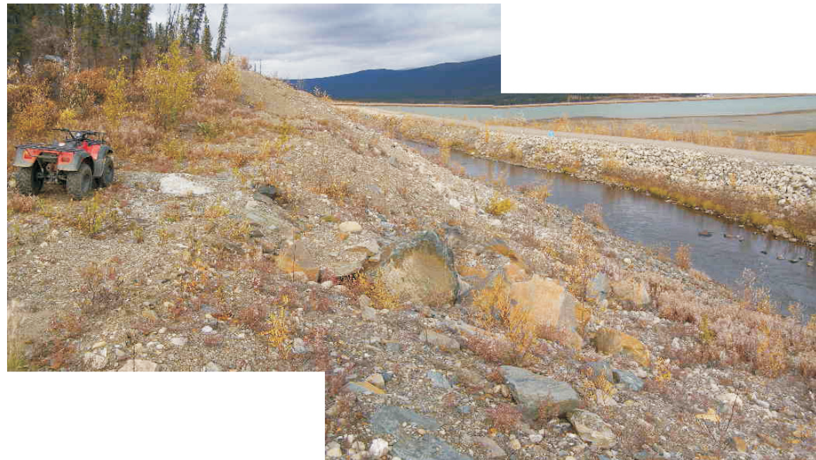
September: show a panoramic view of the thermal protection berm along with the large riprap which was previously placed within a erosional gully. At the bottom of the slope there is a significant amount of vegetation in the erosion gullies indicating water flow.
