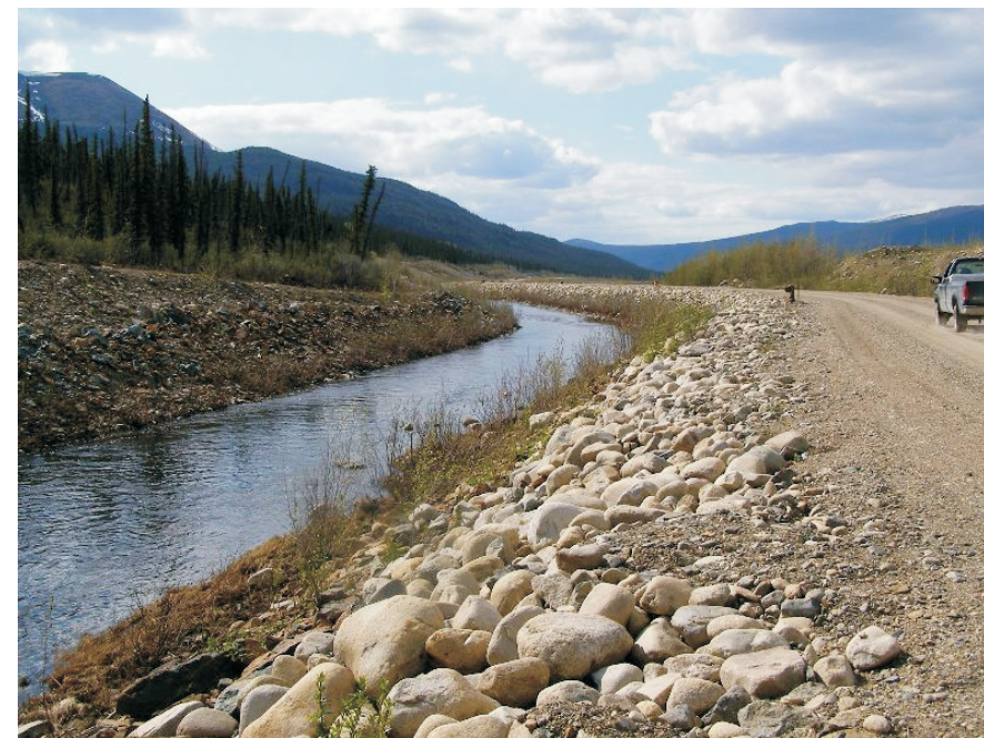
June: shows the first main corner in the portion of the RCDC that was upgraded in 2004.
