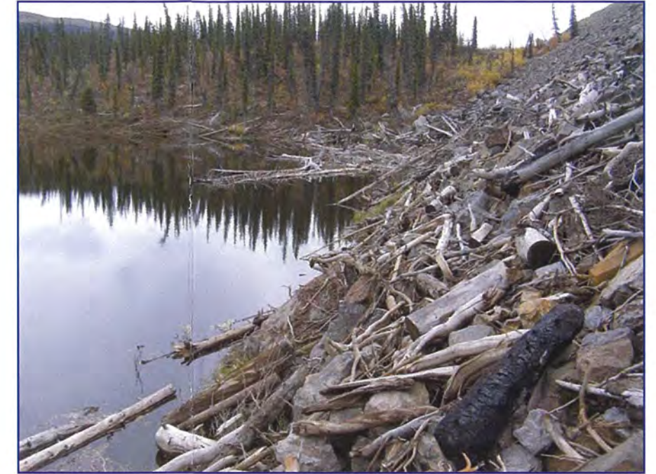
September: looking towards the east limit of the upstream pond. Note that the water level is approximately 3 m below the high water mark that is indicated by debris deposited on the face of the drain.
