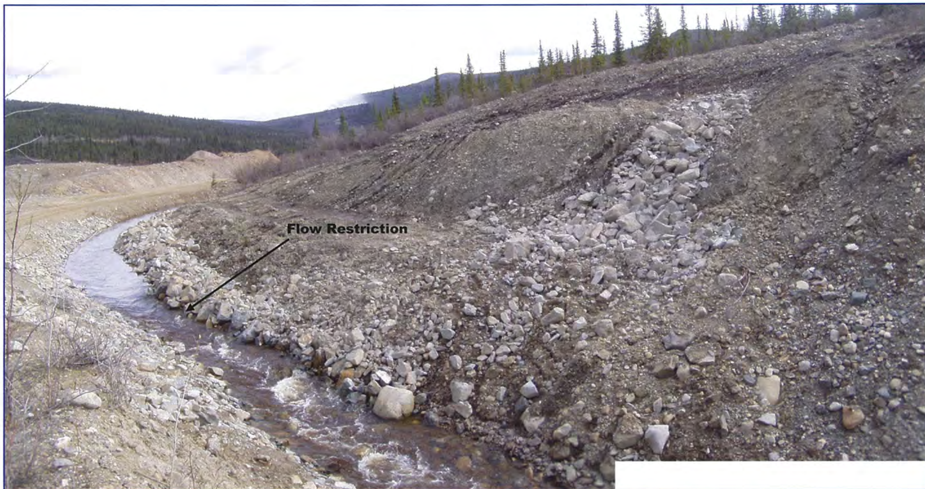
May: a panoramic view of the repaired slough area which was caused partially by over steepened banks. The area is still restricting the flow through the channel.
