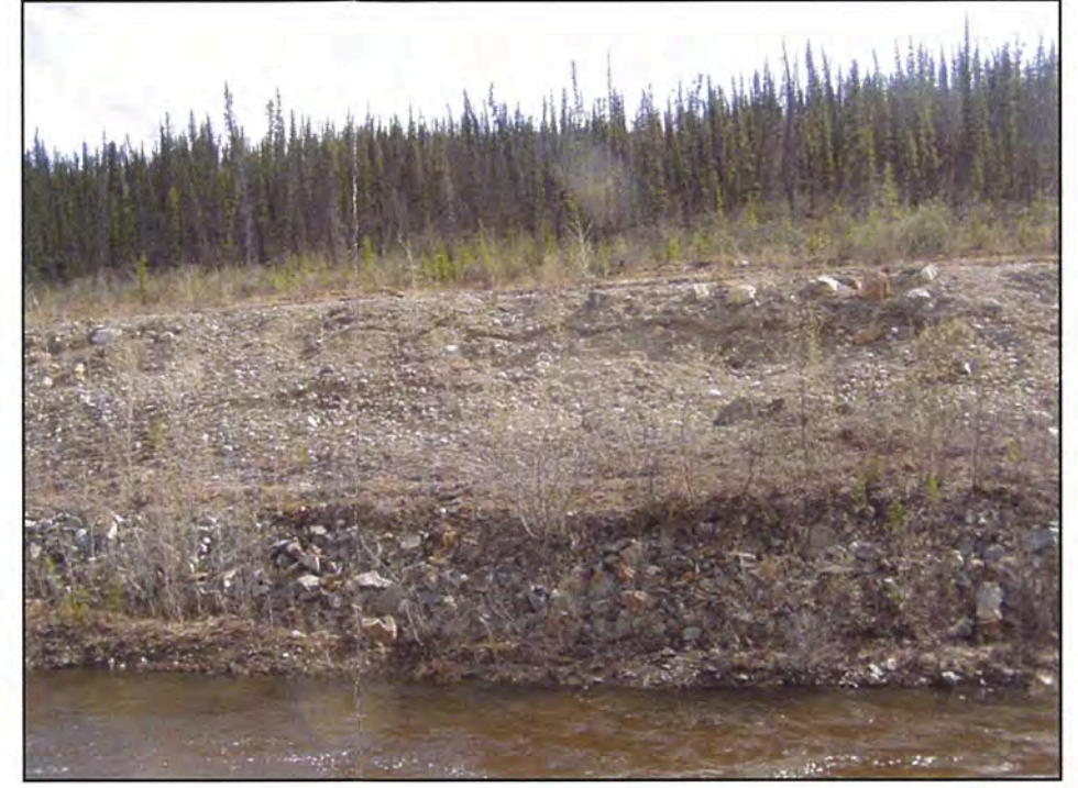
May: shows a view of the slump in the backslope of the Diversion Channel.
