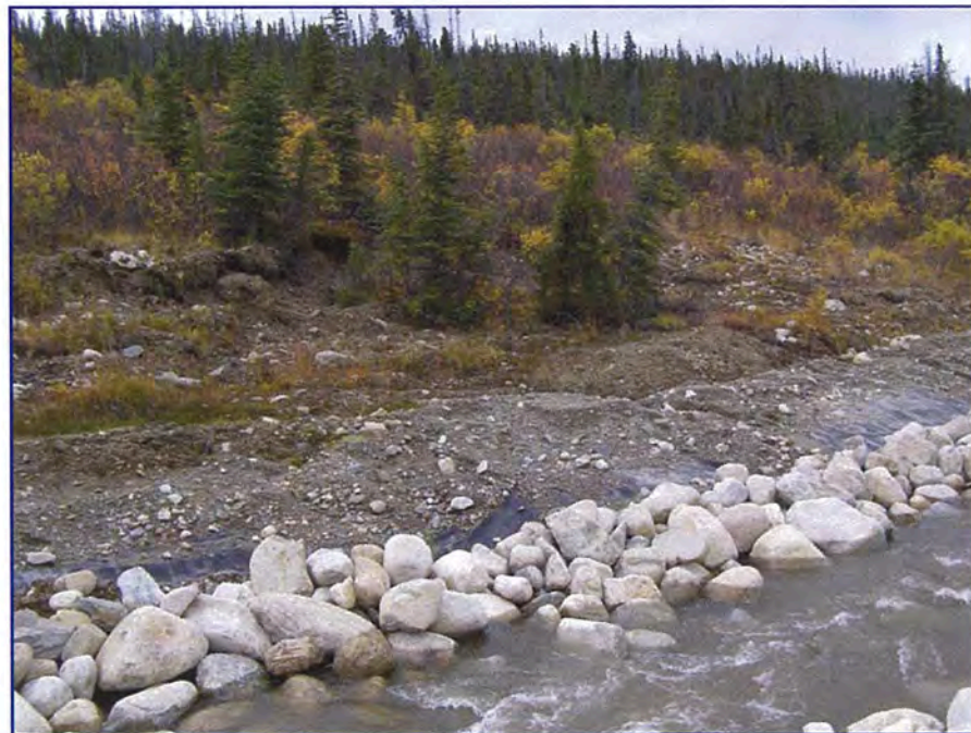
September: shows the backslope above the repair area. Note the slumping of the disturbed ground.
