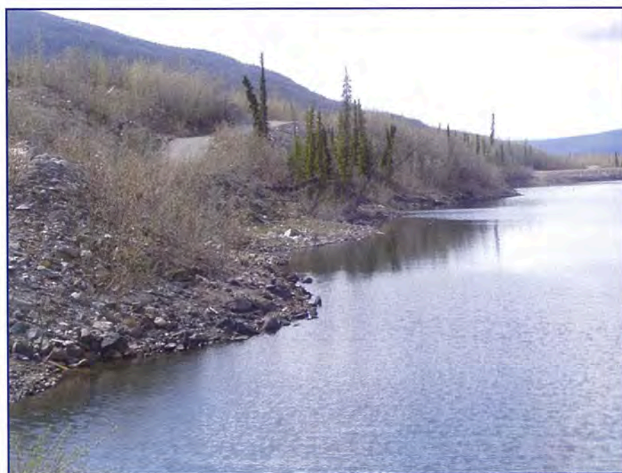
May: view of the polishing pond shoreline, which is formed by the spoil pile base. Note that this is an area of slumping and seepage.
