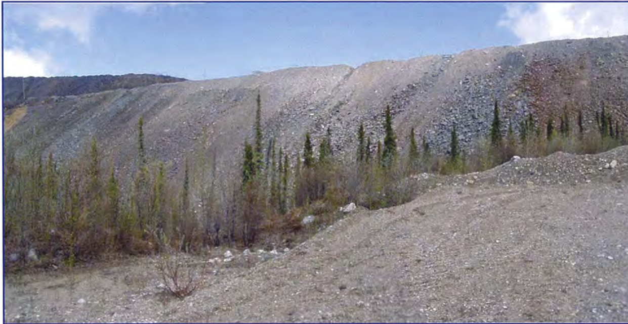
May: shows an overview of the downstream side of the North Fork Rock Drain. Note the erosion gully on the face.
