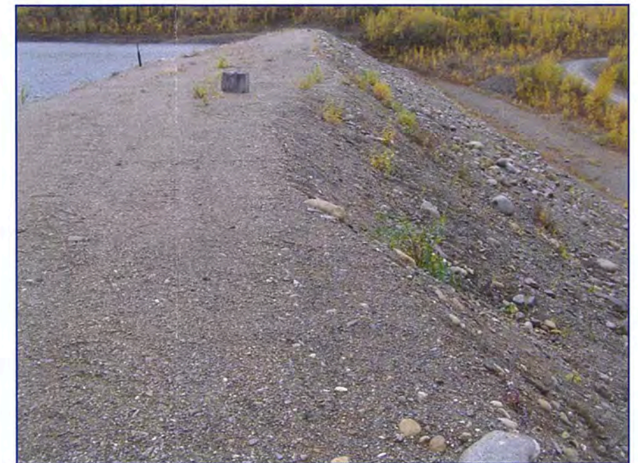
September: shows a view of the crest and downstream face with an area that needs to be filled in to re-establish the design crest width.
