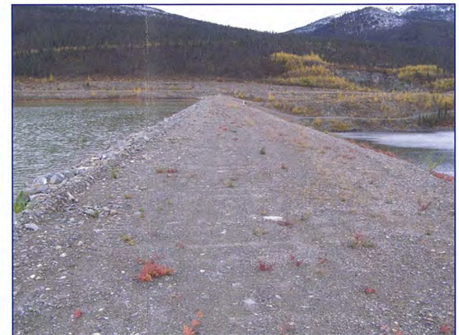
September: a view of the dam crest, note that there is a small amount of vegetation growing after removal in 2007.
