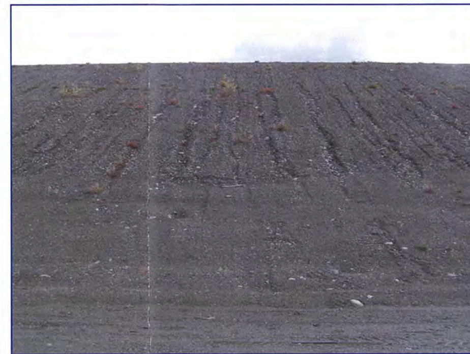
September: a view from the crest of the Intermediate Dam looking at the downstream face. Note the appearance of the erosion rills on the face.
