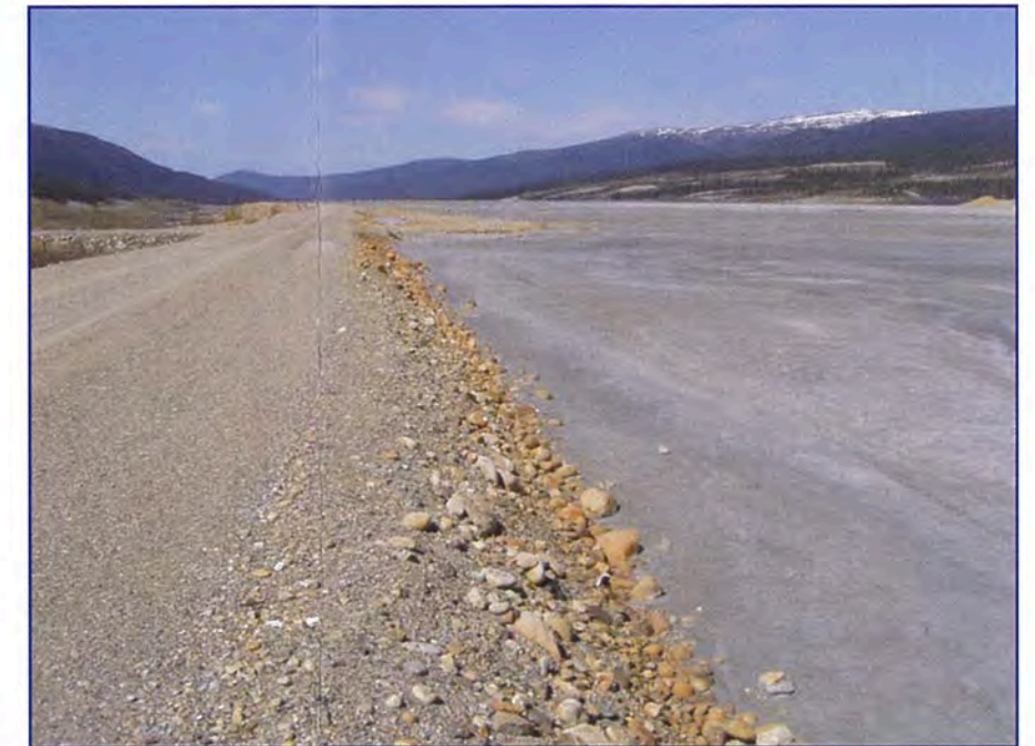
June: looking down the upstream face from the crest of the dam.
