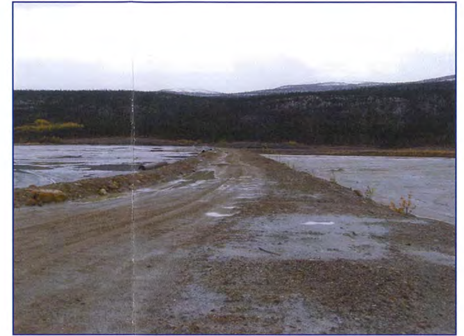
September: a view of the crest of the dam. Note that some settlement holes are forming and erosion is evident.
