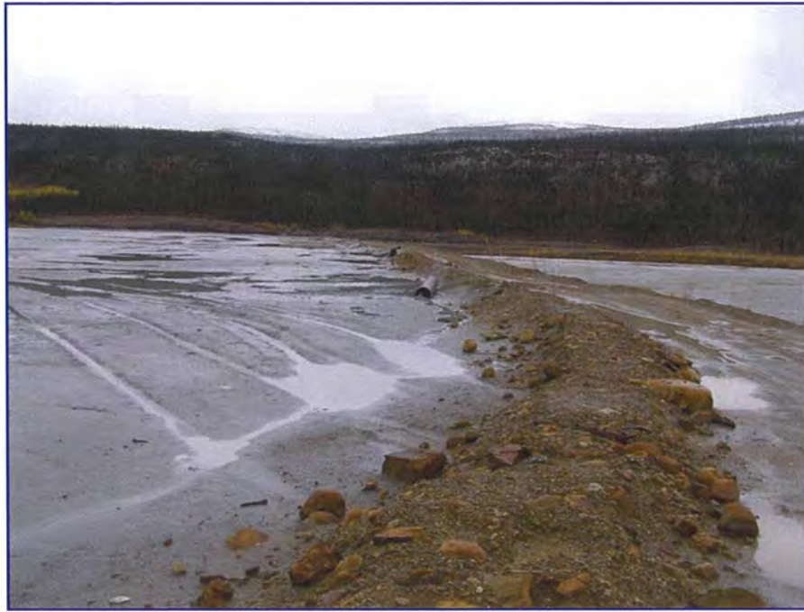
September: shows the upstream side of the Secondary Dam. Note the water ponded near the small berm on the upstream side of the crest.
