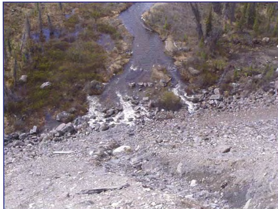
May: a view looking down from the crest at the discharge of the Rock Drain.
