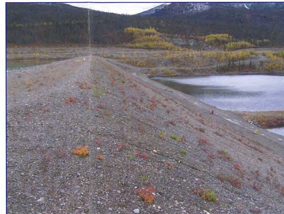
September: a view from the crest of the Intermediate dam looking at the downstream face.
