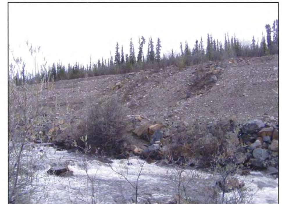
May: shows a view of some erosion gullies in the backslope of the canal.
