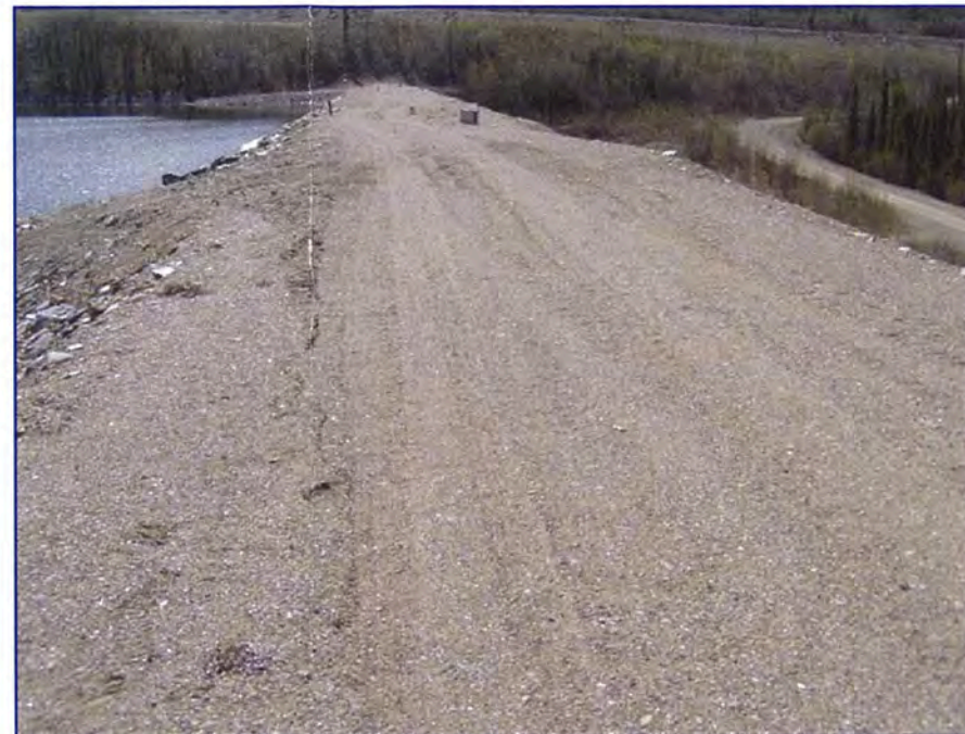
May: shows a view of the crest of the dam, with a faint crack in the road.
