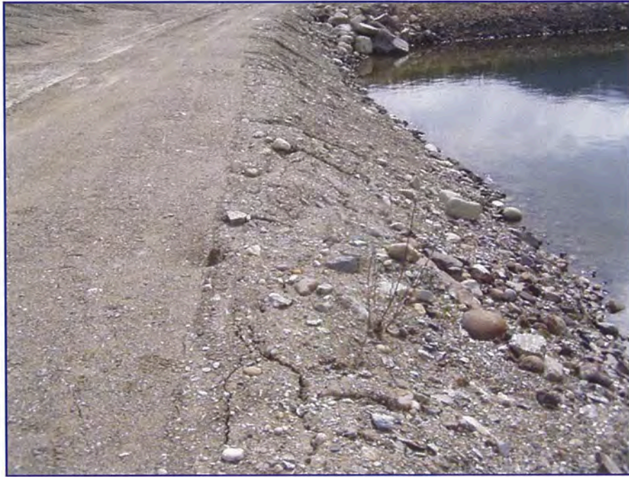
May: a view of minor cracking occurring at the edge of the polishing pond. Note that cracking has historically been seen in this area.
