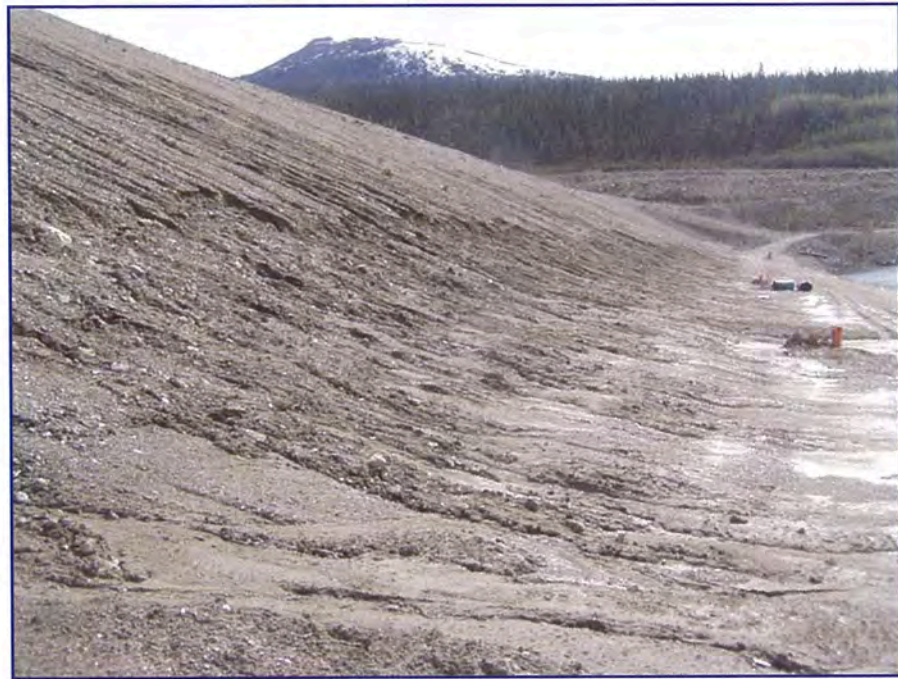
May: shows a view of erosion on the downstream face of the dam. This area should be repaired by removing the fines from the road surface.
