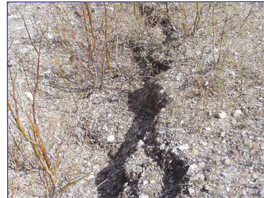
May: view of the headscrap formed by the slumping area, was noted in last year's inspection.
