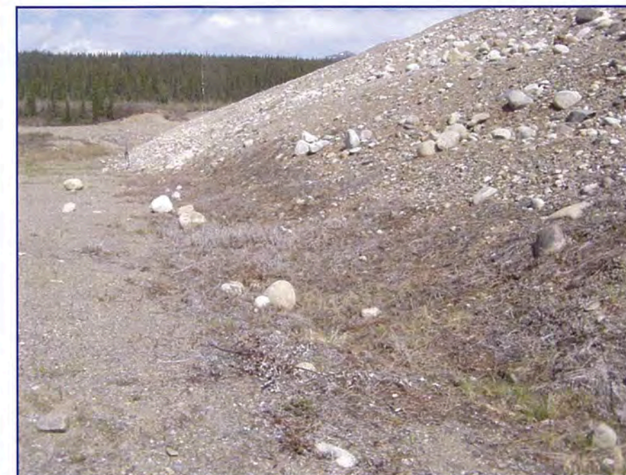
May: shows a view of the toe of the downstream side of the dam with some water loving plants present, which likely indicated seepage. Note that the ground appears to be softer at the intersection of the dam and the drain.
