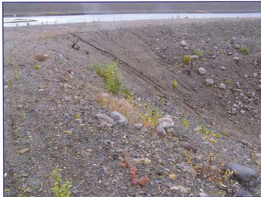
September: shows a view of some of the minor erosion that is occurring at the intersection of the crest and the left bank of the emergency spillway.
