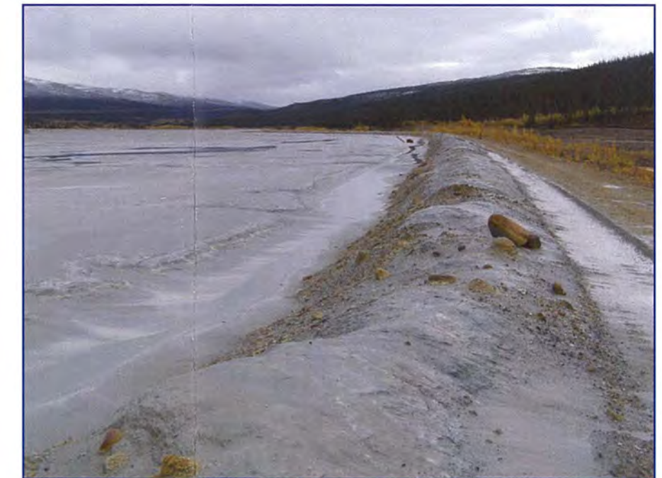
September: shows the upstream side of the dam with a piled tailings.
