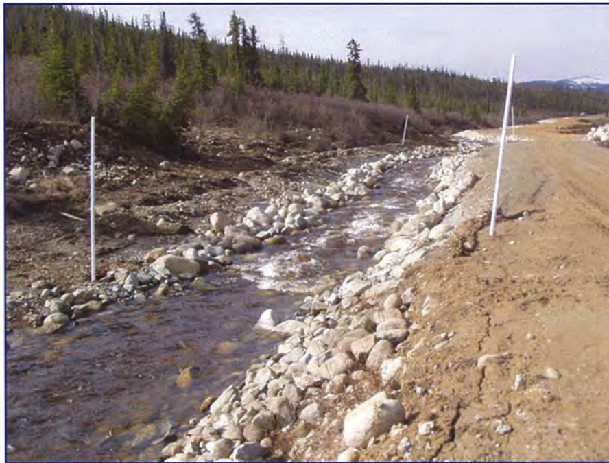
May: shows an downstream view of the area that was repaired in 2007. Note that some of the fill is soft and cracking.
