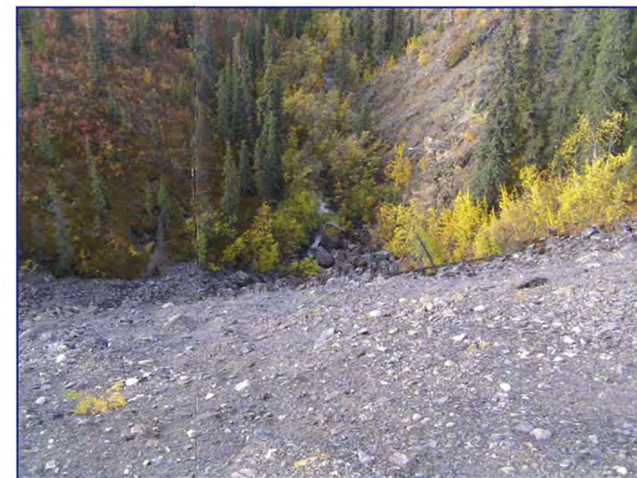
September: shows the downstream face of the rock drain with water flowing clearly from the toe.
