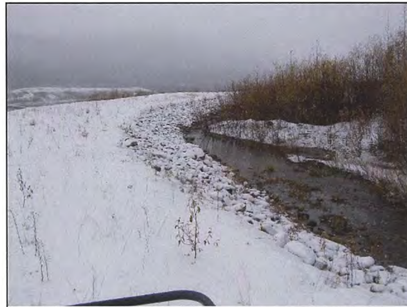
September: shows where the Interceptor Ditch comes up against the berm located proximal to the access road. We can see here that the water is adequately deflected and there does not appear to be any signs of erosion or deformation on this berm.
