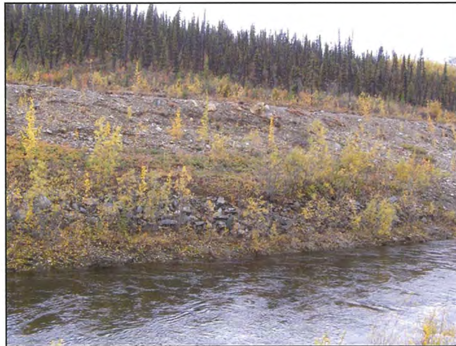
September: shows a slump area that has had some advancement over the past year. Repair is not yet needed.
