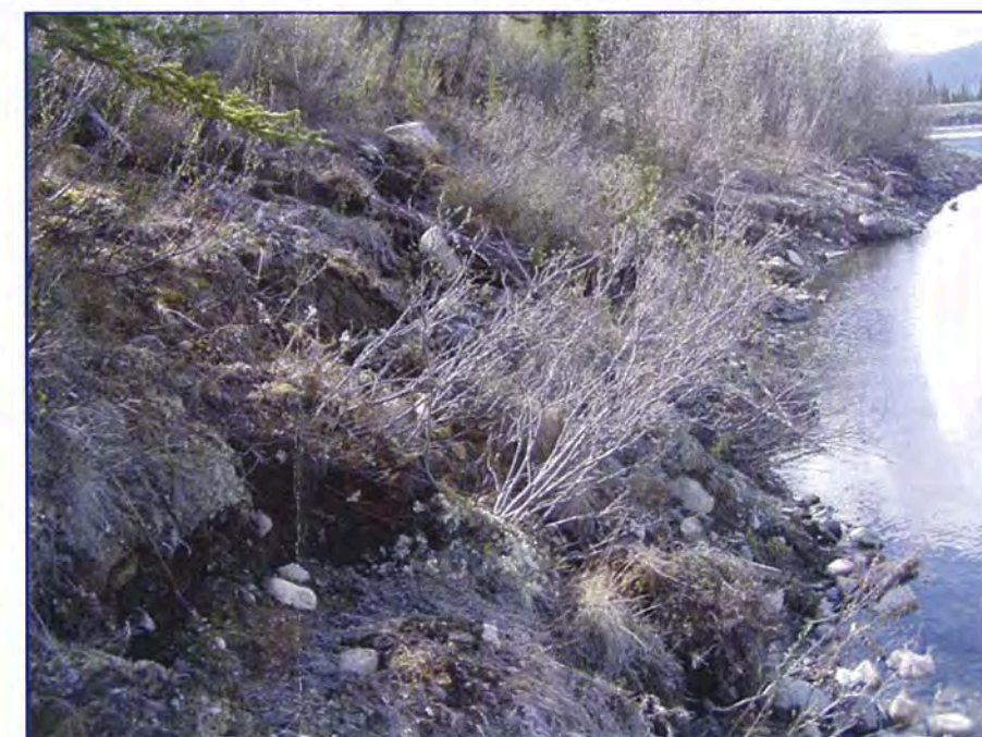
May: shows retrogression of bank in seepage discharge area.
