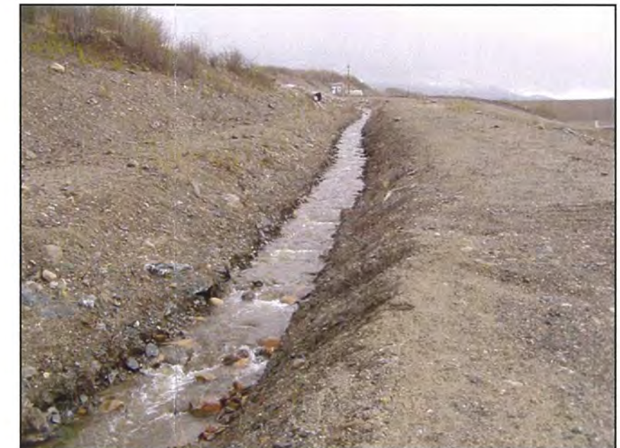
May: an upstream view of the North Valley Interceptor Ditch towards the culvert.
