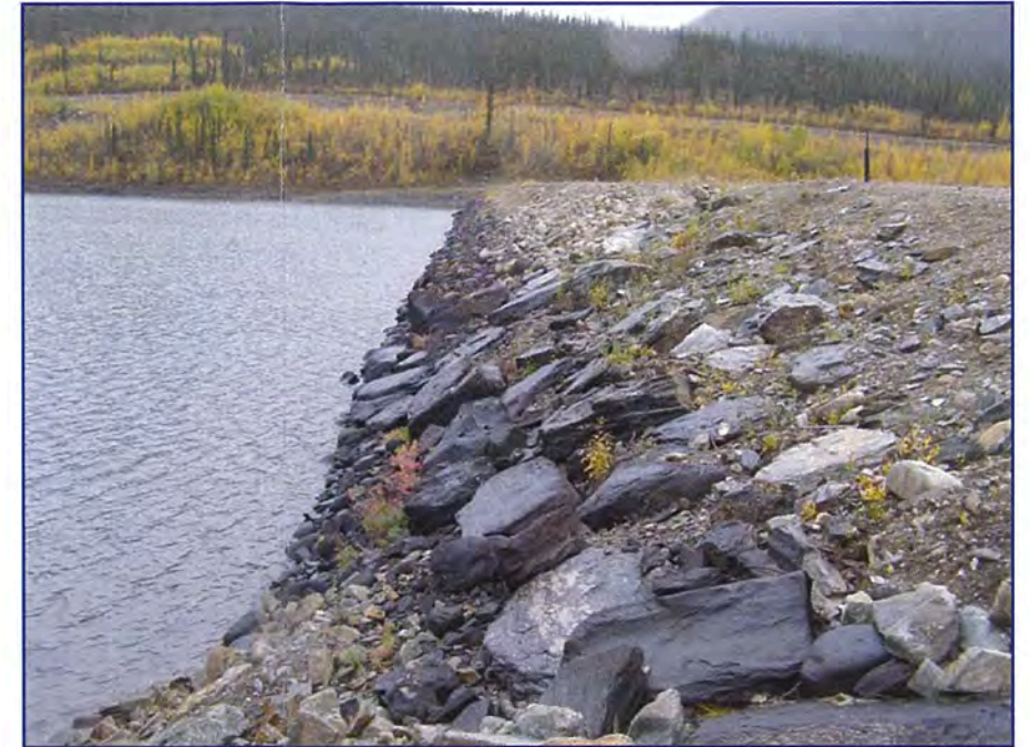
September: shows a view of the upstream face riprap and pond level.
