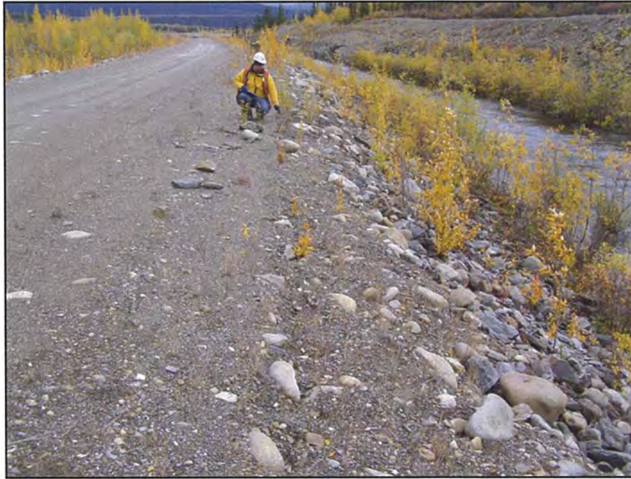
September: shows a tension crack that has formed on the upstream crest. The crack extends approximately 20 m and should be observed for further propagation and repair. Trees on the upstream slope should be removed next year.
