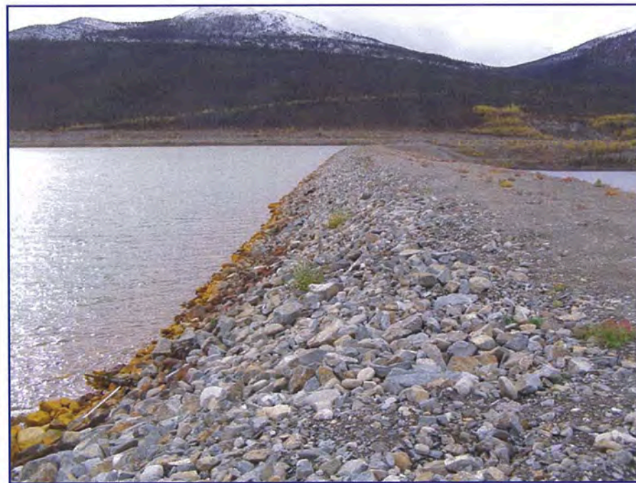
September: shows a view of the upstream face which was repaired in July 2007. Appears to be in good condition with no wave erosion occurring.
