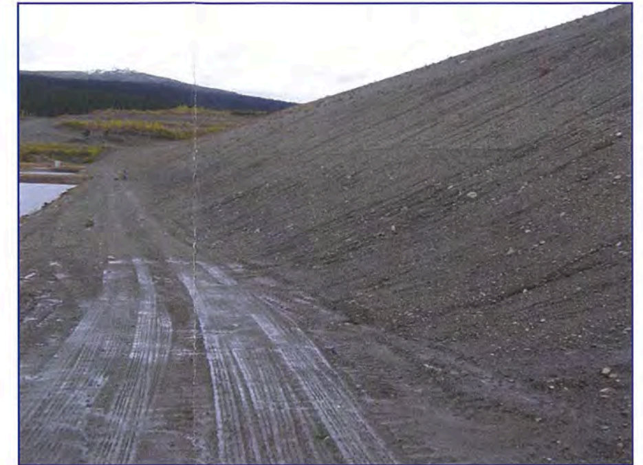
September: shows a view looking towards the right abutment down the lower road.
