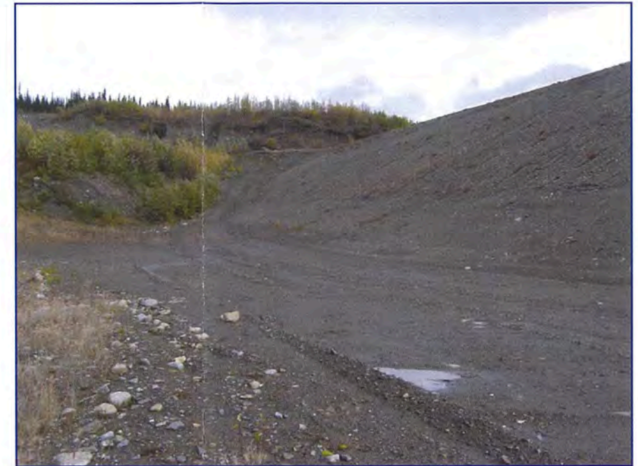
September: shows the intersection of the downstream face with the north abutment. Vegetation was removed and the area was graded for construction access in 2007.
