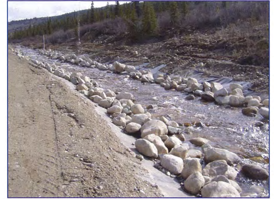
May: shows an upstream view of an area with geotextile exposure.
