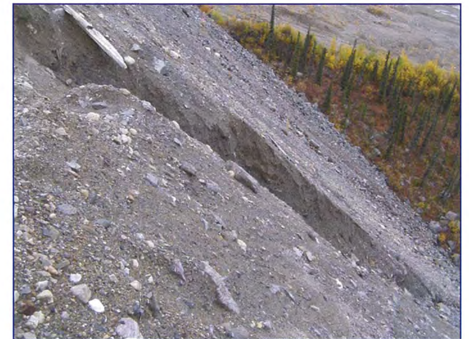
September: a view of the side slope of the drain and the erosion channel cutting through it. This erosion gap in the protection berm should be repaired to prevent further erosion on the face.
