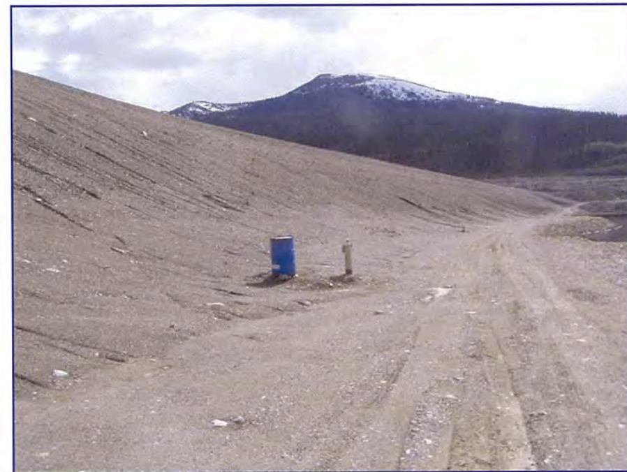
May: shows a view of the toe of the dam at the lower road. Note slough material at the toe.
