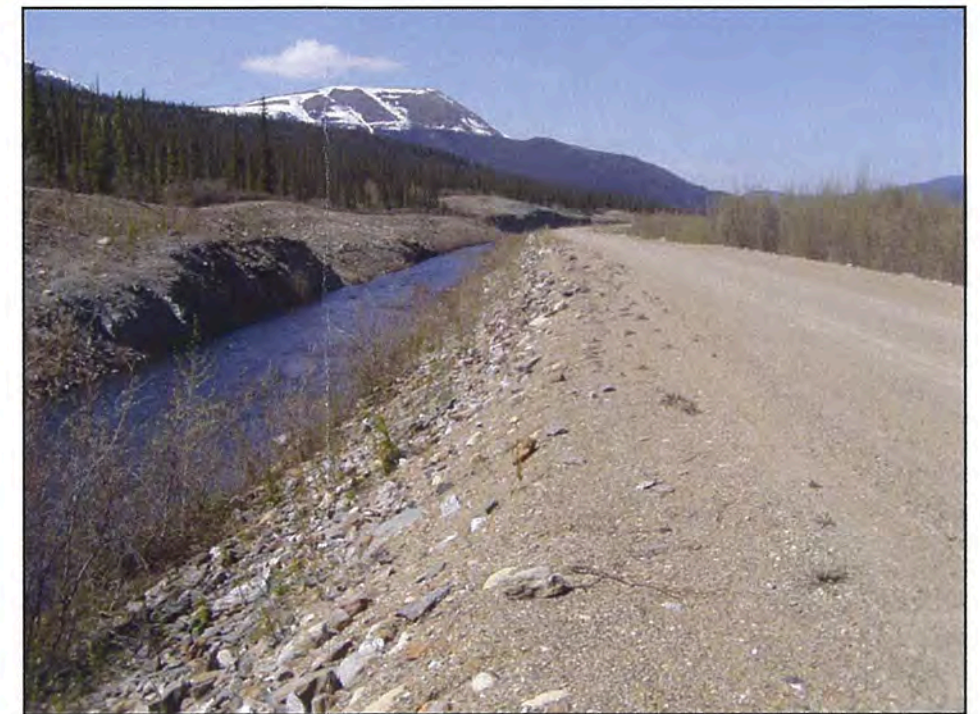
June: a view of the Diversion looking downstream. Note the bedrock outcrop on the left bank.
