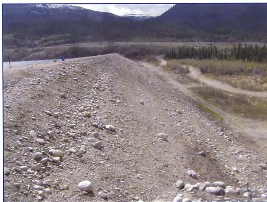
May: looking at the downstream face of the dam from the right abutment.
