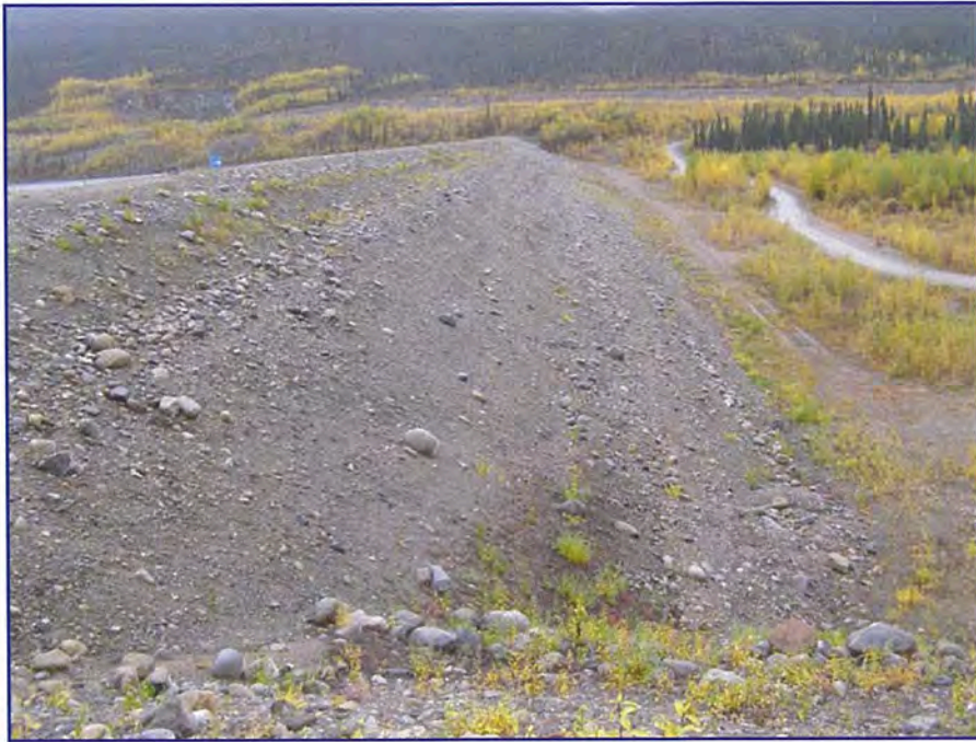
September: shows a view of the downstream shell of the Cross Valley Dam.
