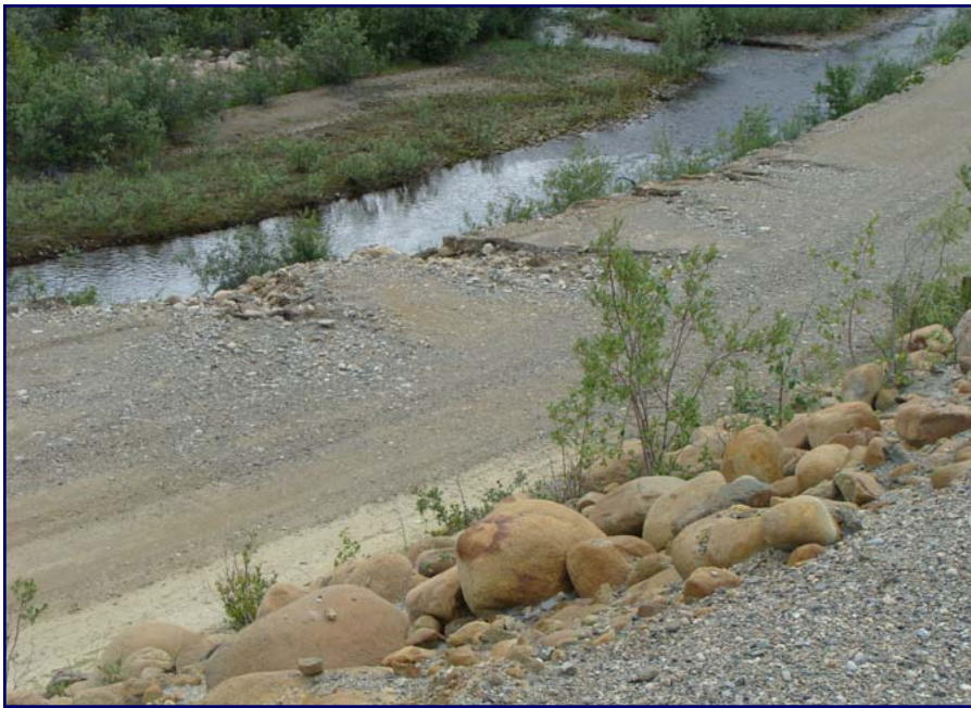
July: shows a view of erosion that is occurring on the lower road at the toe of the dam. This should be repaired by creating a channel to divert run-off.
