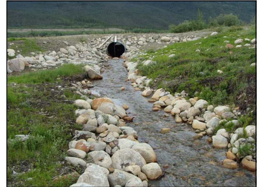
July: a downstream view of the North Valley Interceptor Ditch, looking at the culvert.
