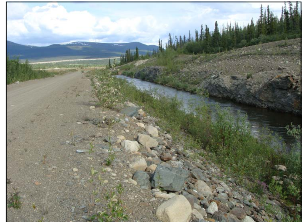
July: a view of the Diversion looking downstream. Note the bedrock outcrop on the right bank.
