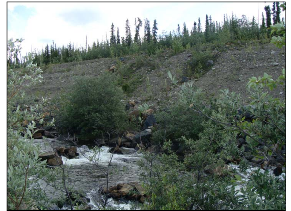
July: shows a view of some erosion gullies in the backslope of the canal.
