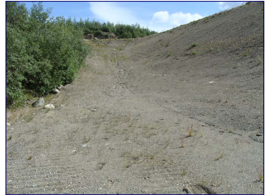
July: shows the intersection of the downstream face with the north abutment. Vegetation was removed and the area was graded for construction access in 2007.
