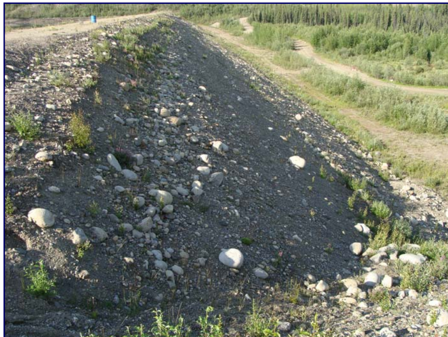
July: shows a view of the downstream shell of the Cross Valley Dam.
