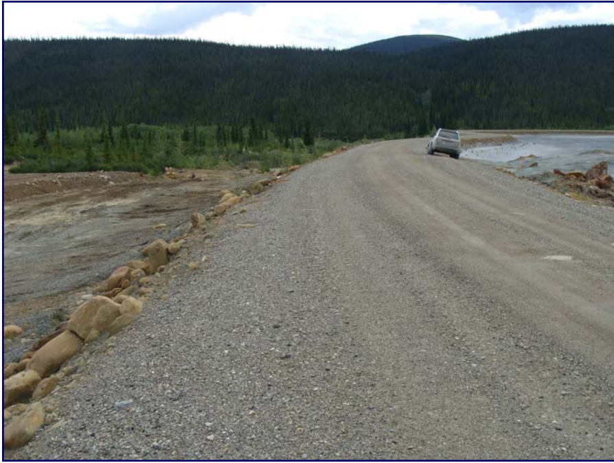
July: shows a view looking South down the crest of the Secondary Dam.
