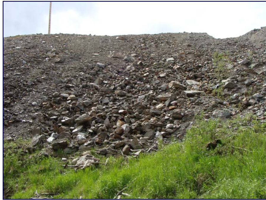
June: shows the face of the upstream side of the rock drain
