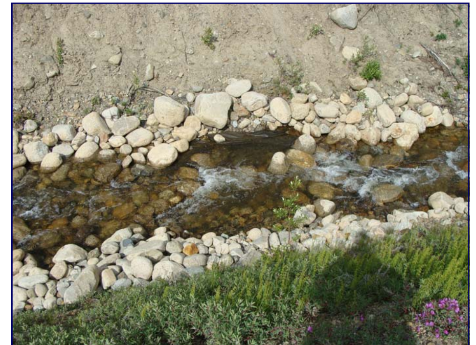
June: shows a view of the lower end of riprap placement in the Faro Creek Diversion. Riprap has been moved downstream and geotextile is exposed. No repairs needed.
