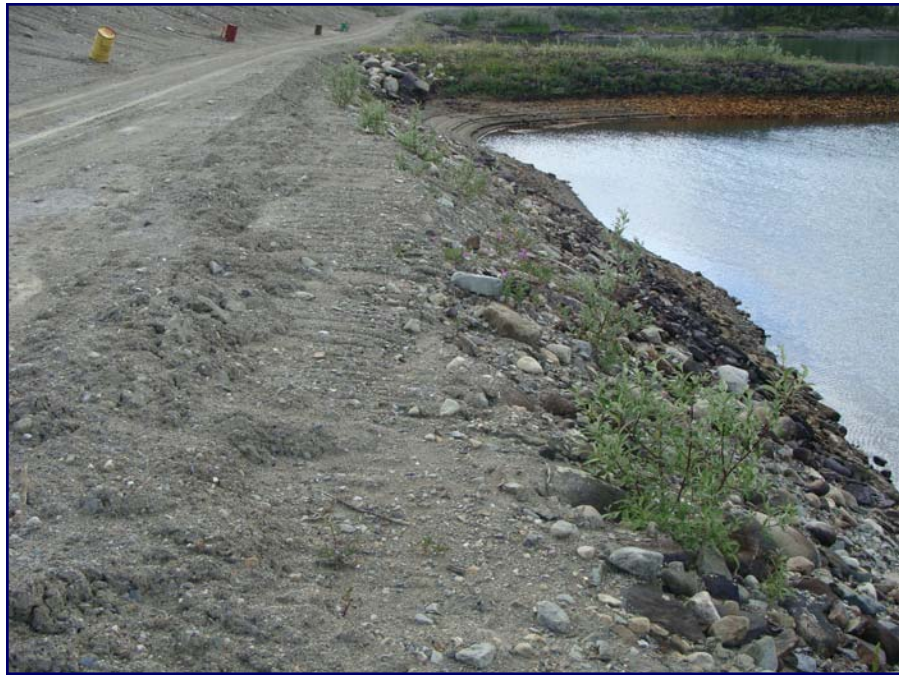
July: a view of minor cracking occurring at the edge of the polishing pond. Note that cracking has historically been seen in this area.
