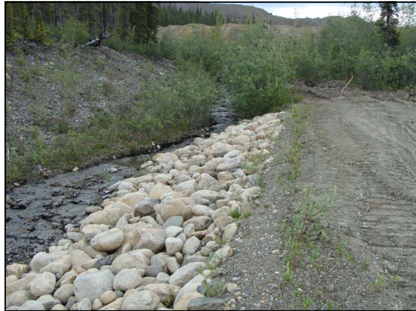
July: shows the start of the North Valley Interceptor Ditch just uphill from the guard house gate. This is the area the dike was repaired before and the riprap is present in the photo. After inspection of this section, it appears that the channel is flowing well with no signs of erosion or blockages.
