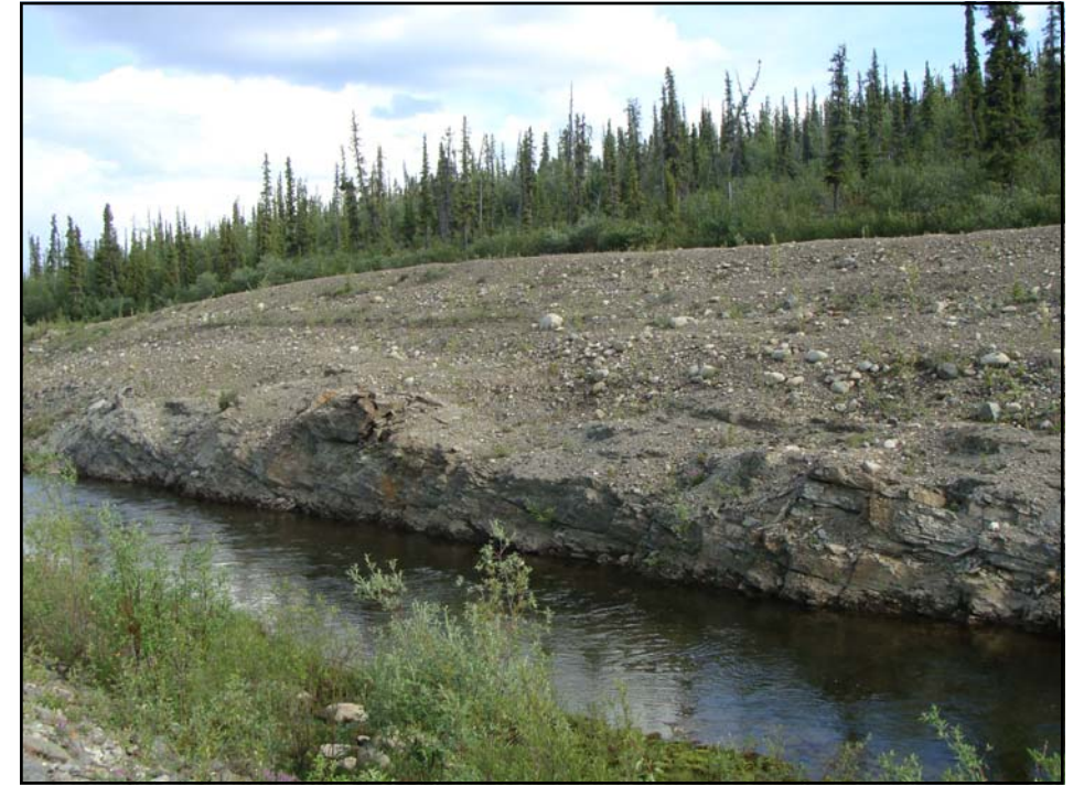
July: shows a view of the slump in the backslope of the Diversion Channel.
