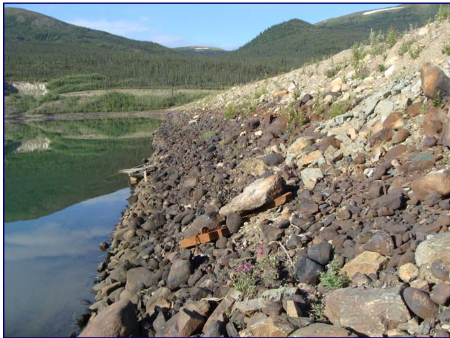
July: looking along the upstream face of the dam at the riprap. Note the water level is lower than the historic high water marks. Some ice plucking damage was noted in 2009, and should be monitored regularly in 2010.
