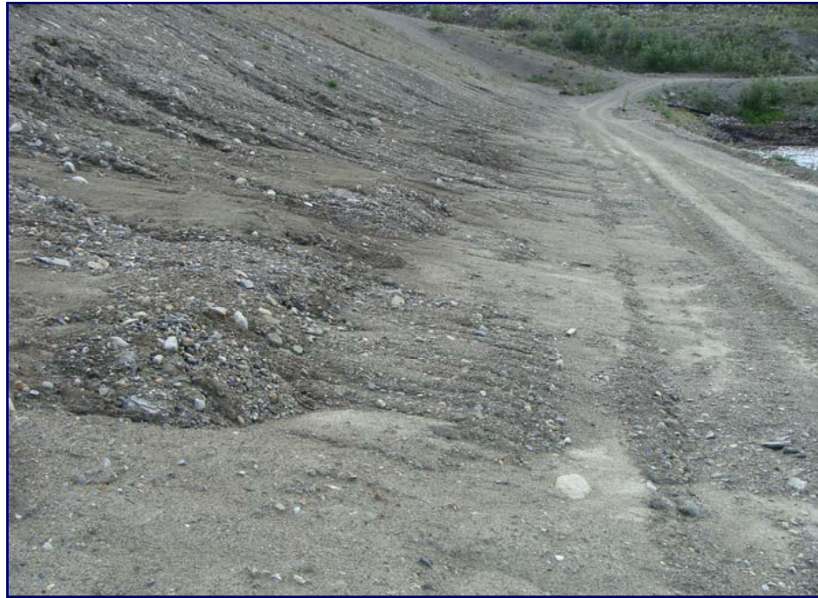
July: shows a view of erosion on the downstream face. This area should be repaired by removing the eroded sand and silt from the gravel drain outlet.
