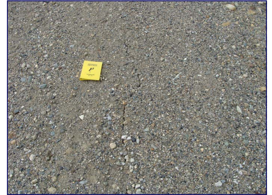
July: A faint crack in the crest of the dam on the tailings side. Monitor the area in 2010 for deterioration.
