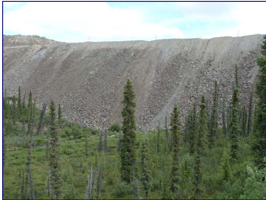
July: shows an overview of the downstream side of the North Fork Rock Drain. Note the erosion gully on the face.
