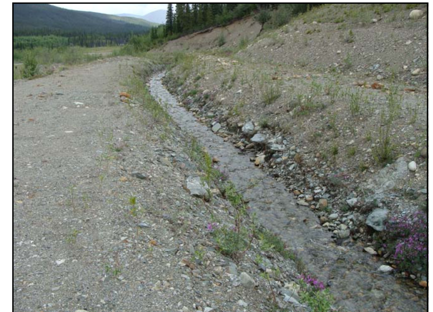
July: a downstream view of the North Valley Interceptor Ditch downstream of the culvert.
