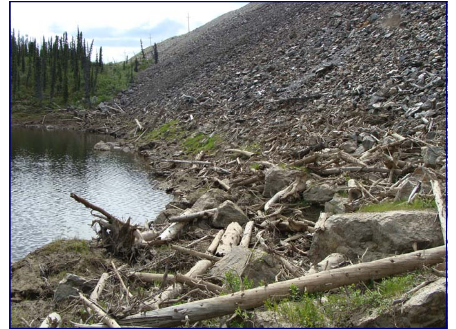
July: looking towards the east limit of the upstream pond. Note that the water level is approximately 3 m below the high water mark that is indicated by debris deposited on the face of the drain.
