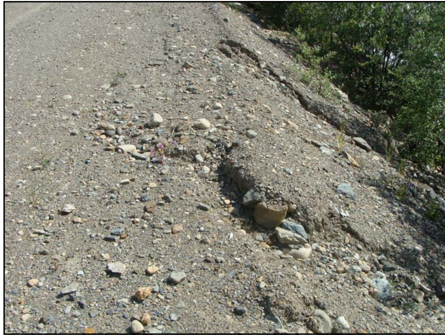
July: shows minor erosion occurring on road edge. Repairs not needed, but should be monitored.
