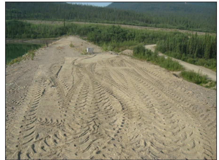
Site Staff Photo, July: shows a view of the crest and downstream face with re-graded compacted surface.
