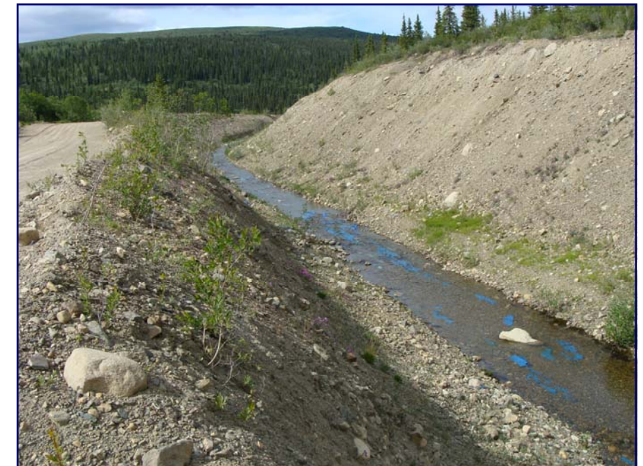
June: an upstream view of the channel, banks appear to be in good condition.
