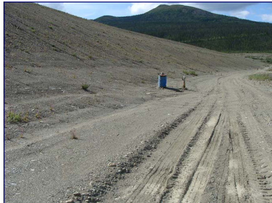
July: shows a view of the toe of the dam at the lower road. Note slough material at the toe.
