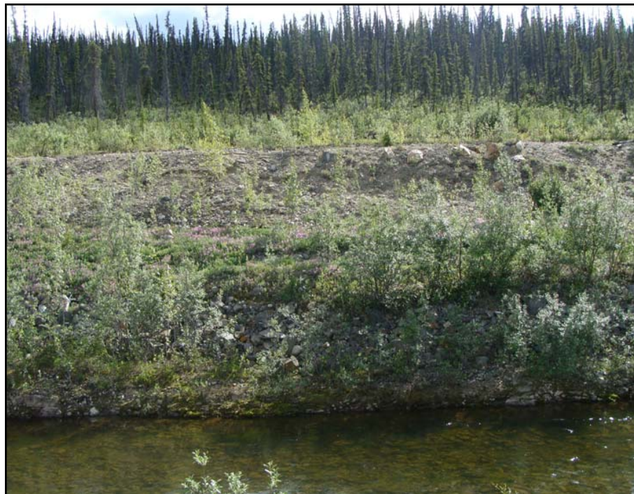
July: shows a slump area that has had some advancement over the past year. Repair is not yet needed.
