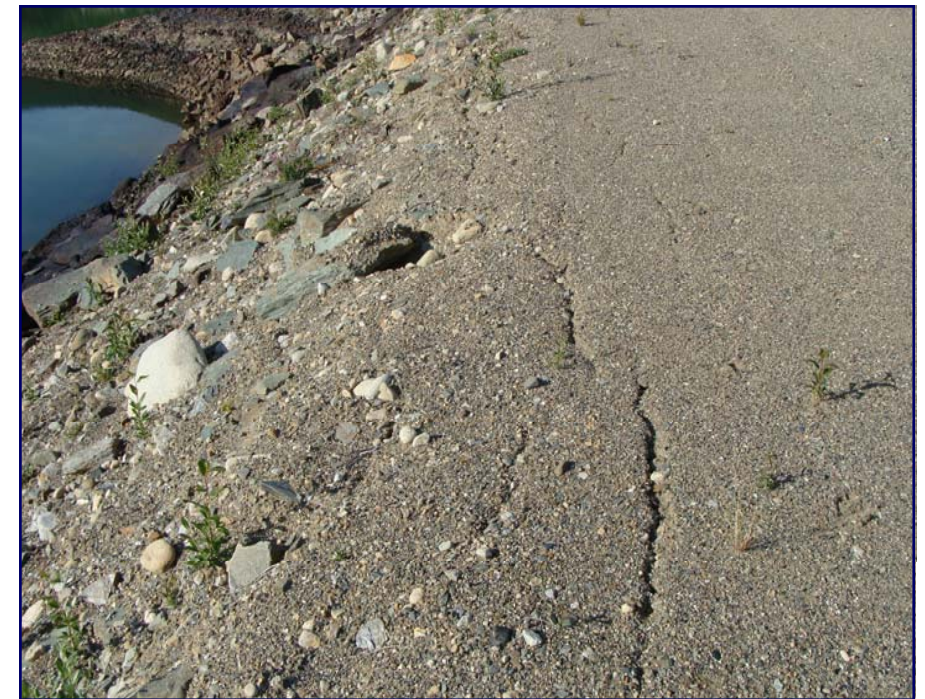
July: view of cracking in the upstream edge of the dam crest. This is likely due to frost action and should be graded and compacted.
