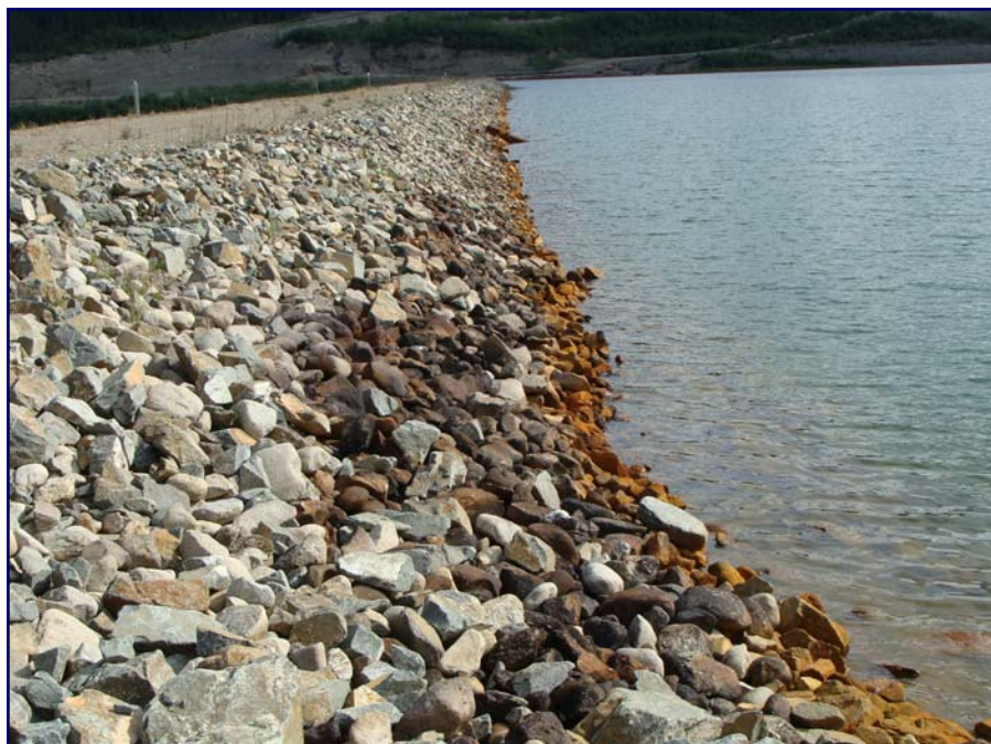
July: shows a view of the upstream face which was repaired in July 2007. Appears to be in good condition with no wave erosion occurring.
