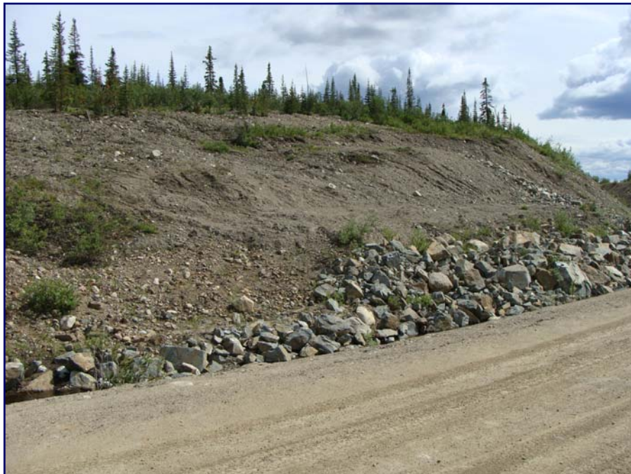
June: shows the slope stability repair zone in the backslope. Note the slumping of the disturbed ground.
