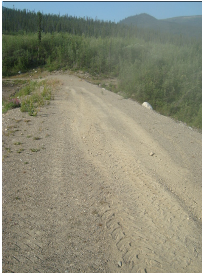
Site Staff Photo, July: shows the crest of the dam after the crack has been repaired.
