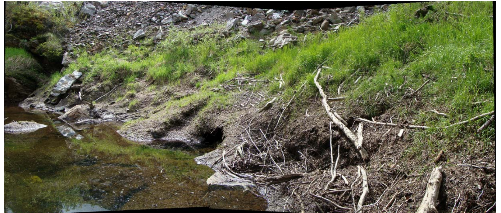
June: a view of the sediment and grass that is present on the upstream face of the rock drain.
