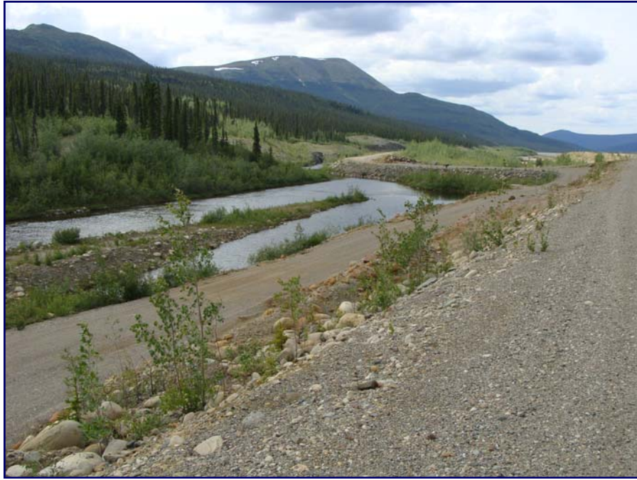
July: shows the downstream side of the Secondary Dam. Note the pond at the Diversion Dam in the background.
