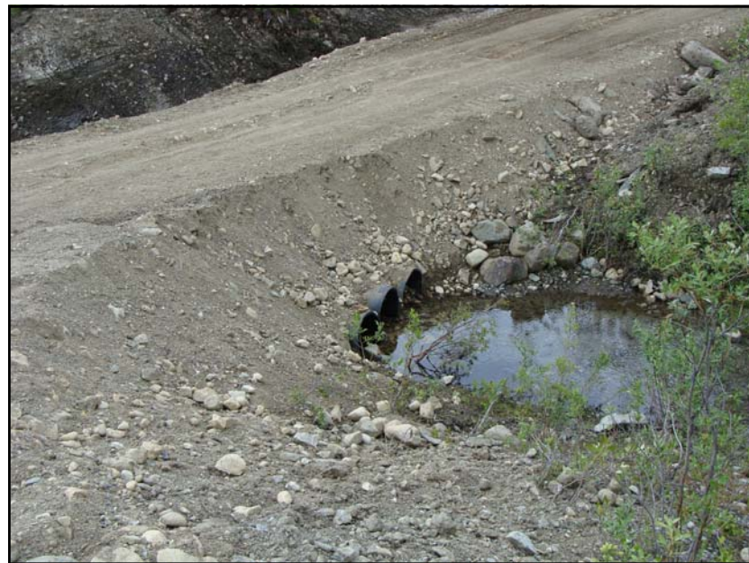
July: shows a new crossing that has been made over the North Valley Interceptor Ditch. Culverts were installed to allow water to flow though.
