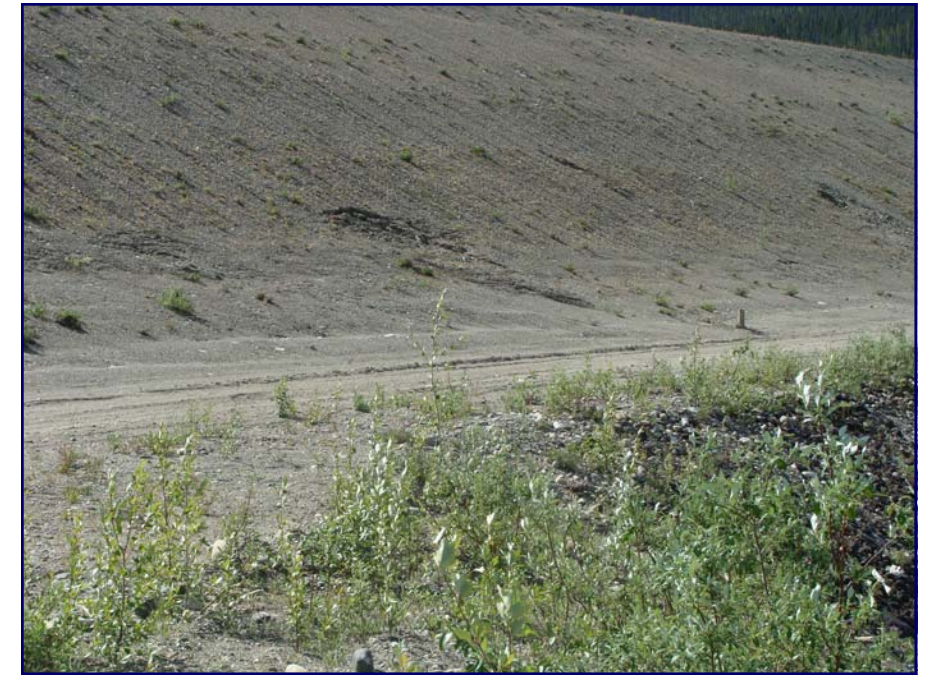
July: shows some minor slumping that is occurring on the face of the downstream side of the dam.
