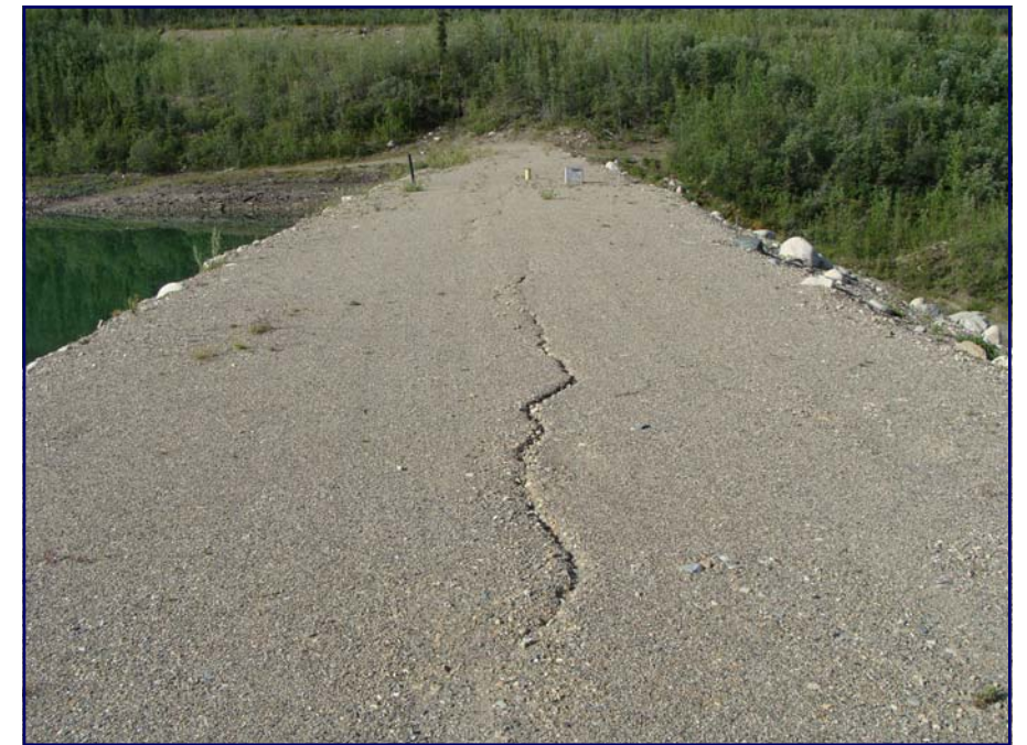
July: shows a crack in the crest of the dam. This is due to frost action and the area should be graded and compacted.
