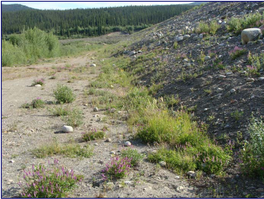
July: shows a view of the downstream toe. Note the concentration of vegetation at the toe. This should be removed.
