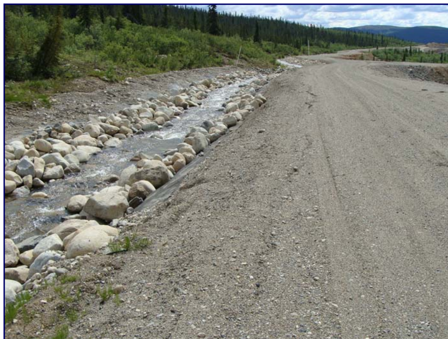
June: shows an downstream view of the area that was repaired in 2007. Note that some of the fill is soft and cracking.
