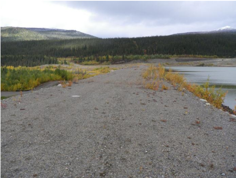
Photo 42 Dam crest along southwest segment – looking northeast, note no visible longitudinal cracks on crest surface (September 11, 2012)
