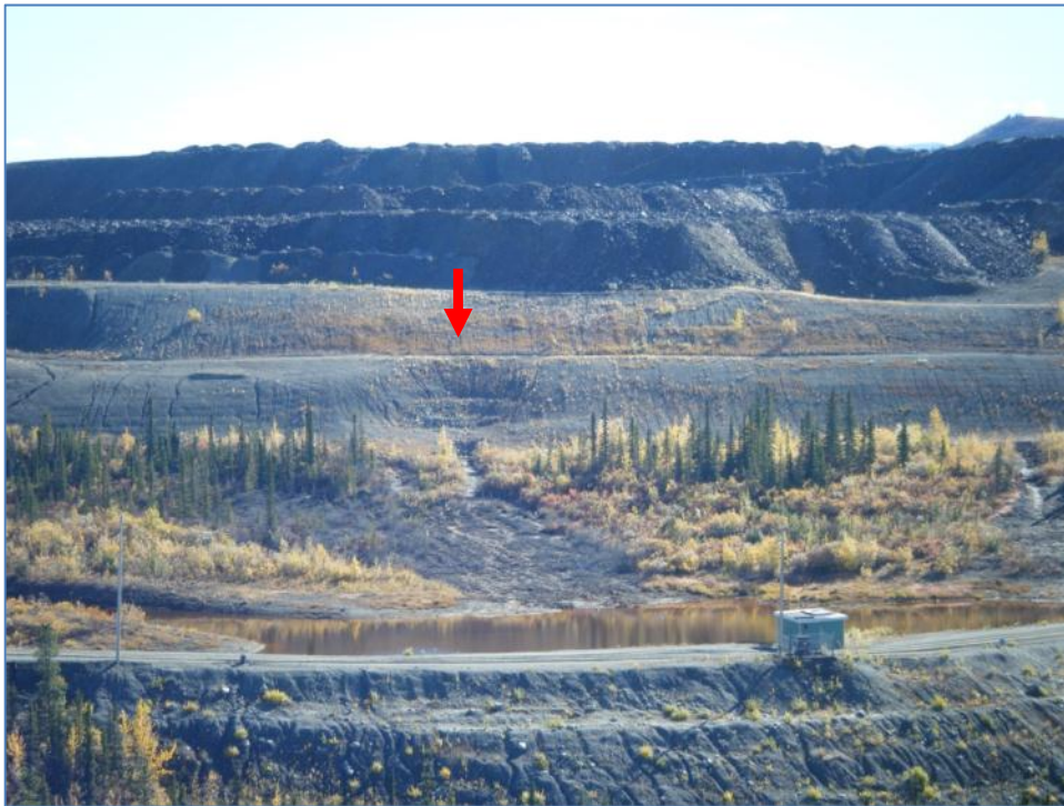
Photo 62 Waste Dump previously noted subsidence at the arrow (September 20, 2012)
