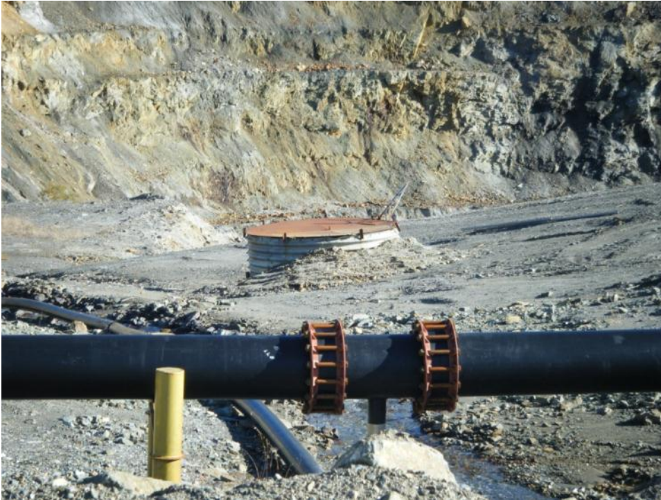
Photo 94 Flow drop box downstream of Vangorda Flume (September 20, 2012)
