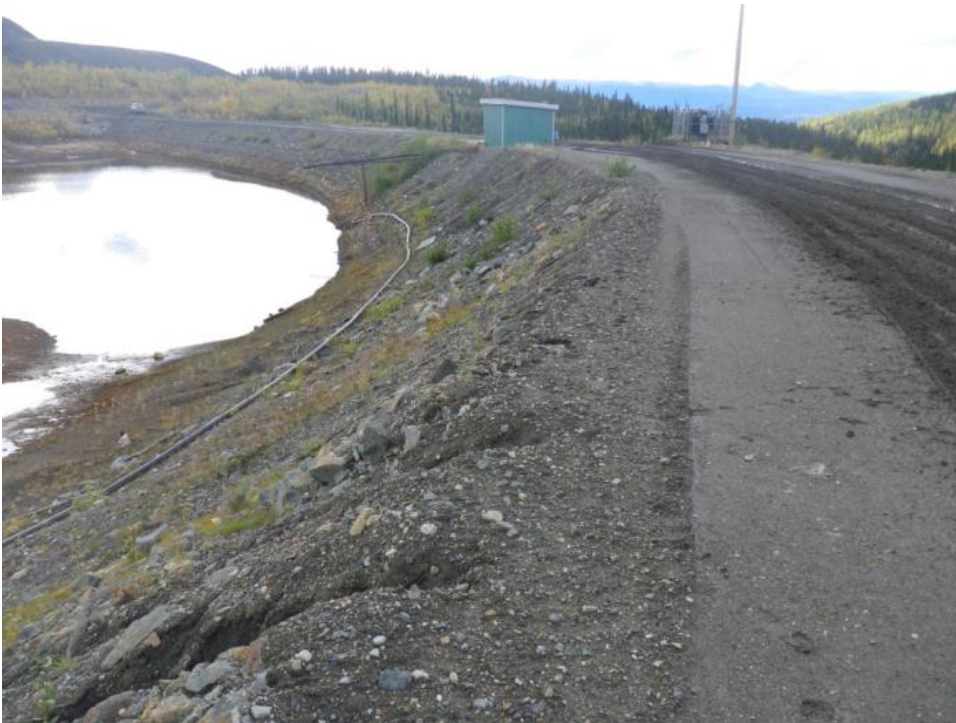
Photo 97 Dam crest and upstream slope - rill erosions in the foreground (September 13, 2012)
