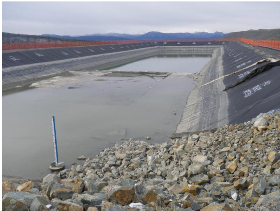
Photo 58 Grum Sulphide Cell water storage pond constructed in 2011 – view in longitudinal direction (September 12, 2012)
