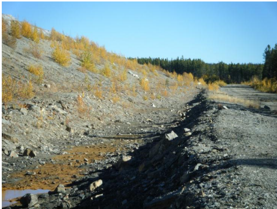
Photo 72 Vangorda Waste Dump Seepage Collection Ditch at Drain No. 3 - looking upstream (September 20, 2012)
