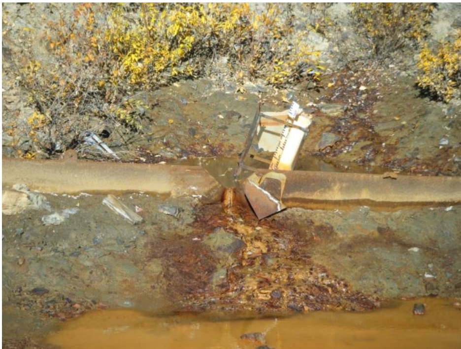
Photo 71 Vangorda Waste Dump Drain No. 3 weir - note delaminated weir plate and crooked staff gauge (September 20, 2012)
