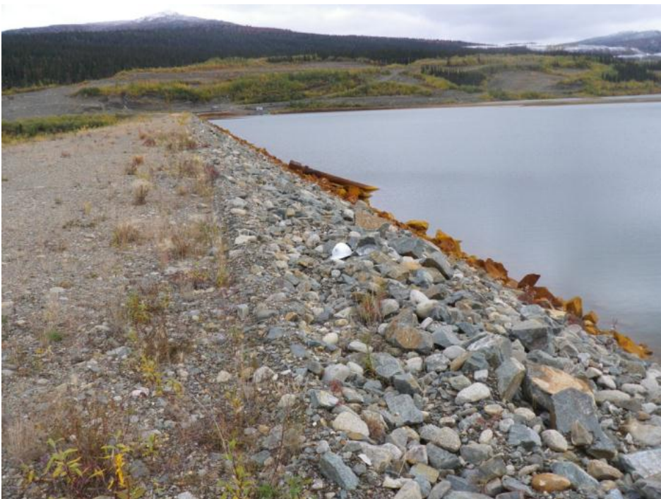
Photo 30 Dam crest and upstream slope – note fill adjustment near crest shoulder marked by hard hat (September 11, 2012)
