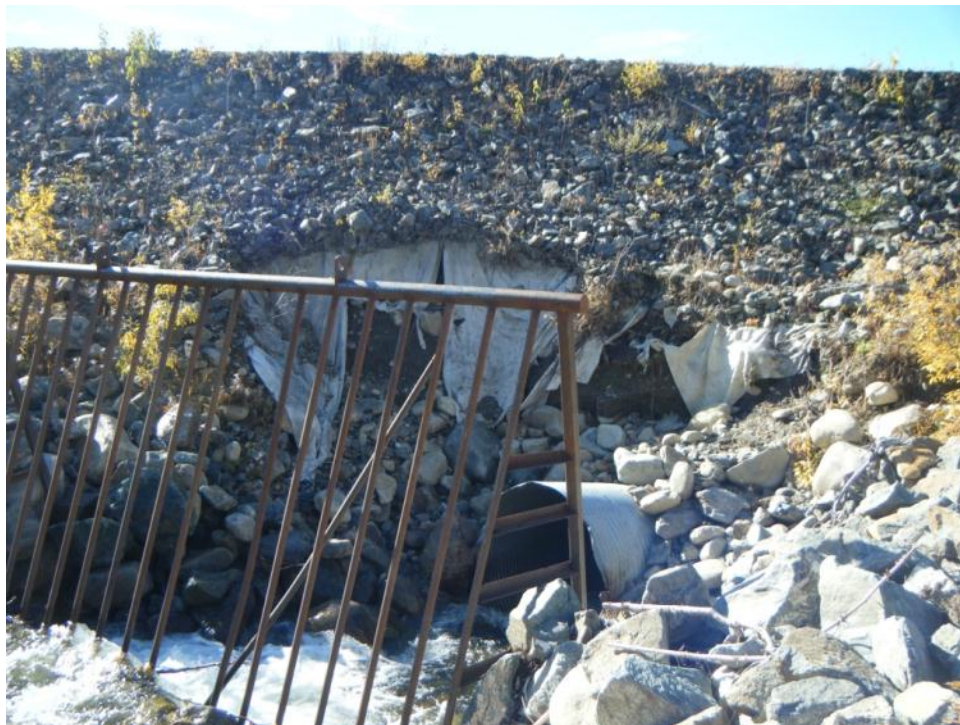
Photo 85 Vangorda Flume intake culvert – note considerable embankment toe erosion around culvert (September 20, 2012)
