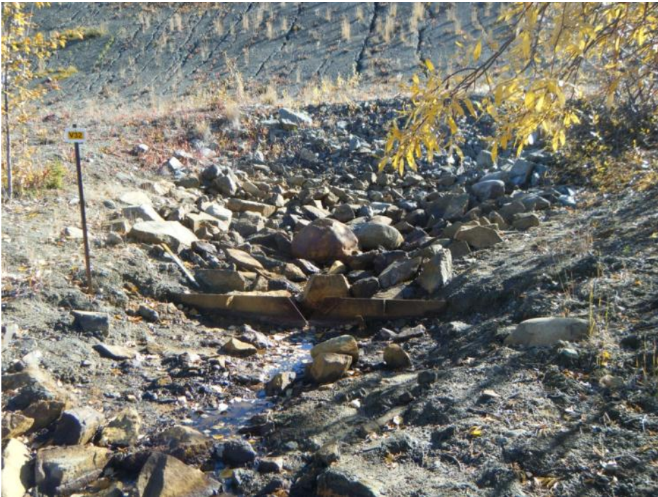
Photo 67 Vangorda Waste Dump Drain No. 5. Weir – looking upstream (September 20, 2012)
