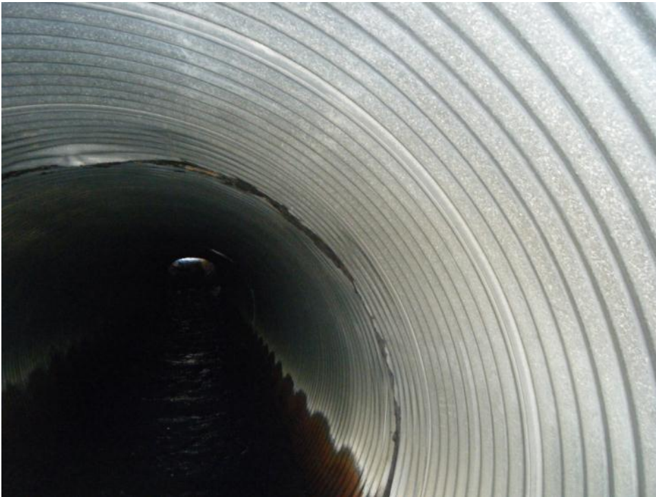
Photo 88 Flume intake culvert as seen from downstream end - first pipe joint appears to be separated (September 20, 2012)
