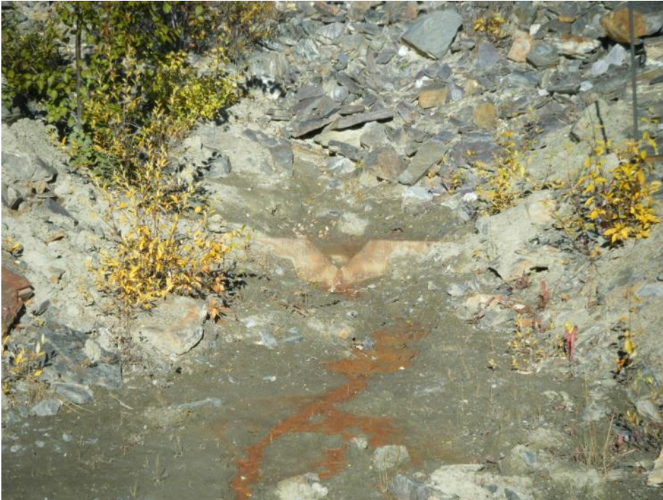
Photo 74 Vangorda Waste Dump Drain No. 2 weir (September 20, 2012)
