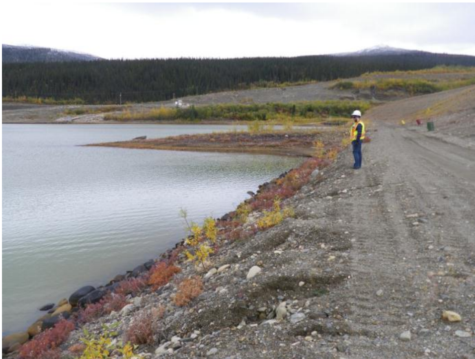
Photo 36 Downstream berm - note rill erosion on berm shoulder in the foreground (September 11, 2012)
