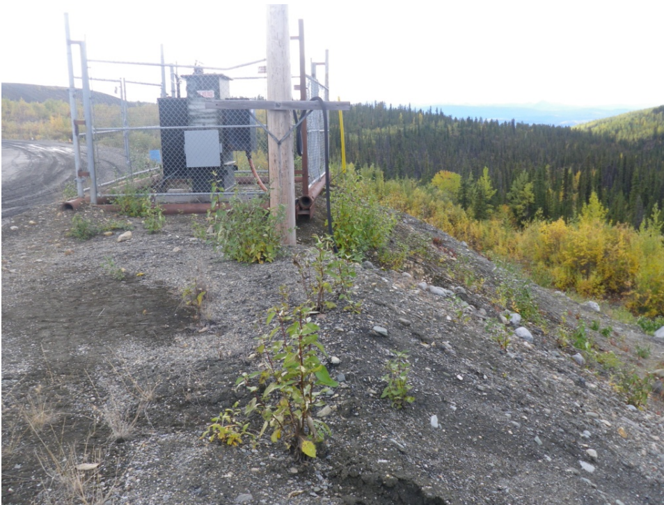
Photo 99 Rill erosions near transformer on dam crest (September 13, 2012)
