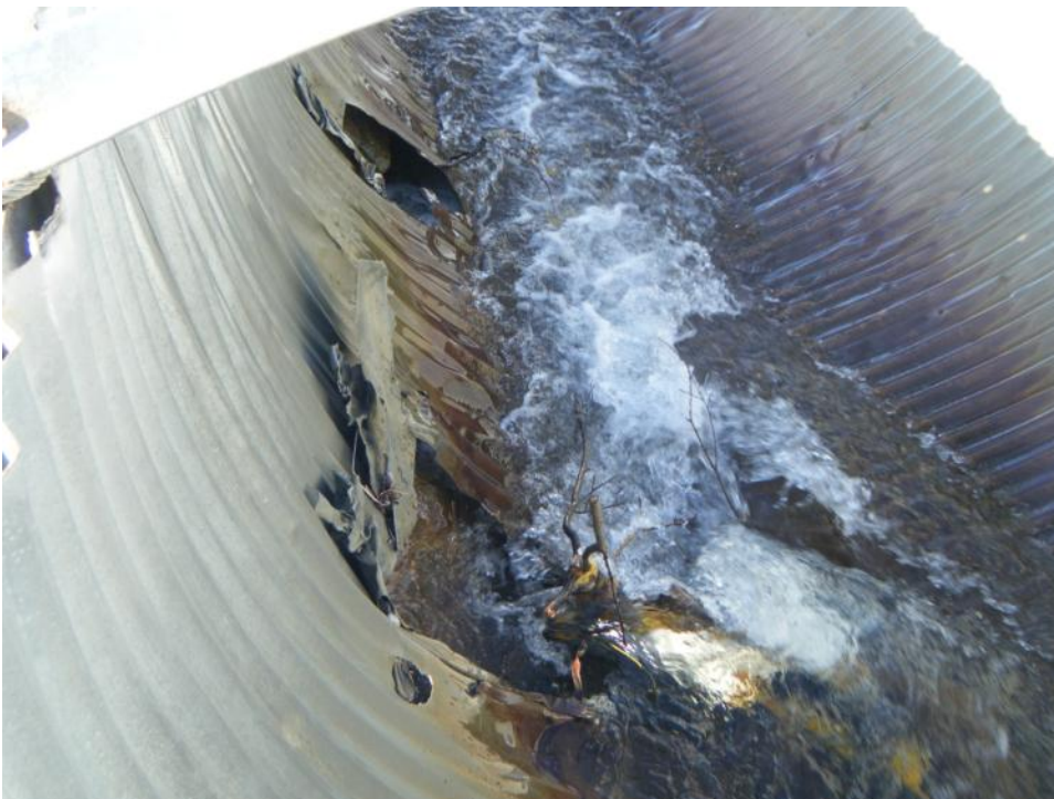
Photo 91 Damaged Flume (September 20, 2012)
