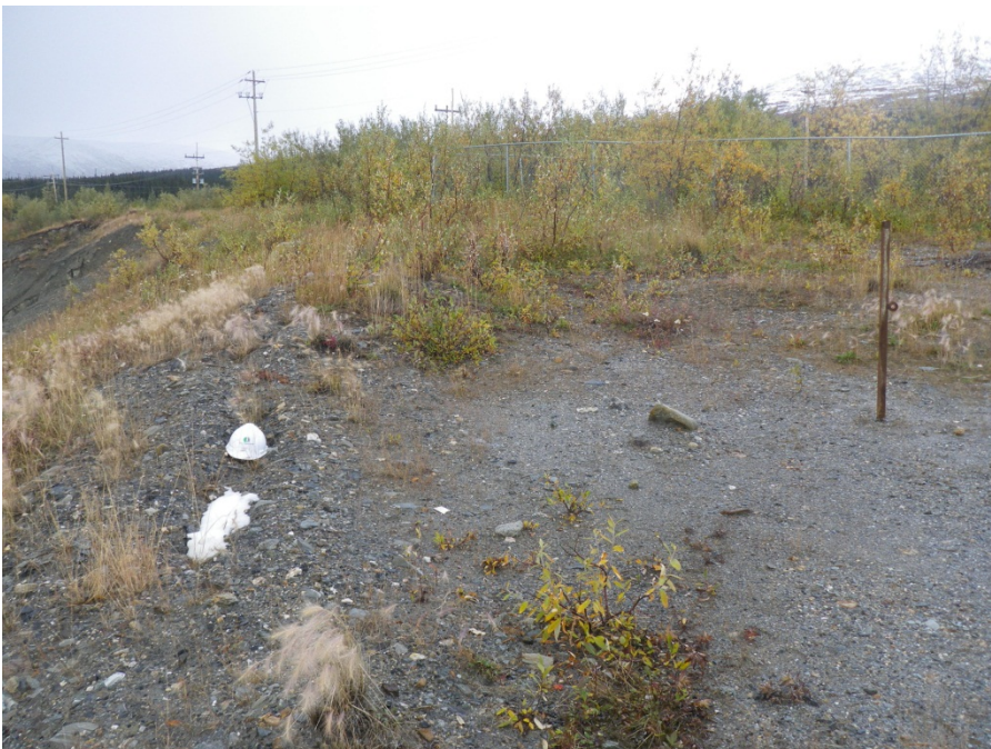
Photo 53 Reference Rod SP-1 along south array – ground deformation noted at hard-hat location (September 12, 2012)
