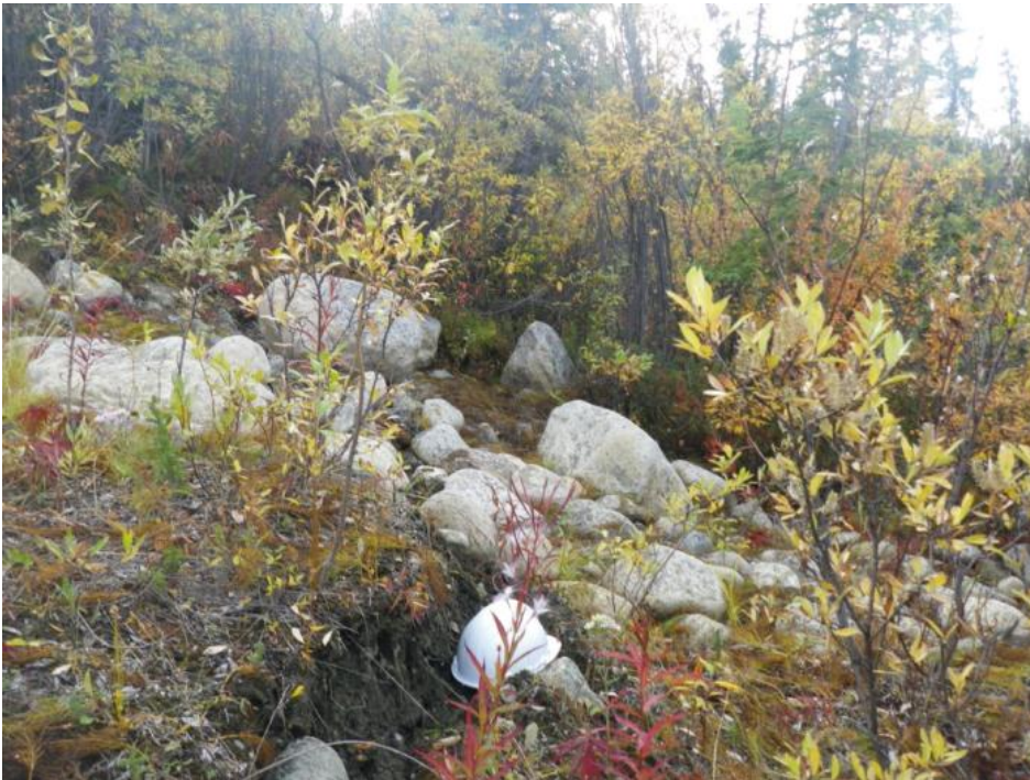
Photo 106 Close up of crack across spillway channel shown on Photo ____ (September 13, 2012)
