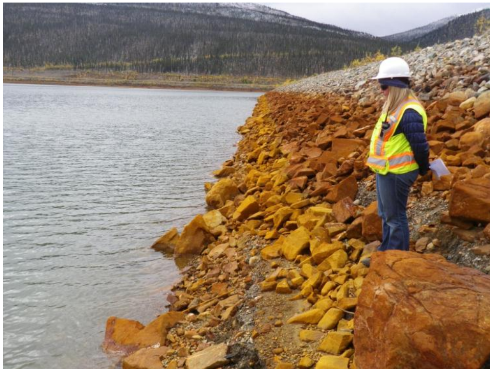
Photo 26 Wave erosion zone on upstream slope – note marker rod installed by Brodie in 2010 in the foreground (September 11, 2012)
