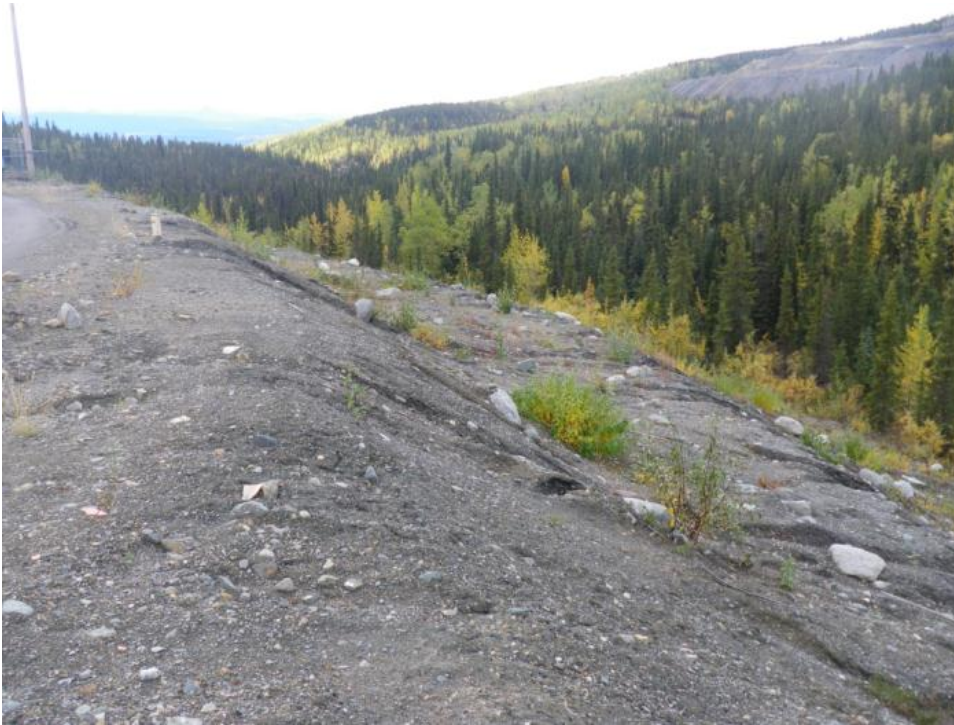
Photo 98 Rill erosions on downstream slope (September 13, 2012)
