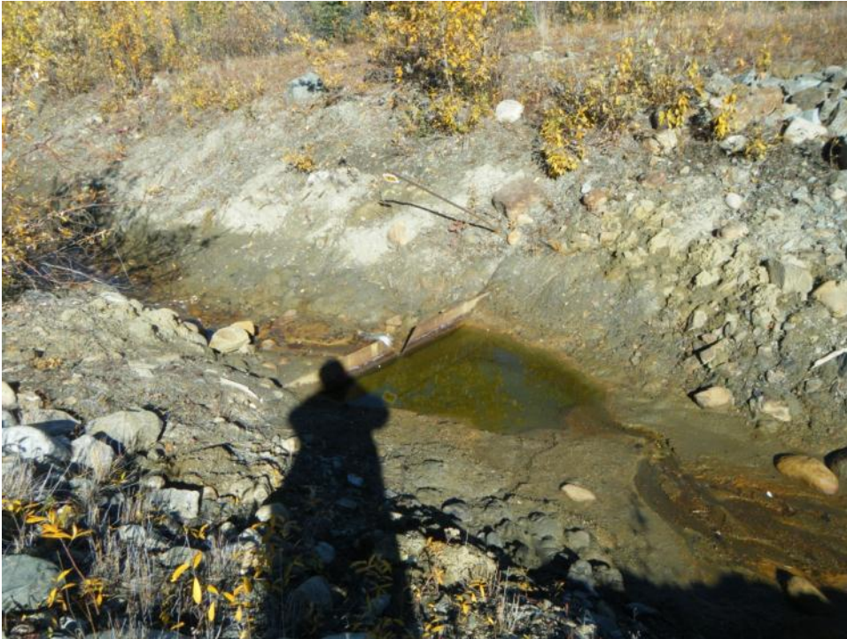
Photo 66 Vangorda Waste Dump Drain No. 6 Weir (September 20, 2012)
