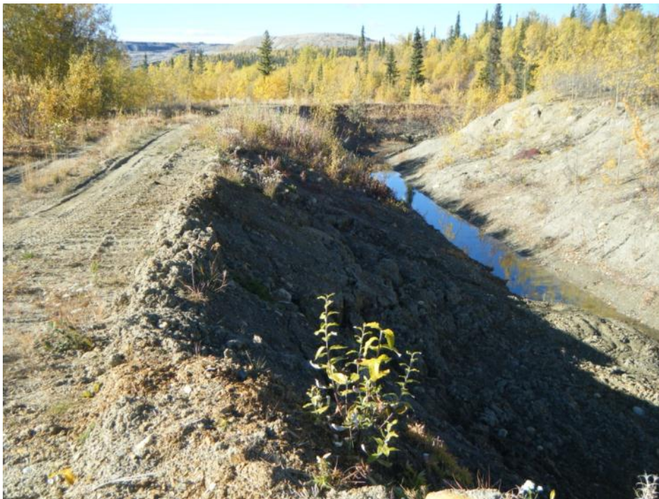
Photo 83 Interceptor Ditch – looking upstream, note slumped road slope (September 20, 2012)
