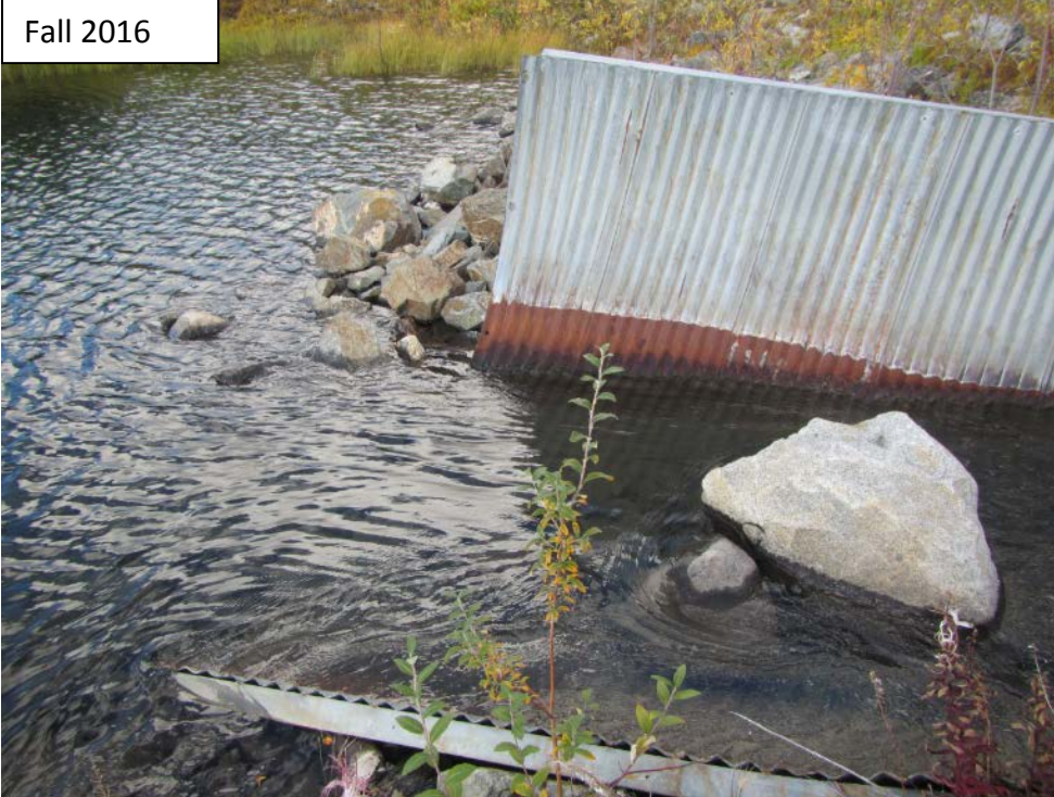
Photograph 59 Upper end of spillway from the Upper to Lower Sediment Pond. Boulders impeding flow.
