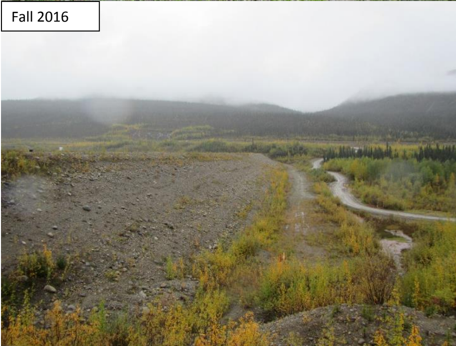
Photograph 29 Downstream slope of Cross Valley Dam looking south. Some minor rill erosion and vegetation on slope. Conditions are similar across the whole slope.
