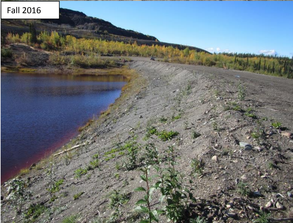
Photograph 56 Little Creek Dam upstream slope, repaired rill erosion. Minor vegetation.
