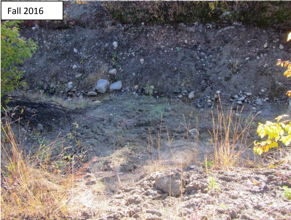
Photograph 44 Slumping on road slope. Progressed slightly since spring.
