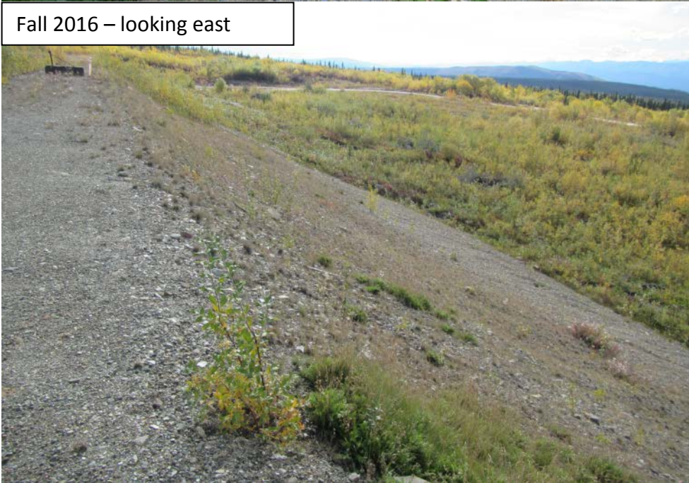
Photograph 66 Clarification pond, dyke crest and downstream slope. Some trees to be removed.
