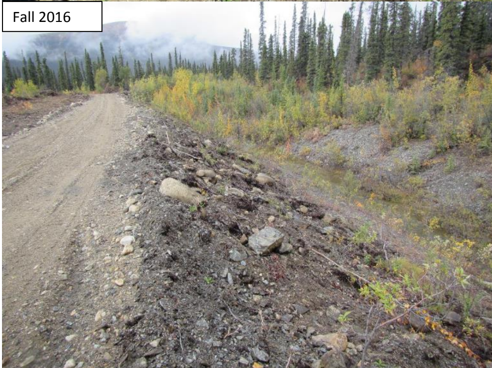
Photograph 7 Interceptor Ditch upper man-made reach - vegetation roots were removed in fall 2016. Erosion control measures should be implemented in spring 2017. Approximately 565 m from the diversion inlet.
