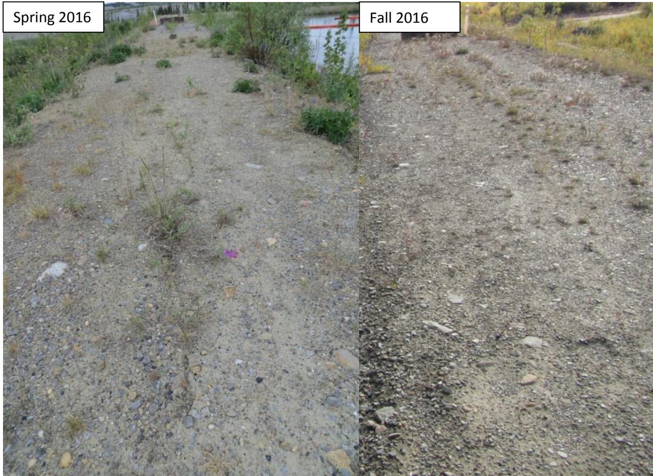
Photograph 68 Clarification pond, longitudinal freeze-thaw cracks. Not as evident in the fall.
