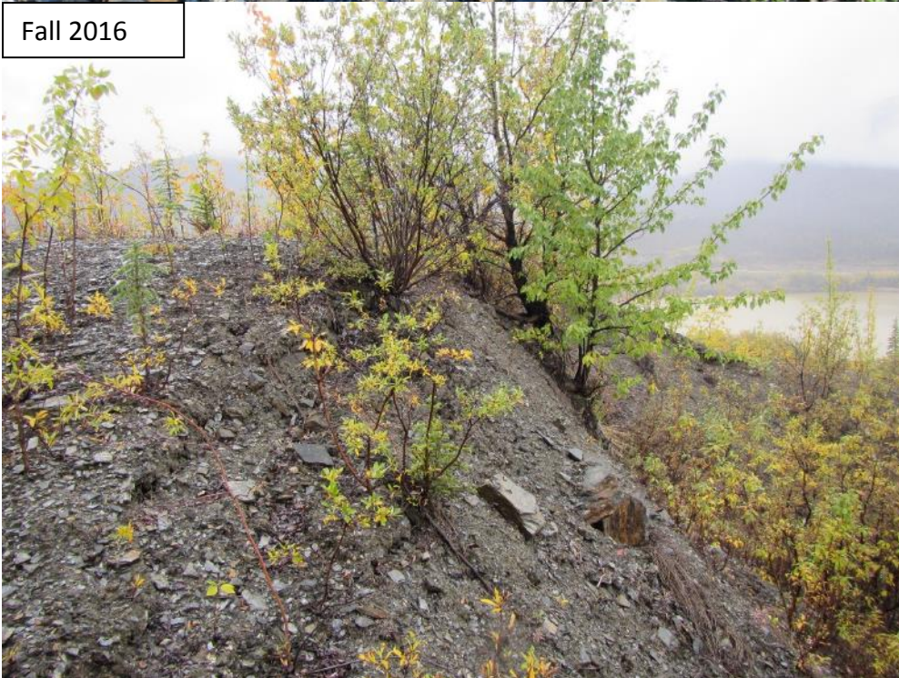
Photograph 10 Slumping at the End of the Middle Reach. Similar conditions in spring and fall. Approximately 2150 m from the diversion inlet.
