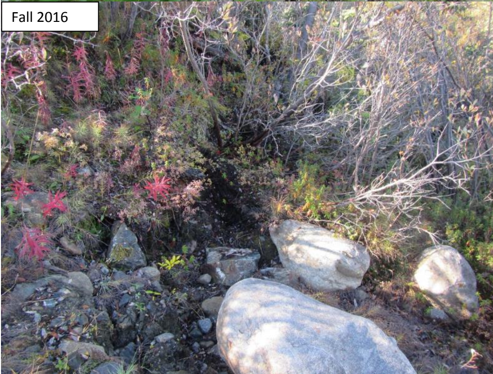
Photograph 58 Ground slope crack across downstream spillway channel near discharge end. Similar conditions in spring and fall.
