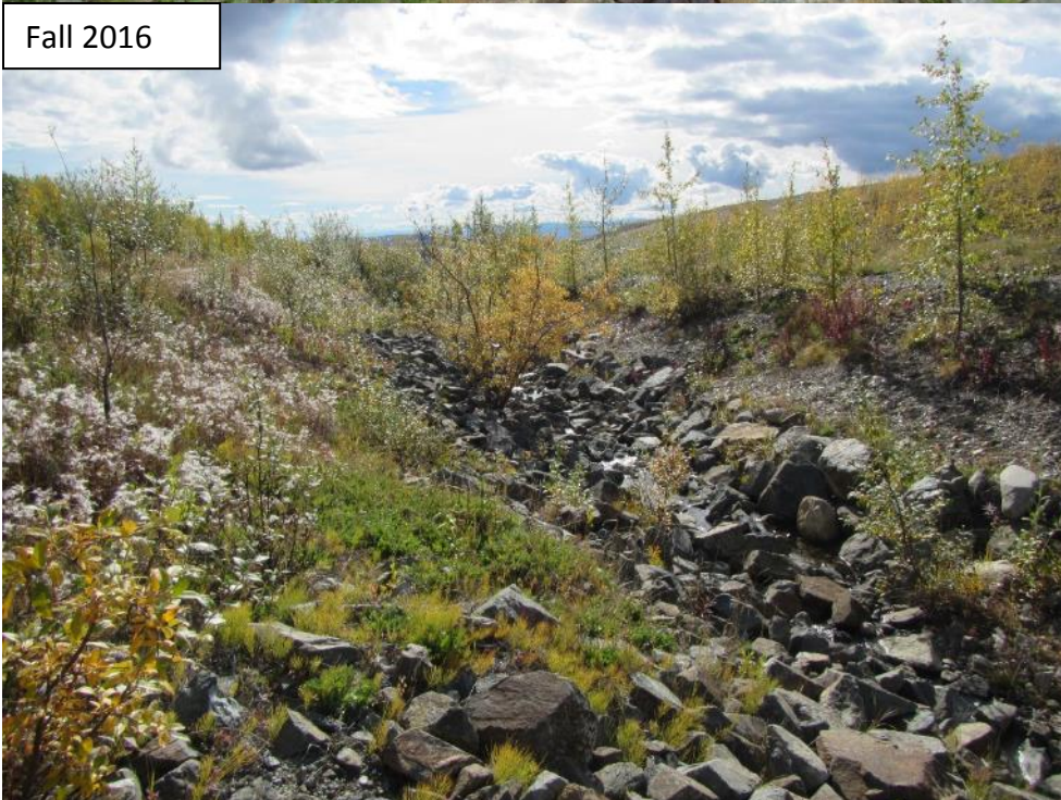
Photograph 61 Pond spillway channel, looking downstream towards Grum Interceptor Ditch. Trees on embankment and in spillway should be removed.
