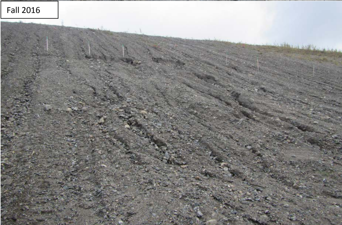
Photograph 27 Repairs along downstream slope. Some surface erosion since spring.
