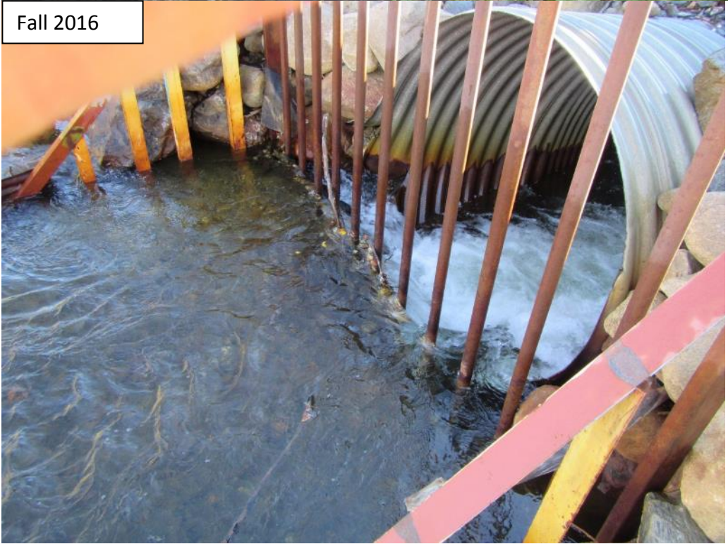
Photograph 52 Outlet to Flume Plunge Pool - trash rack. Leaves and woody debris accumulate on the trash rack and need to be removed as part of regular maintenance.
