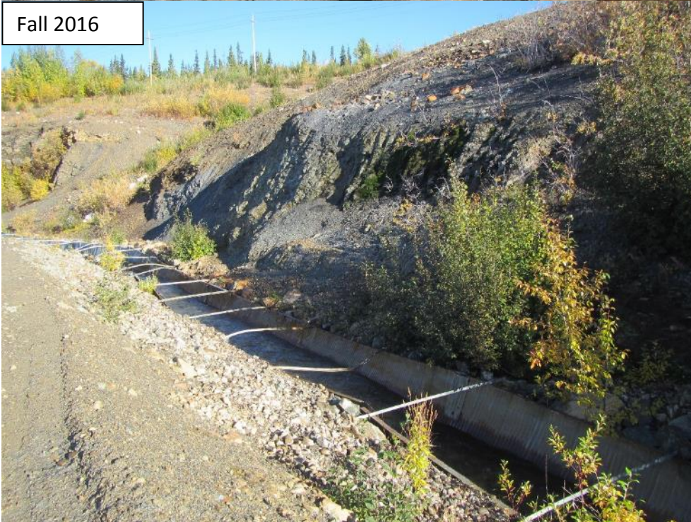
Photograph 48 Damaged flume and bent bracing rods
