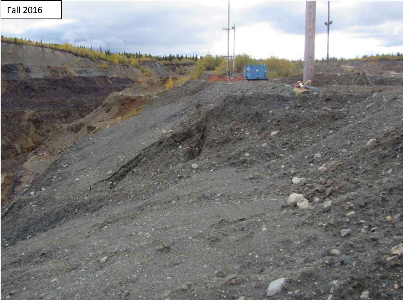
Photograph 36 Vangorda Diversion Sinkhole showing signs of settlement.
