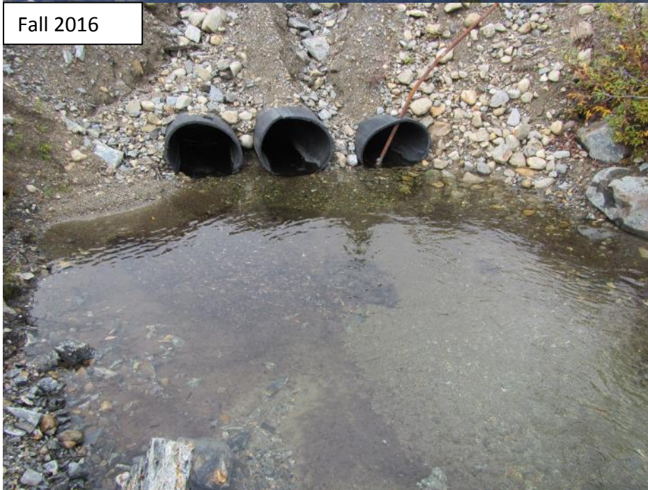
Photograph 8 Interceptor Ditch (Faro Creek) upstream side of the well access road. Satisfactory conditions. Approximately 255 m from the diversion inlet.
