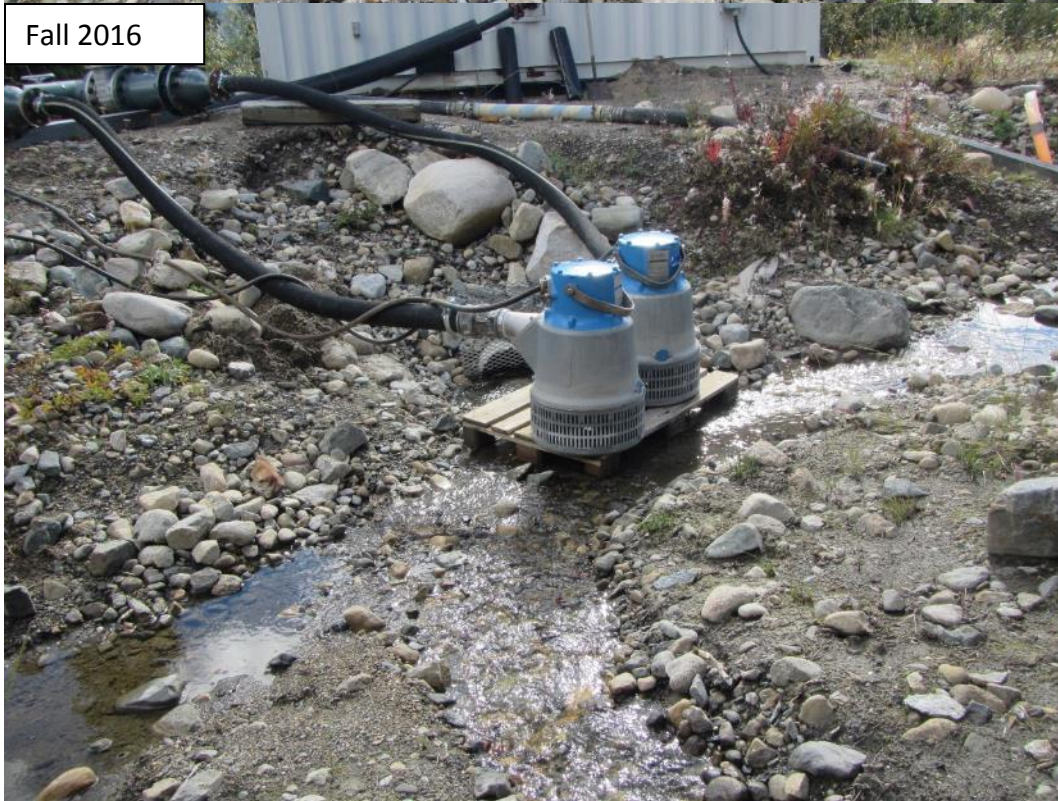
Photograph 63 V-15 ditch and pumps, water pumped out before reaching Moose Pond
