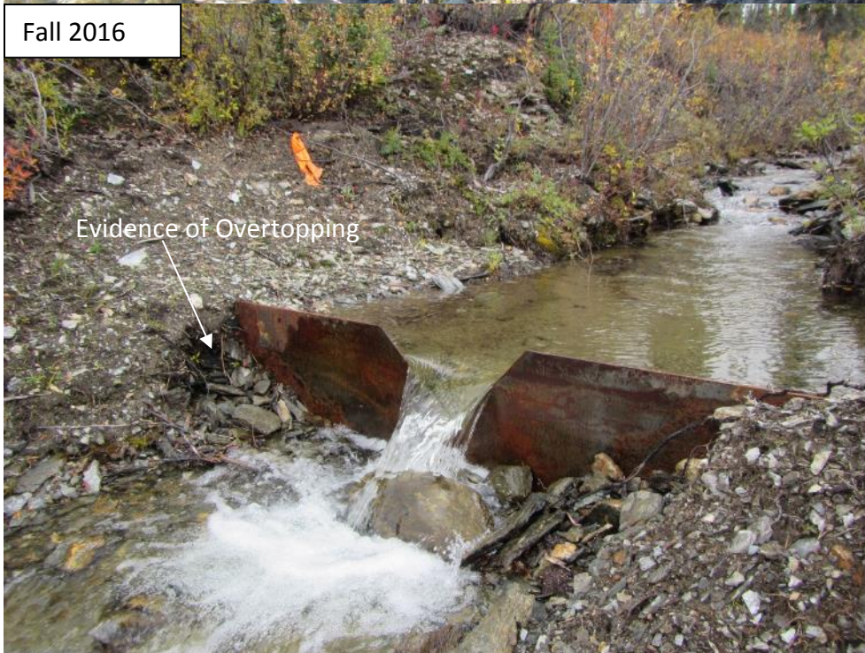
Photograph 6 Interceptor Ditch upstream of upper man-made reach at new weir location. Evidence of overtopping on right abutment.
