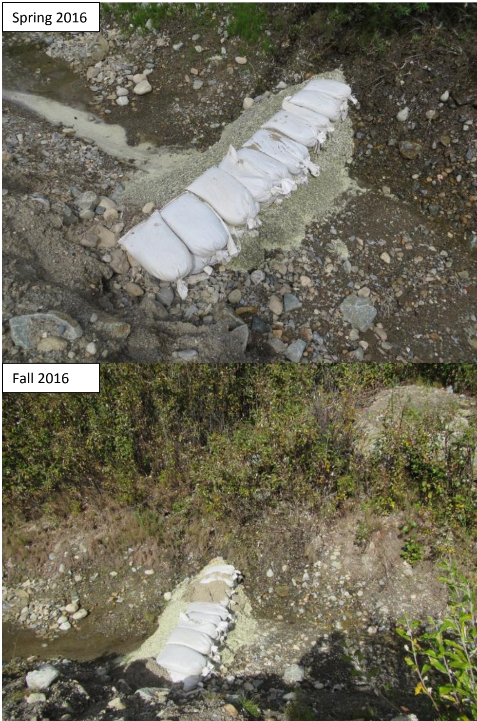
Photograph 62 Sand bags and bentonite are blocking most of the seepage to Moose Pond.
