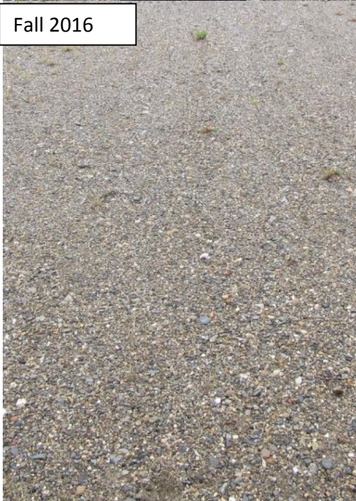
Photograph 30 Freeze-thaw longitudinal cracks closed along dam crest, looking south. Crack is closed (not visible in photo) in fall.
