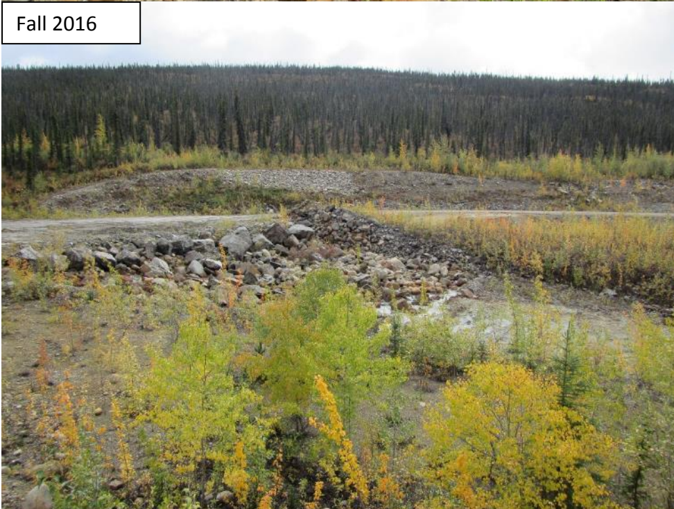
Photograph 24 Fuse plug of Canal Dyke, looking upstream. Vegetation on downstream slope of Secondary Tailings Dam should be removed.
