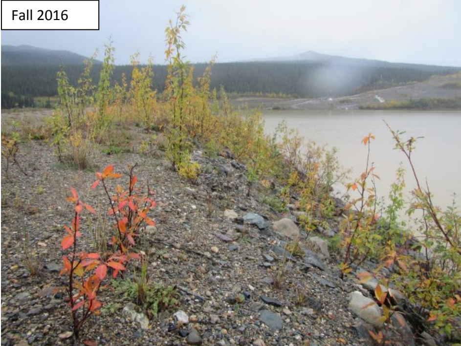
Photograph 31 Upstream slope (looking north), vegetation growth. Trees should be removed.
