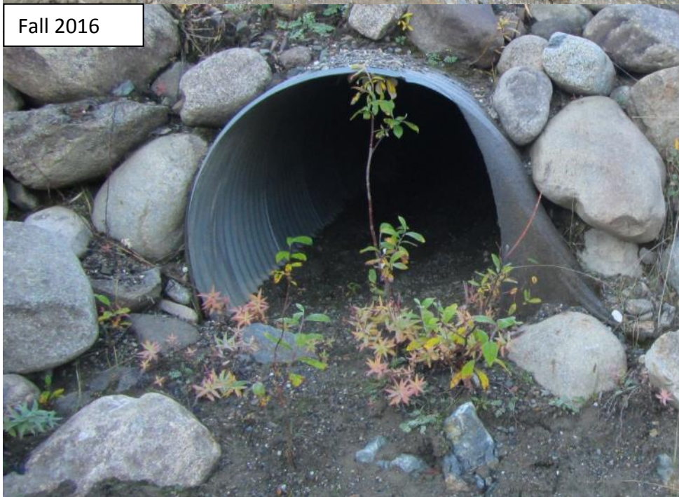
Photograph 46 Flume emergency spillway culvert entrance area (only one culvert shown). Sediment in culvert.
