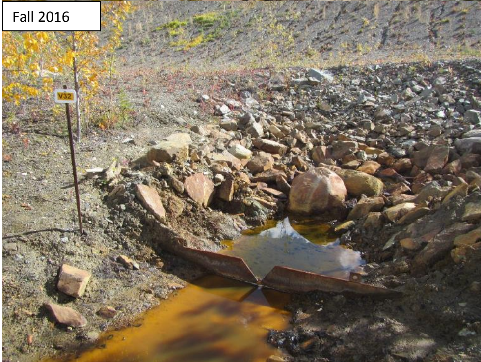
Photograph 39 Drain No. 5 (V32). Pooling downstream of weir. Pond should be cleaned out so it doesn't backwater the weir.
