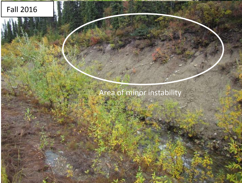
Photograph 5 Vegetation and Slumping on the Faro Creek Diversion Ditch (Upstream of the FCD-4 Stream Gauge Station)
