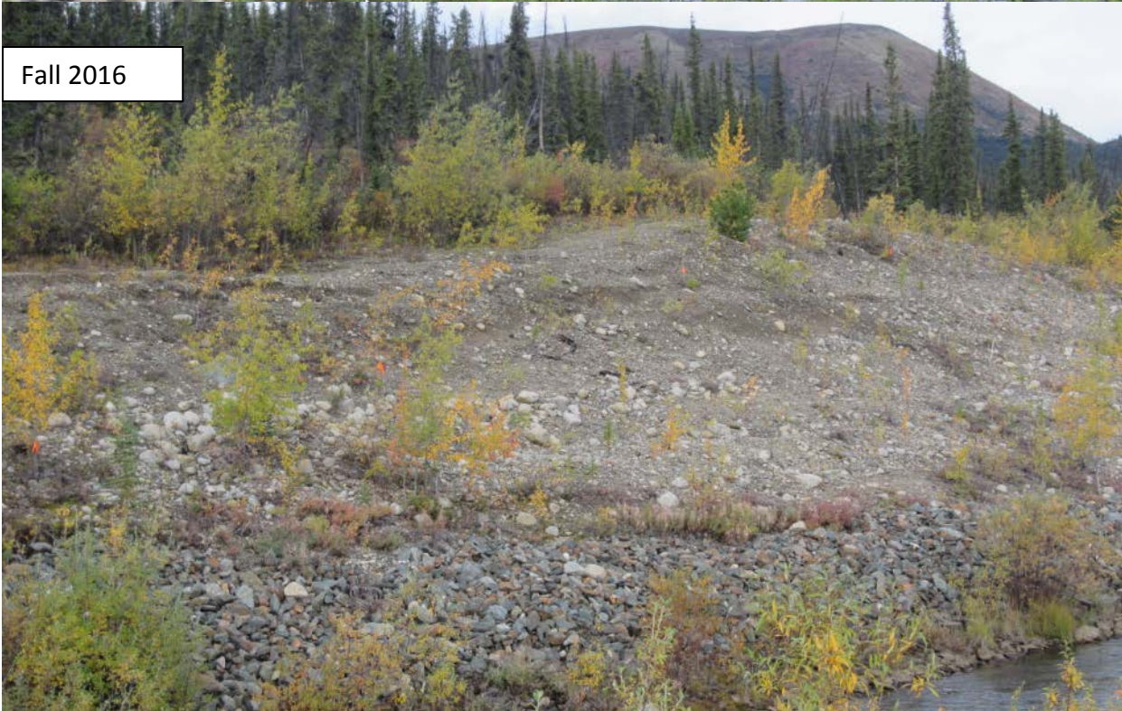
Photograph 13 Rose Creek Diversion Channel back-slope slumping. Similar conditions in spring and fall.
