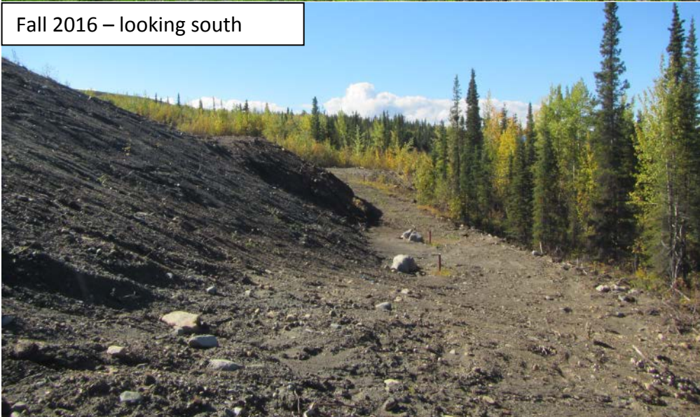
Photograph 55 Little Creek Dam downstream toe. Vegetation has been removed since spring. Slope is subject to erosion and should be repaired and stabilized.
