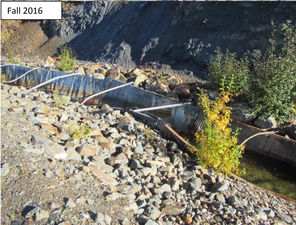
Photograph 50 Damaged flume, flat slope, and constricted channel
