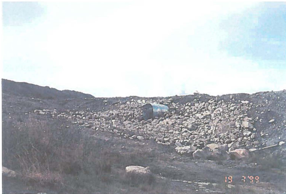
Photo 16: View of the inlet to the culvert after more rip rap was placed
