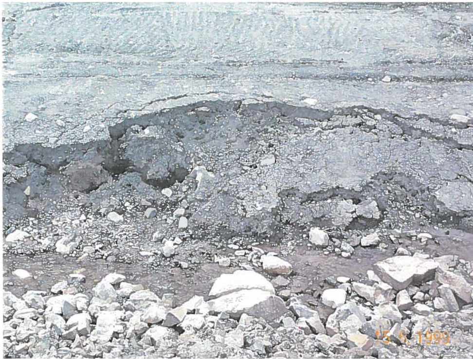
Photo 29: Erosion in GID Sideslopes below Treatment Plant
