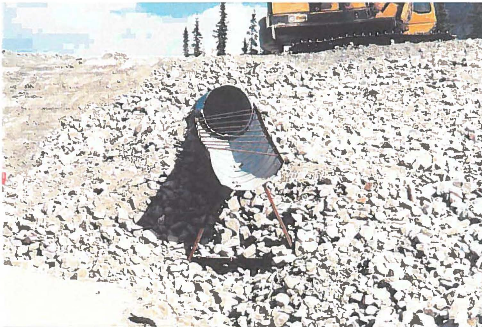
Photo 20: outlet of LCD culvert with Flume attached, September 1999
