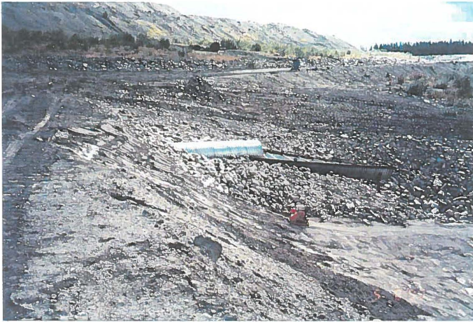
Photo 19: View of the Culvert outlet with additional riprap and the attached half-round flume, September 1999
