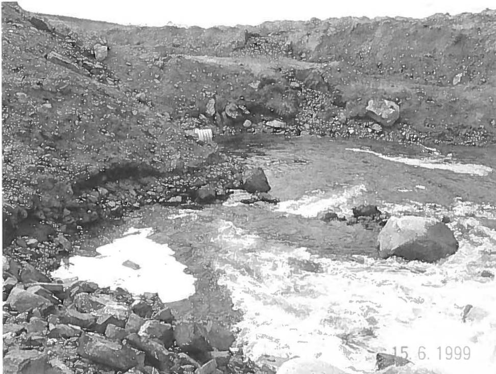
Photo 25: Erosion of the Sideslopes at the Stilling Basin below the Vangorda Creek Diversion
