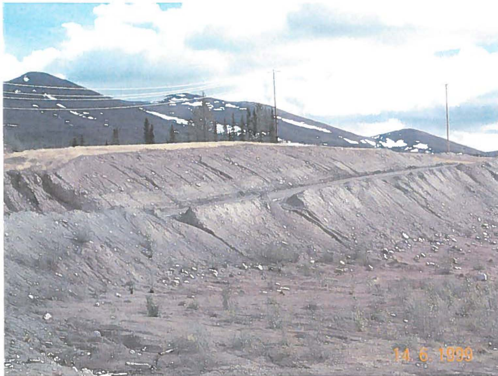
Photo 13: Erosion Gullies in Approach Road to Little Creek Dam
