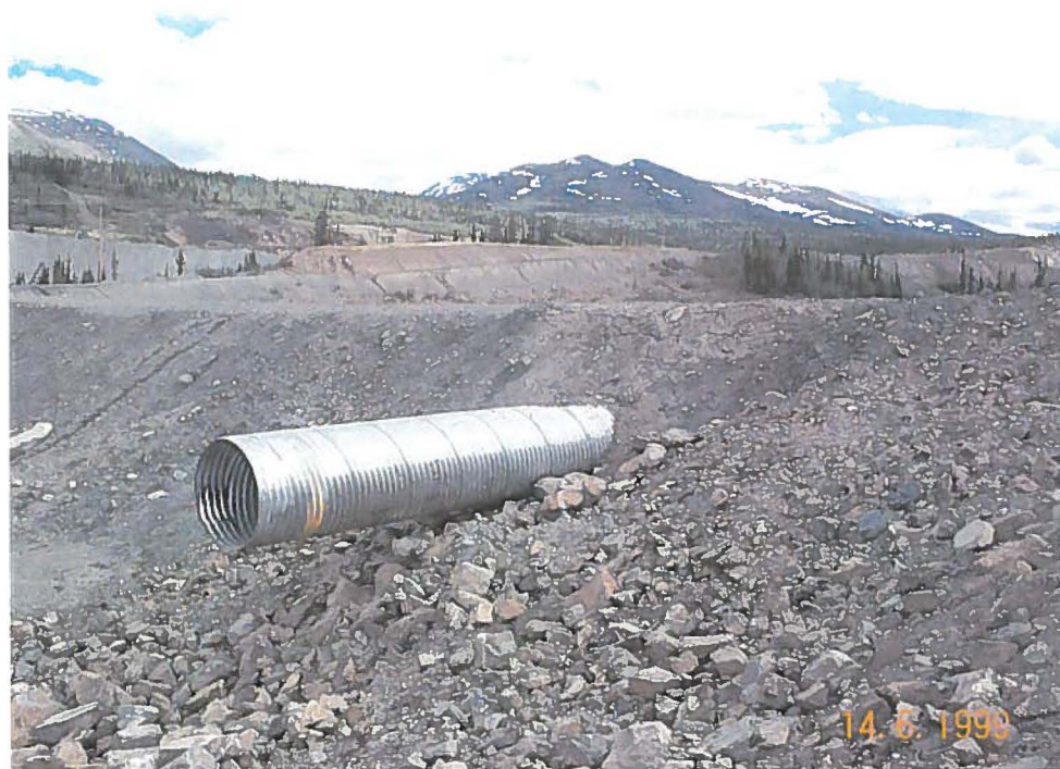
Photo 18: View North of Outlet end of Culvert Spillway at Little Creek Dam
