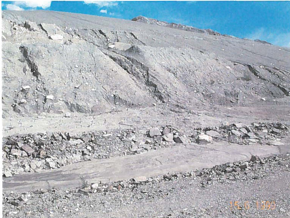
Photo 21: Erosion Gullies in till Berm below resloped areas of Vangorda Waste Dump
