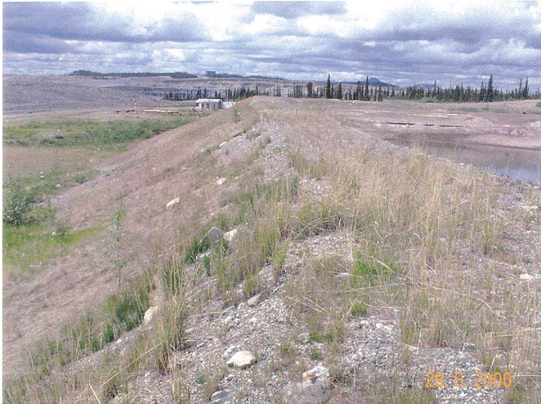
Photo 25 Vegetation on downstream face of Sludge Pond Dyke.
