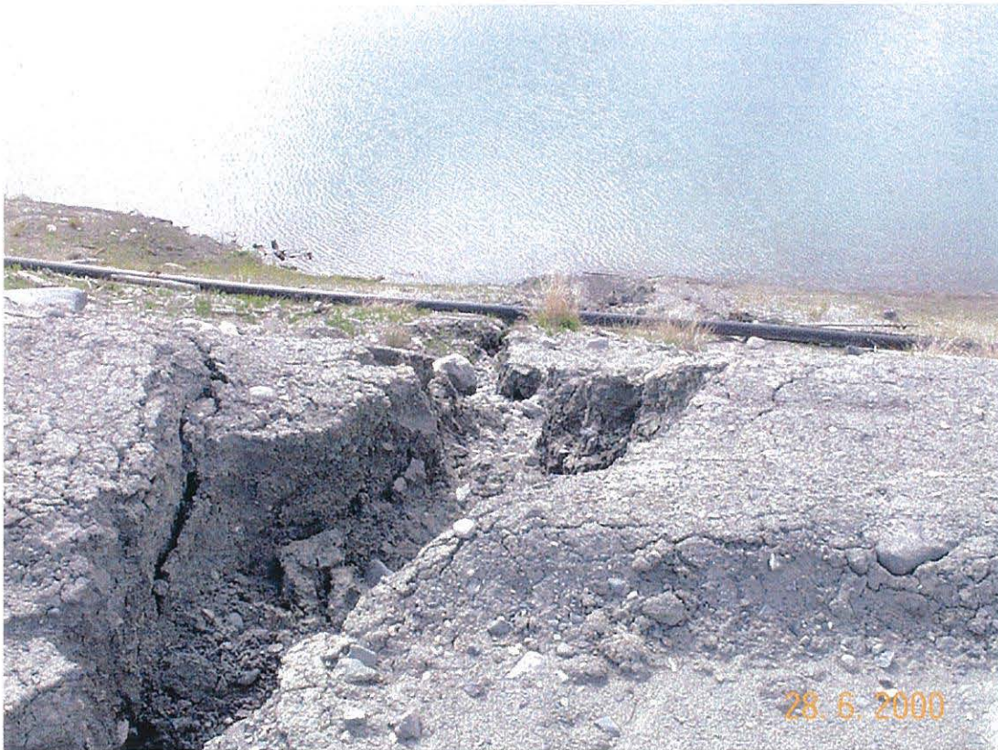
Photo13 Erosion Gully on the upstream face of Little Creek Dam
