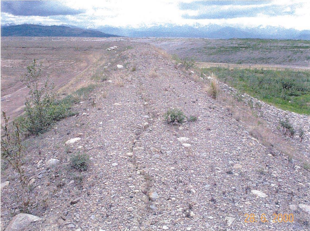
Photo 24 Tension Crack in crest of the Sludge Pond Dyke
