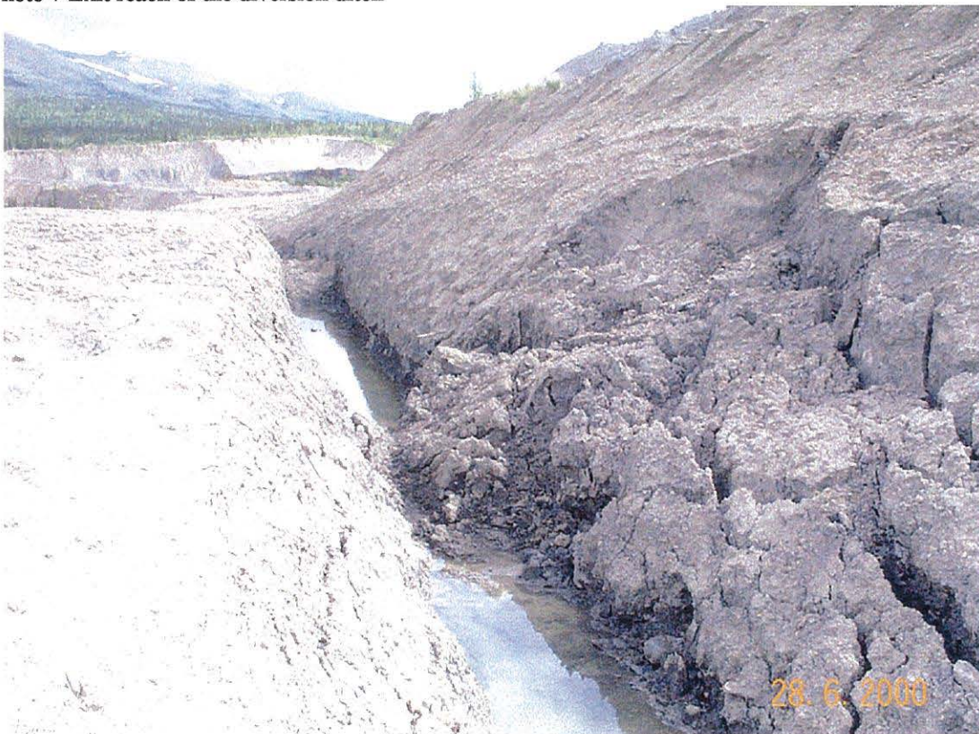
Photo 8 Subsidence in the Diversion ditch
