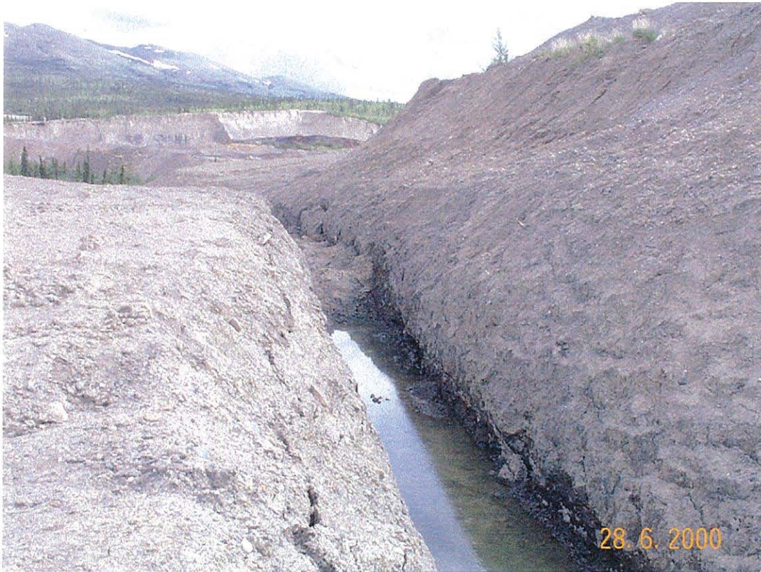
Photo 9 Poned Water in the diversion ditch
