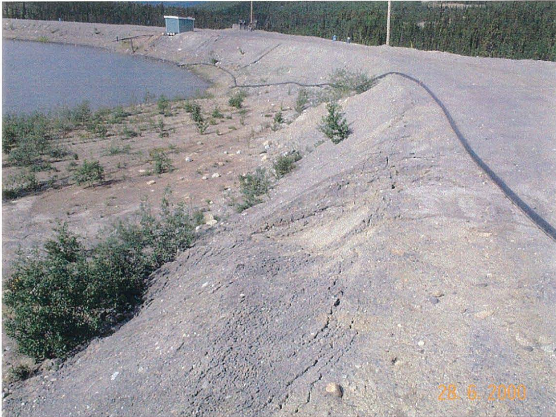
Photo11 Bank Erosion on east approach road
