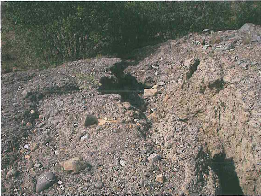
Photo 11: Erosion gully in approach road to Little Creek Dam
