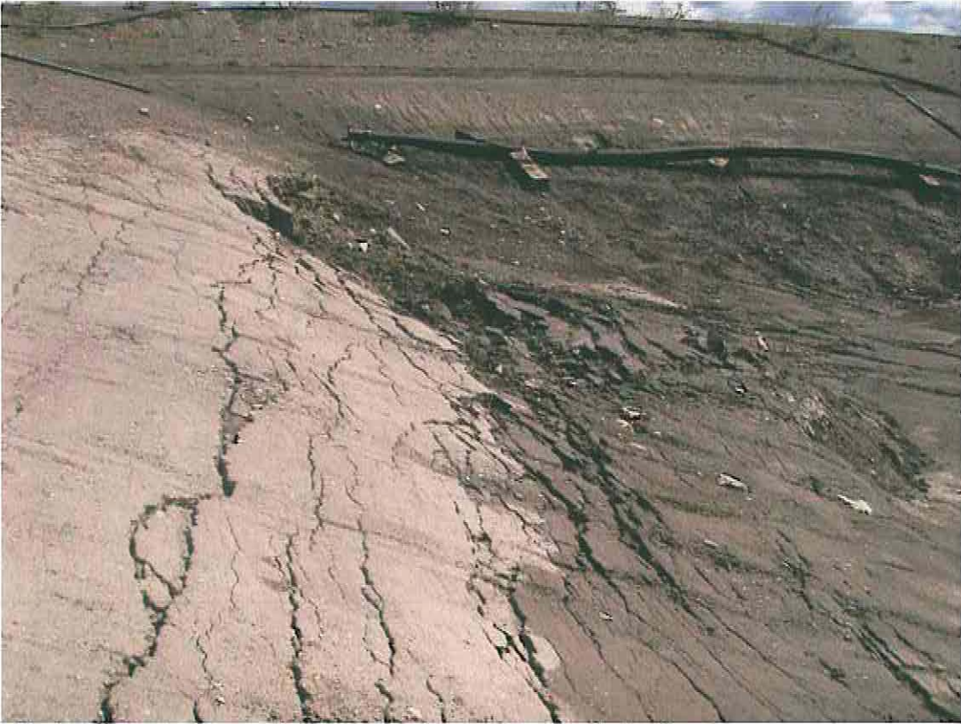
Photo 19: Instability on the upstream slope inside the Sludge Pond
