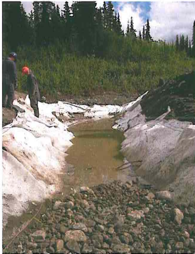
Photo 27: Runoff diversion ditch along haul road during construction showing the Bentamat Liner and course granular cover
