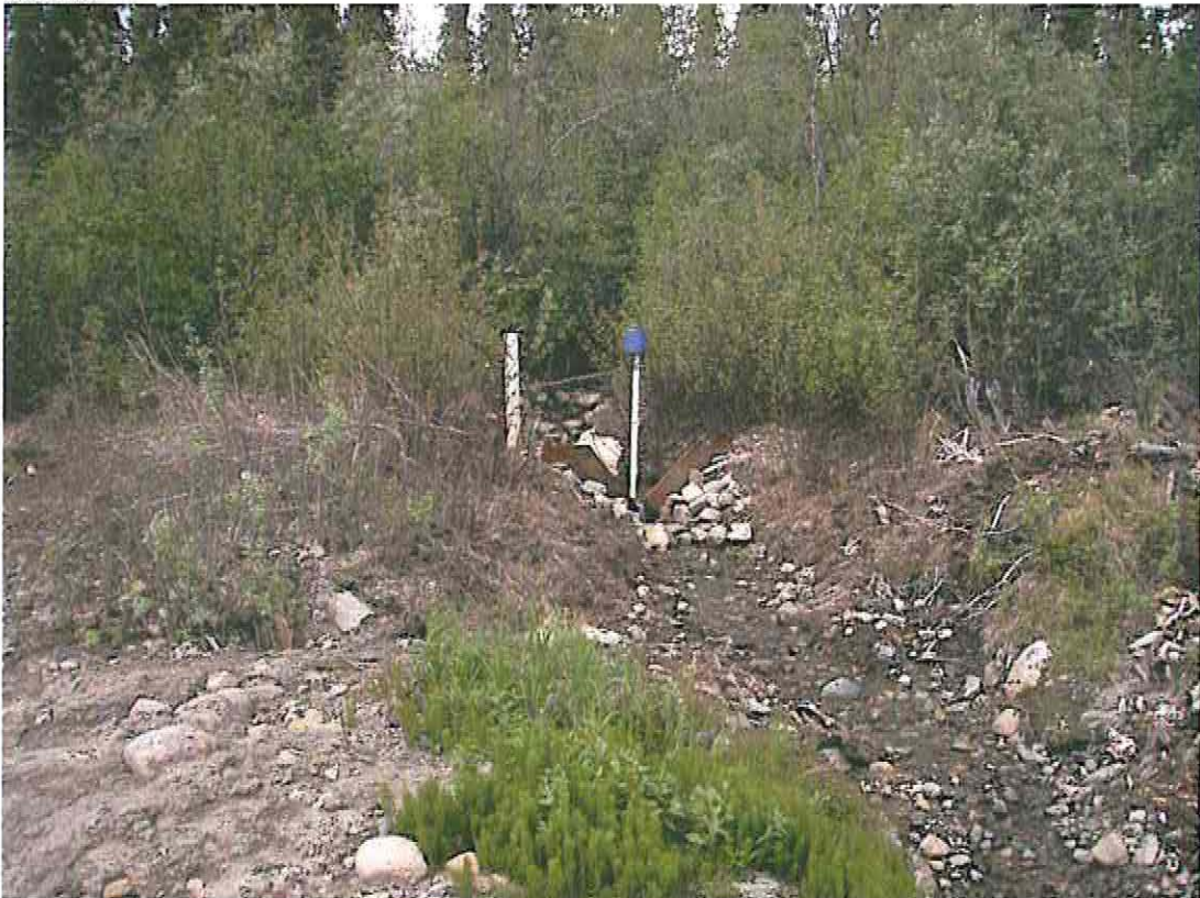
Photo 2: V-notch weir on Grum Creek.
