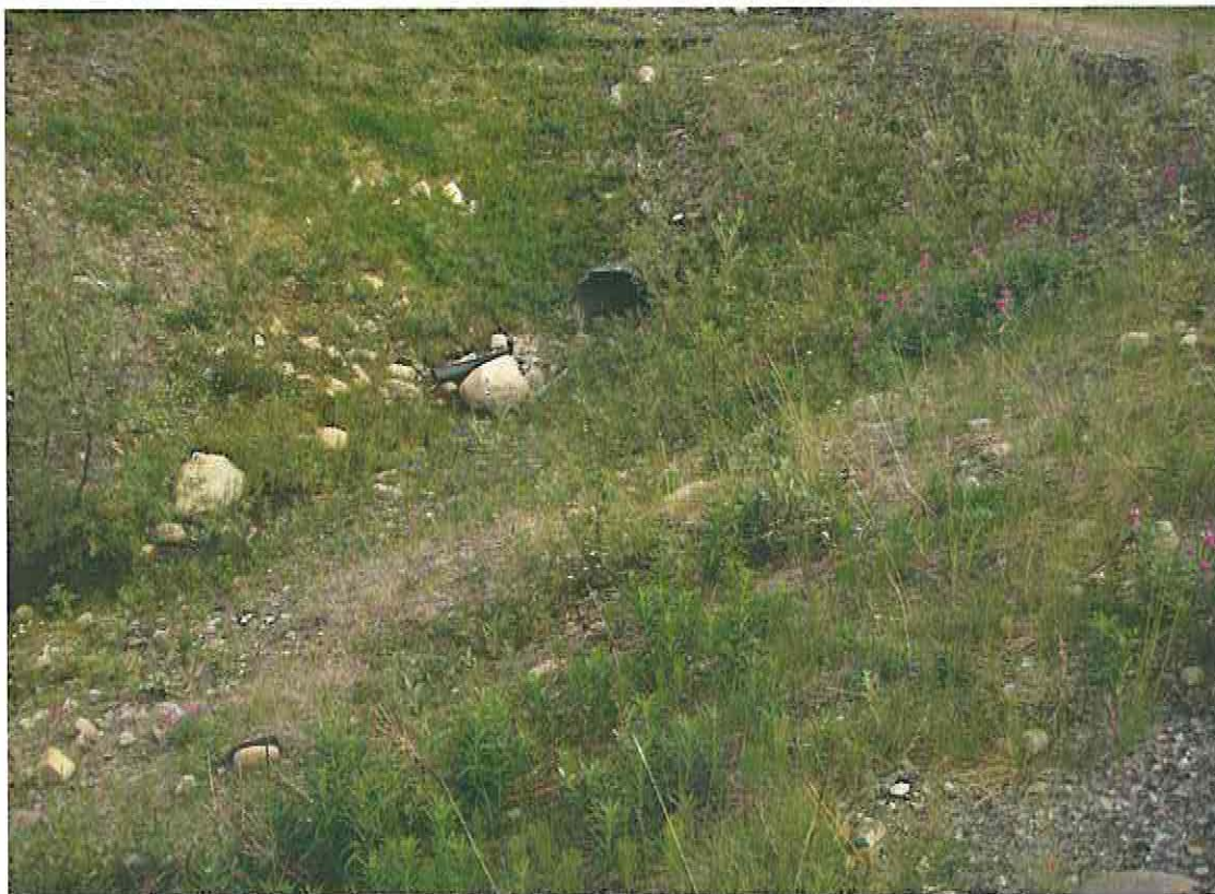
Photo 21: Debris accumulation at culvert entrances along Grum Interceptor Ditch
