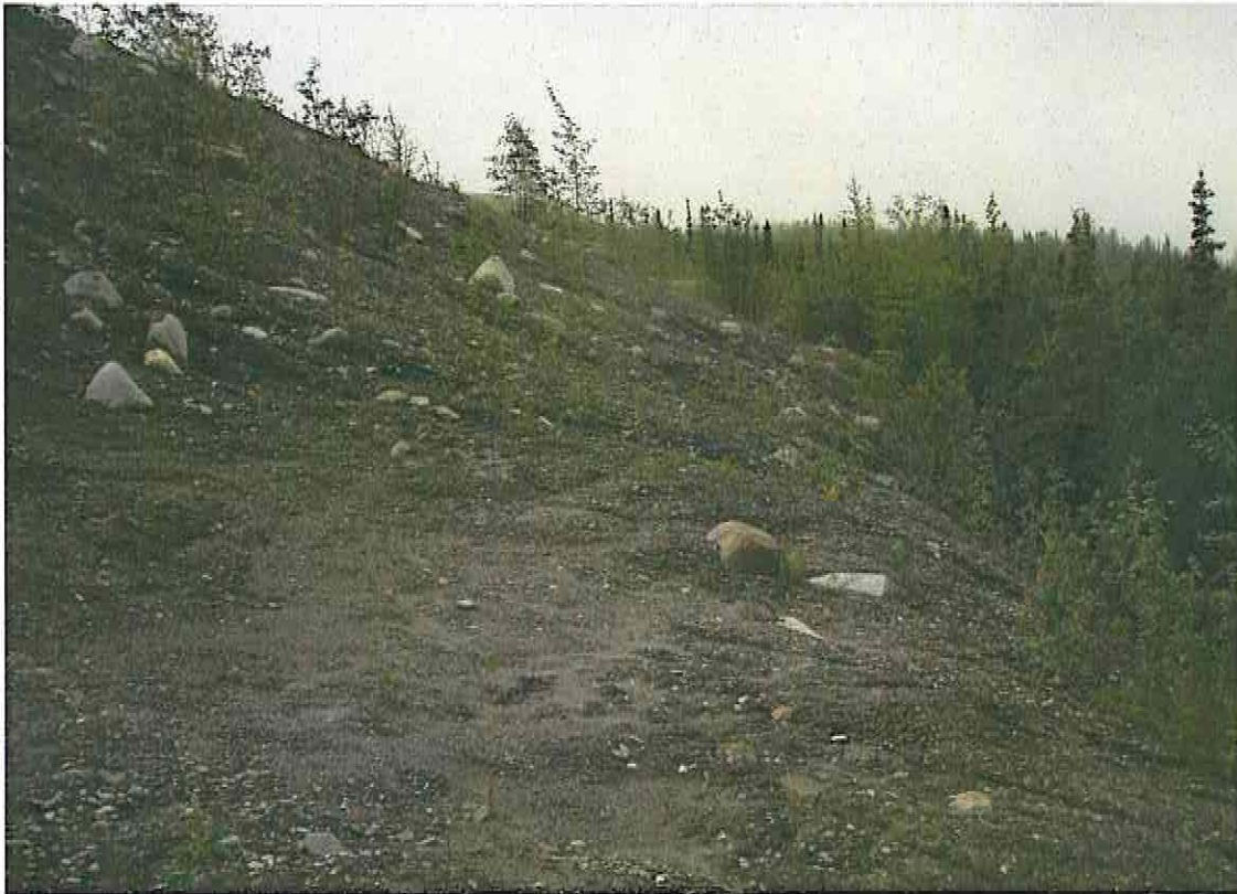
Photo 11: Erosion gullies on downstream slope of LCD
