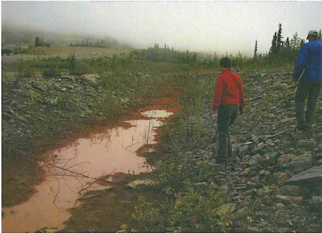
Photo 5: Seepage Collection Channel along toe of Vangorda Waste Dump
