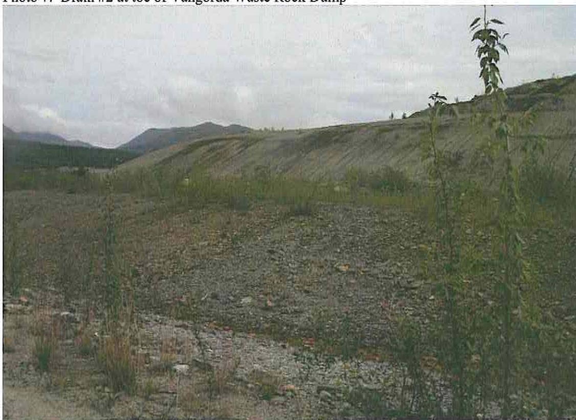
Photo 8: Wetspots and a shallow subsidence on the resloped surface of the Till Starter Dyke at the Vangorda Waste Dump
