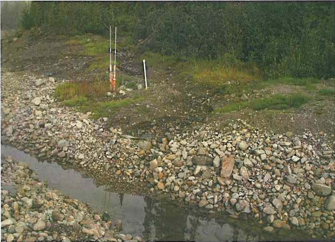
Photo 23: Seepage discharge into V-15 diversion
