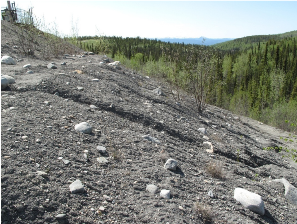
Photo 14: Erosion Gullies on downstream face of Little Creek Dam
