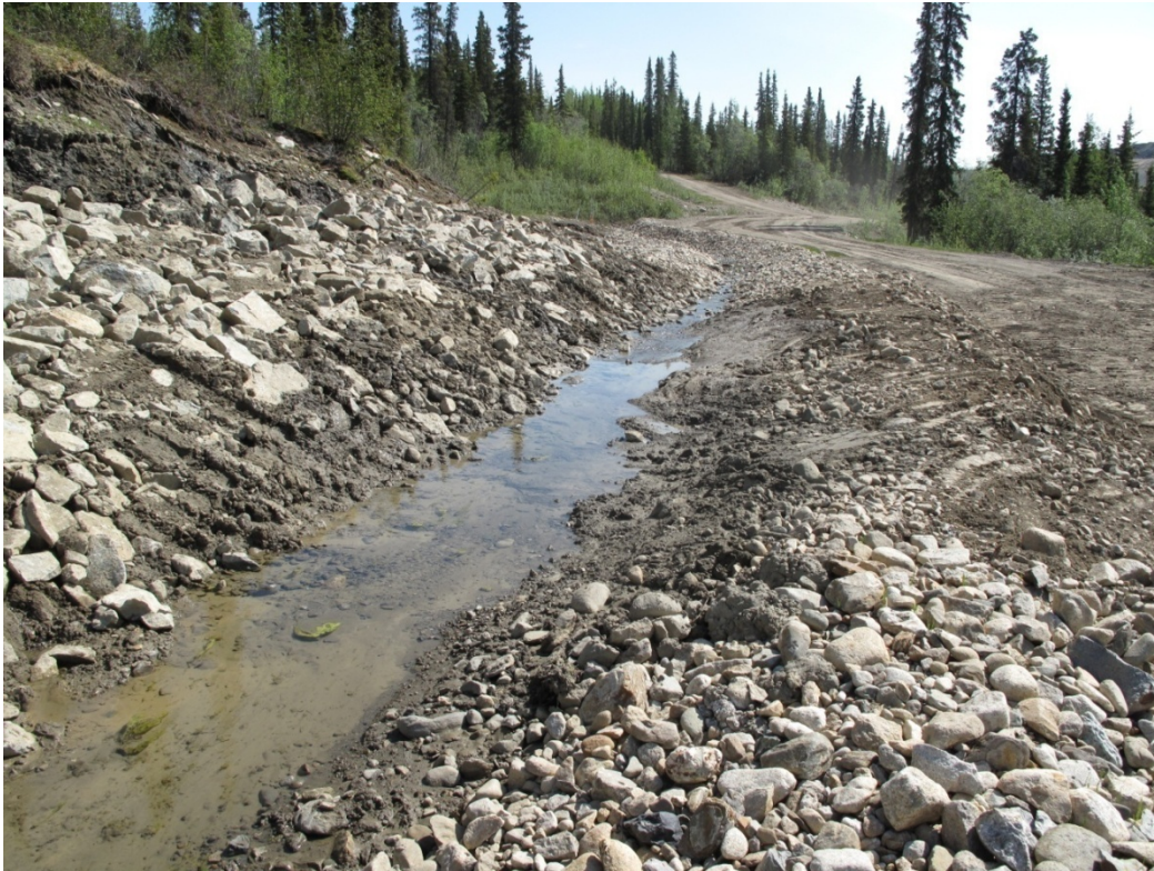
Photo 28: Area of subsidence noted during the 2008 inspection. The slide debris has been removed and the side slope was repaired
