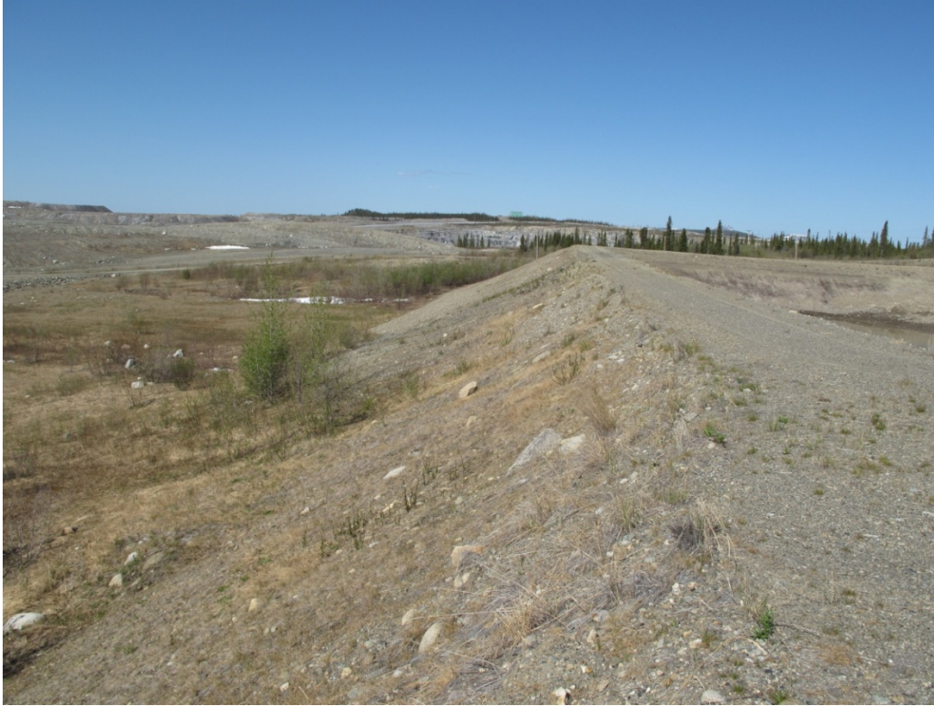
Photo 23: Downstream slopes of Dyke around Sludge Pond at Vangorda Water Treatment Plant
