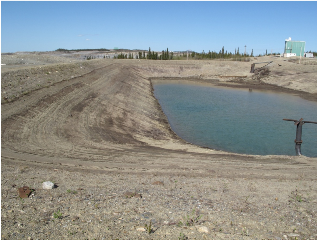
Photo 21: Upstream view of the dyke around the Sludge Pond at Water Treatment Plant
