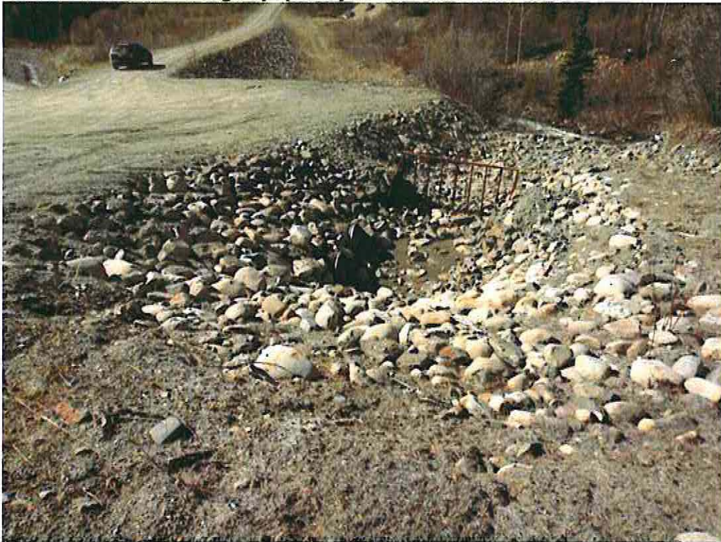
Photo 18: Inlet to emergency spillway at the Headworks of the Vangorda Ck Diversion
