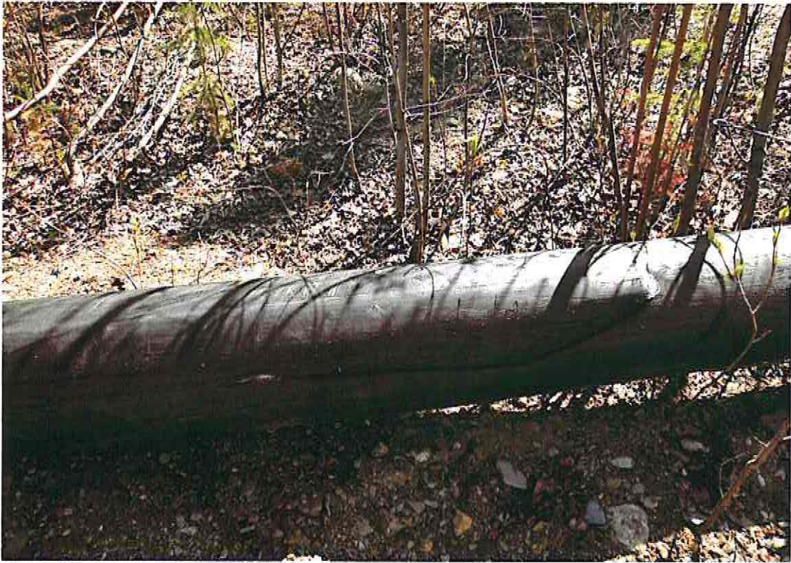
Photo 32: Damage to Siphon Line
