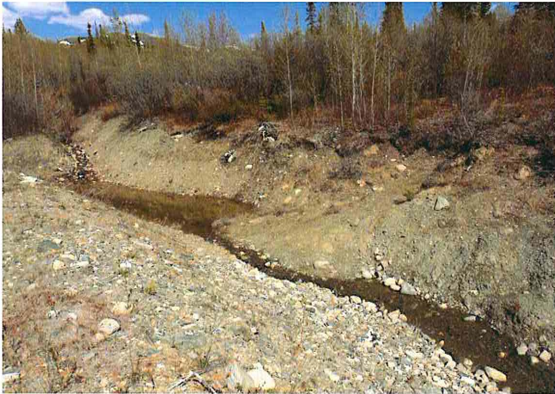
Photo 33: Subsidence in the Surface water runoff diversion ditch above the Vangorda Pit
