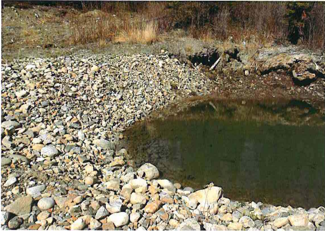
Photo 27: V15 Seepage collection Pond
