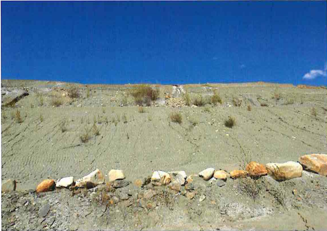
Photo 11: Erosion on the till dyke blow cover trials
