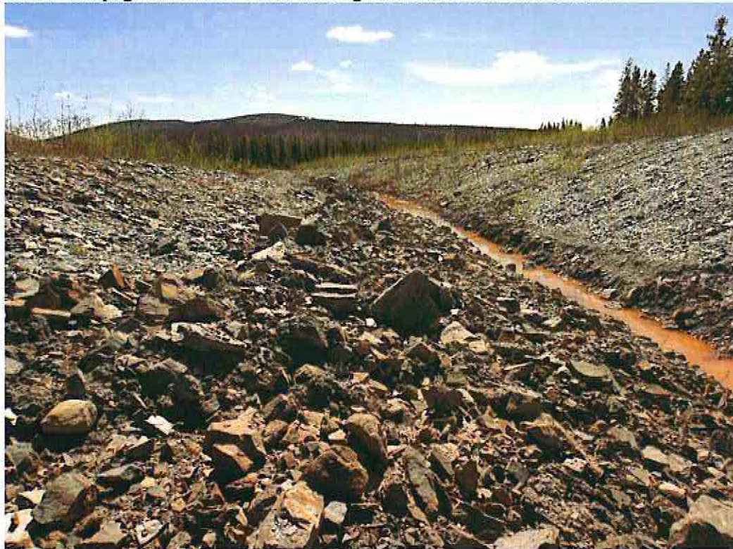
Photo 8: Fall 2009 Excavation of the riprap from the base of the seepage Collection Ditch
