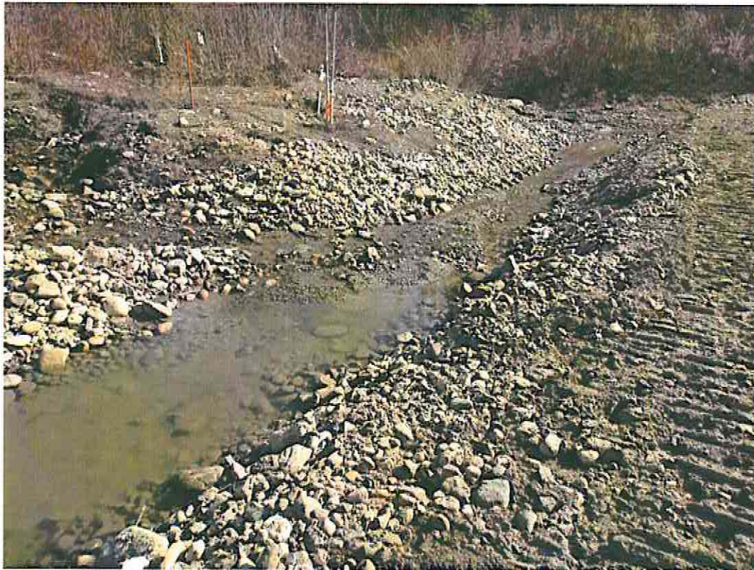
Photo 27: Seepage Collection Ditch Upstream of V-notch Weir in Main Stem of Grum Creek
