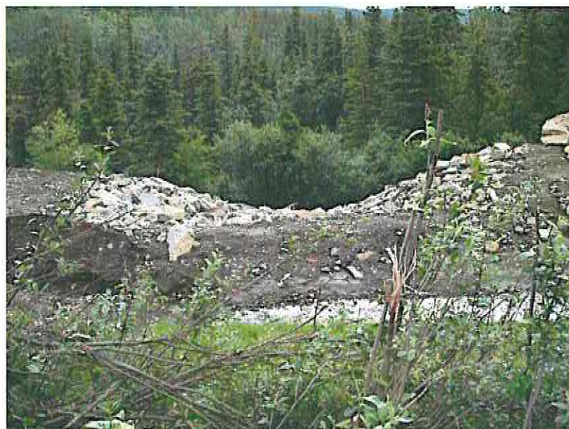
Photo 5: Temporary re-direction off flow blocked off; flow from V15 ditch is directed to Moose Pond (June 26, 2011)
