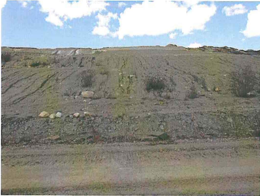
Photo 9: Erosion on the Till Dyke Blow Cover Trials
