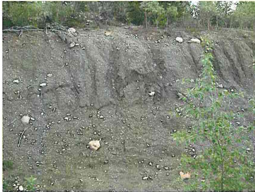
Photo 1: Erosion along Vangorda Interceptor East, upper section (June 26, 2011)
