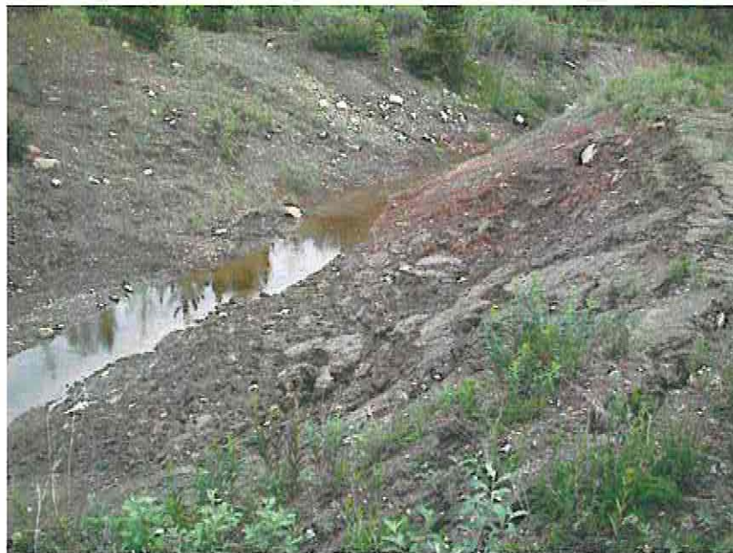
Photo 2: slumping along Vangorda Interceptor East, lower section (June 26, 2011)
