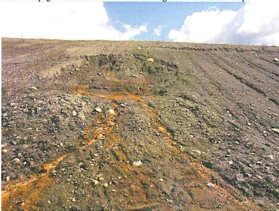
Photo 8: Shallow Subsidence on Till Dyke Above Seepage Collection Ditch
