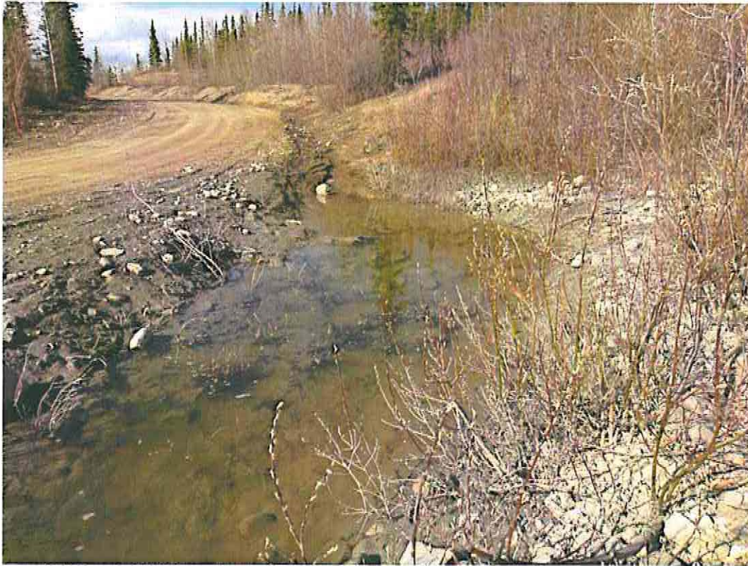
Photo 25 Ponded Water Above Blocked Culvert Below V-15 Pond
