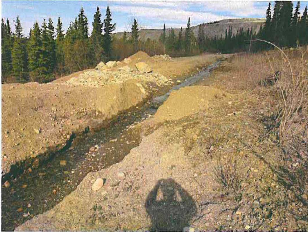
Photo 29: Ditch Above Moose Pond with Riprapped Spillway Installed by DES during High Runoff Event from GSC
