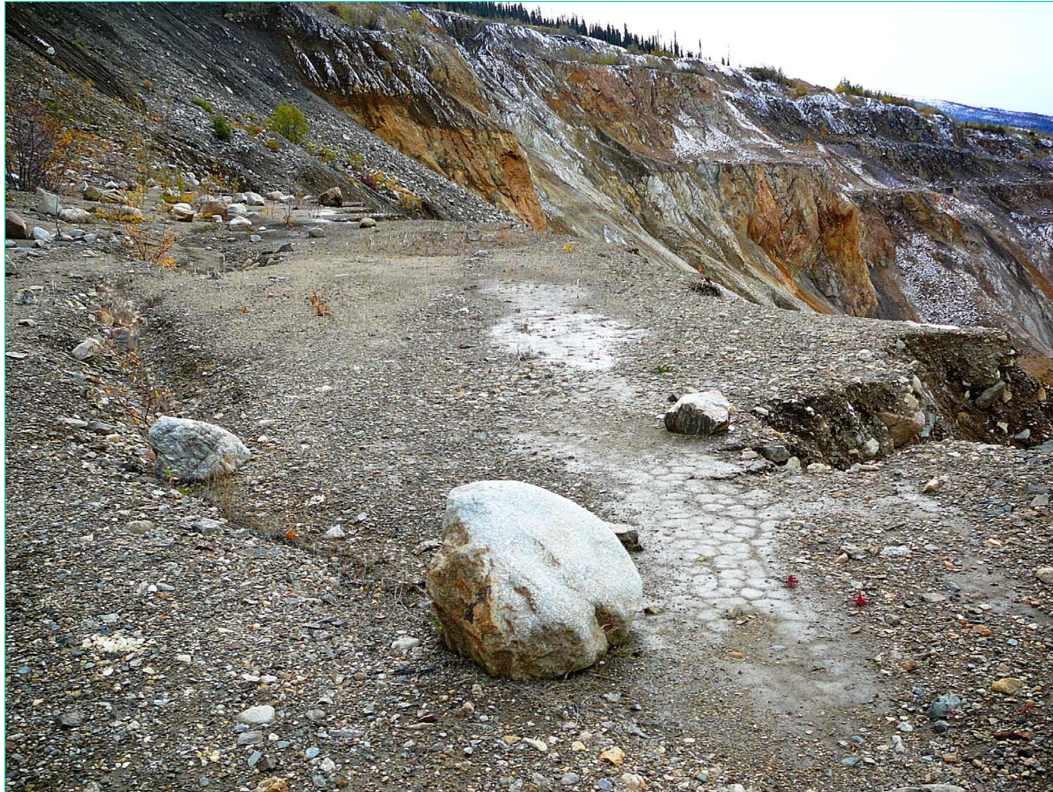
Photograph A-3 Faro Pit – North Instability Zone. Old crack to the north of the instability zone.
