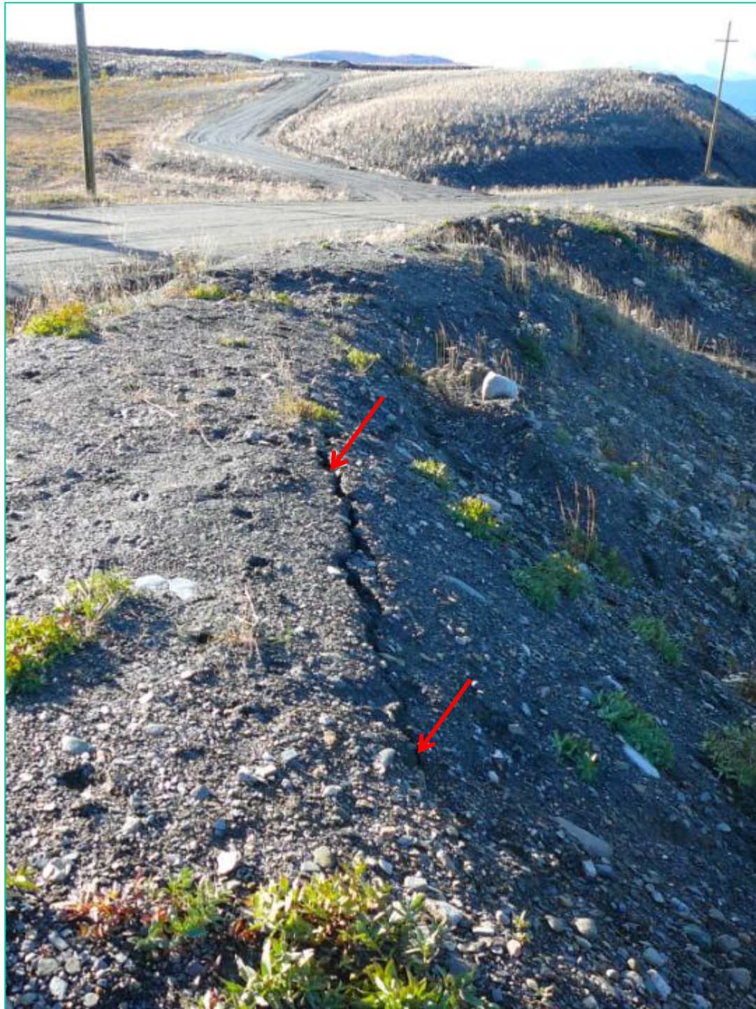
Photograph D-6 Grum Pit recent crack, located to the south of the South Array, near road. View looking southwest.
