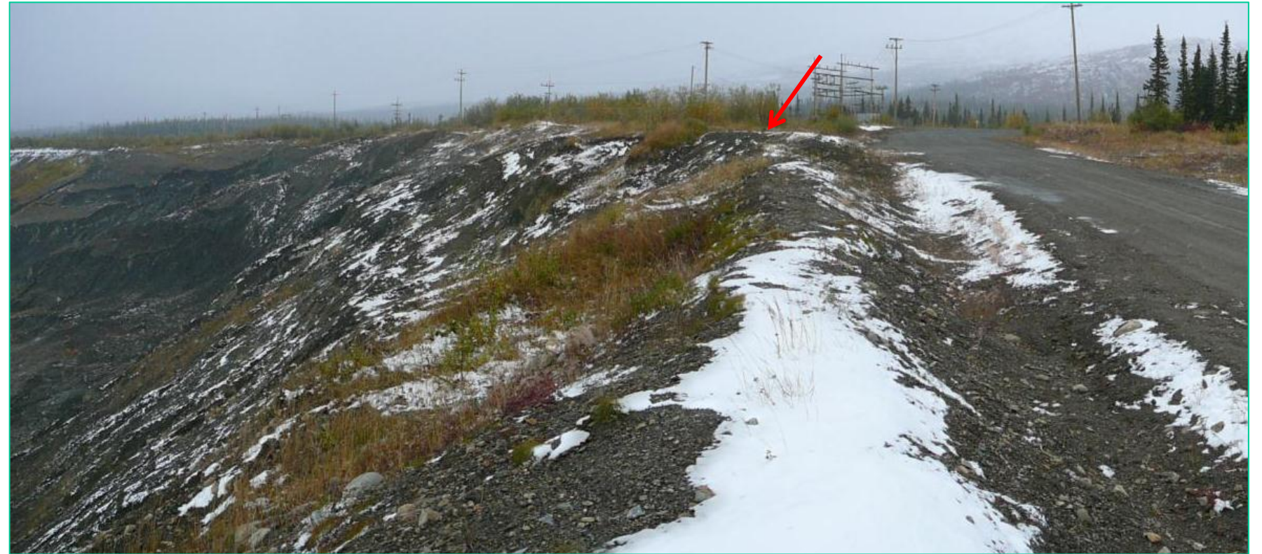
Photograph D-7 Grum Pit recent crack, located to the south of the South Array, near road. Approximate location indicated by red arrow. View looking northeast.
