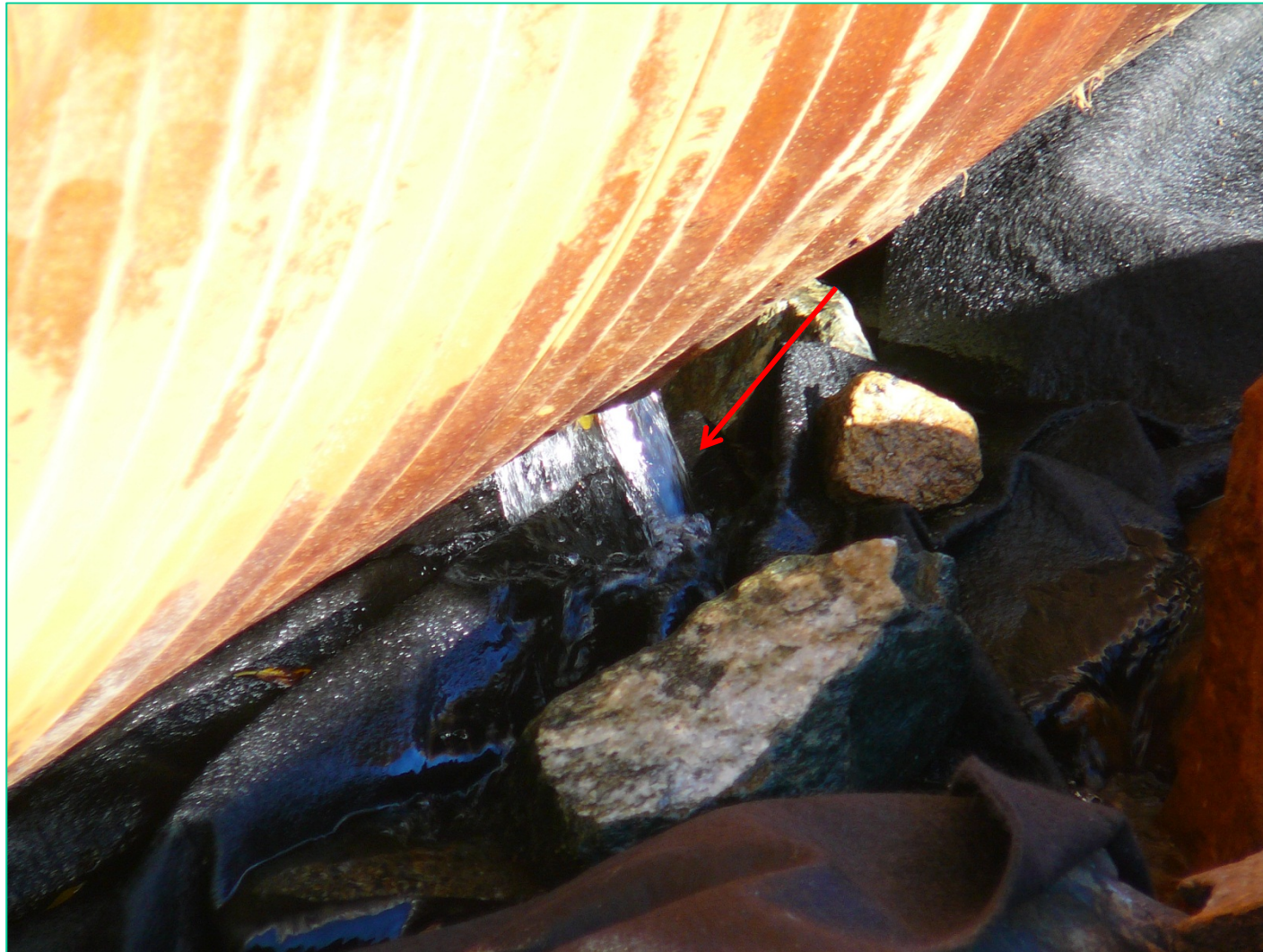
Photograph E-9 Vangorda Pit – Water leaking beneath flume.
