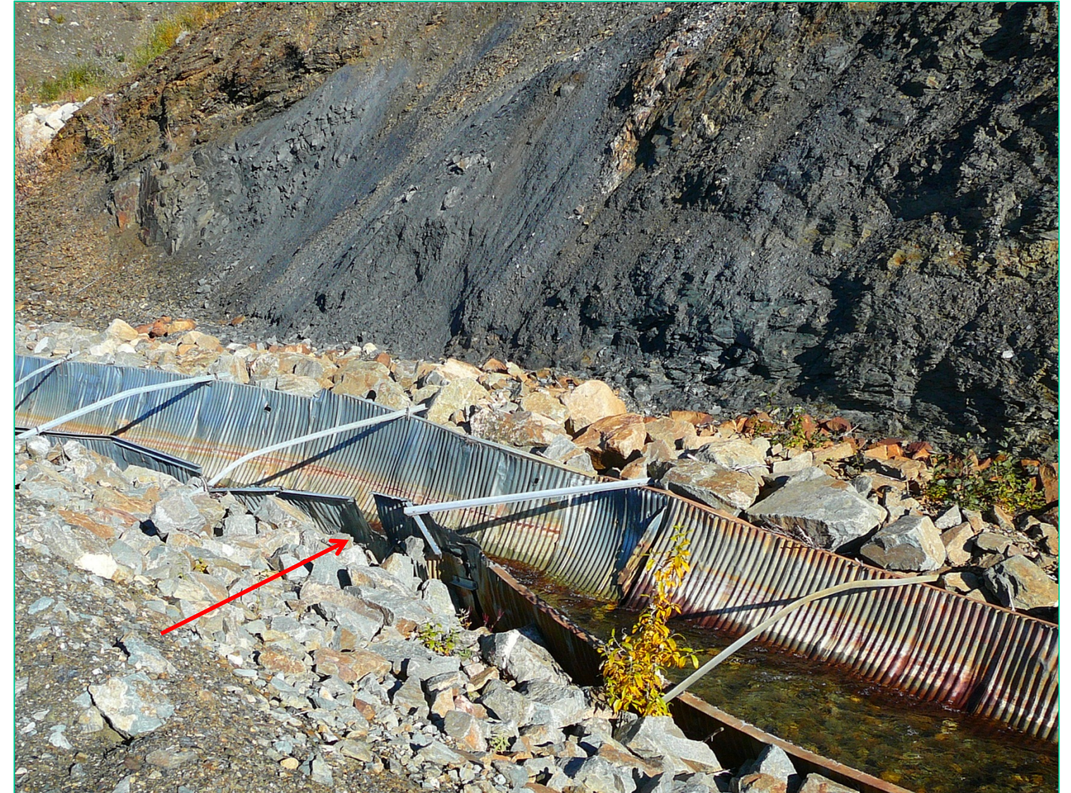
Photograph E-8 Vangorda Pit – Vangorda Creek Diversion Channel. Sections are in disrepair, allowing leaks. View looking north.
