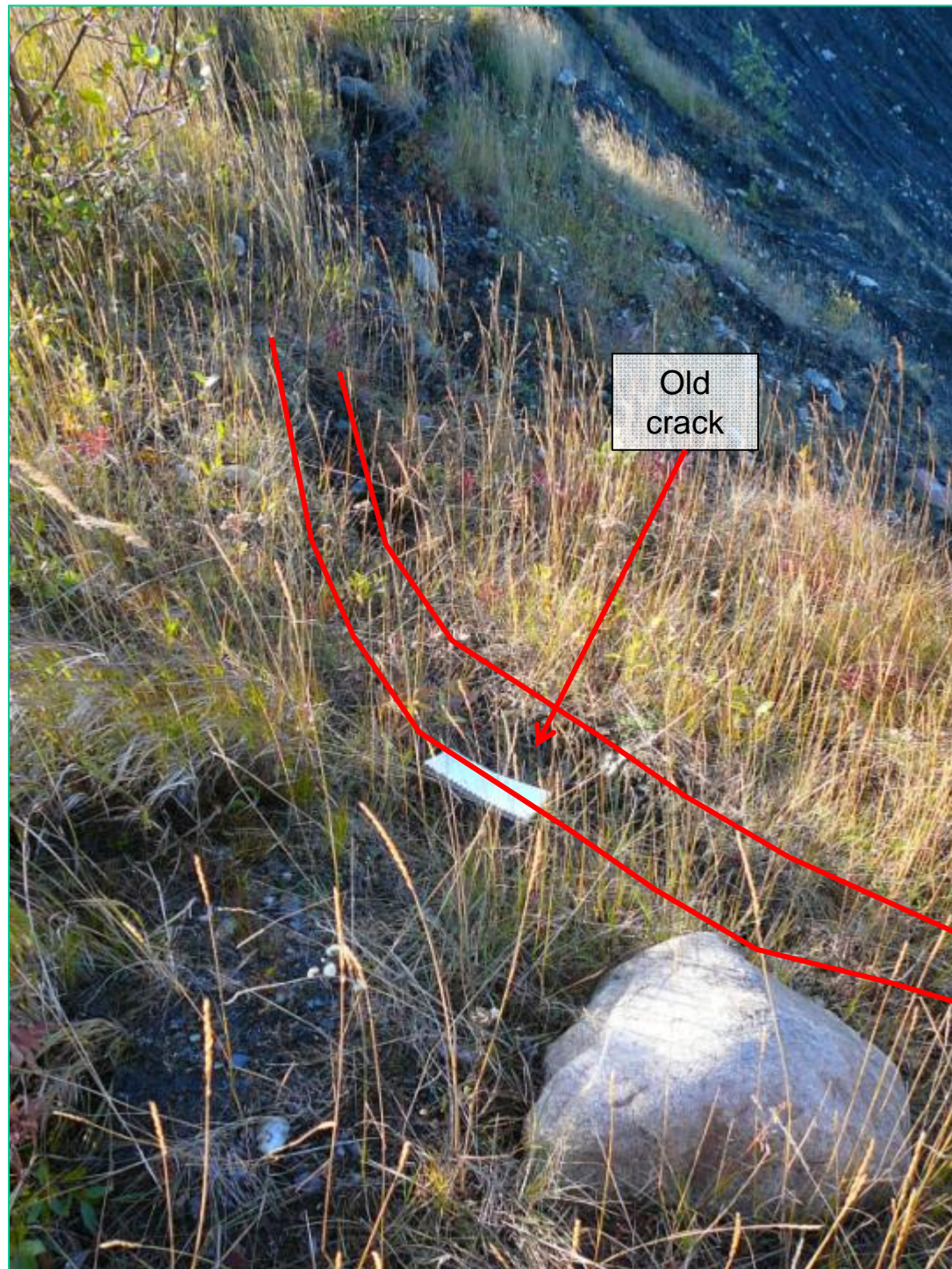
Photograph D-10 Grum Pit old crack, located at crest of east wall, south of the South Array. View looking south.
