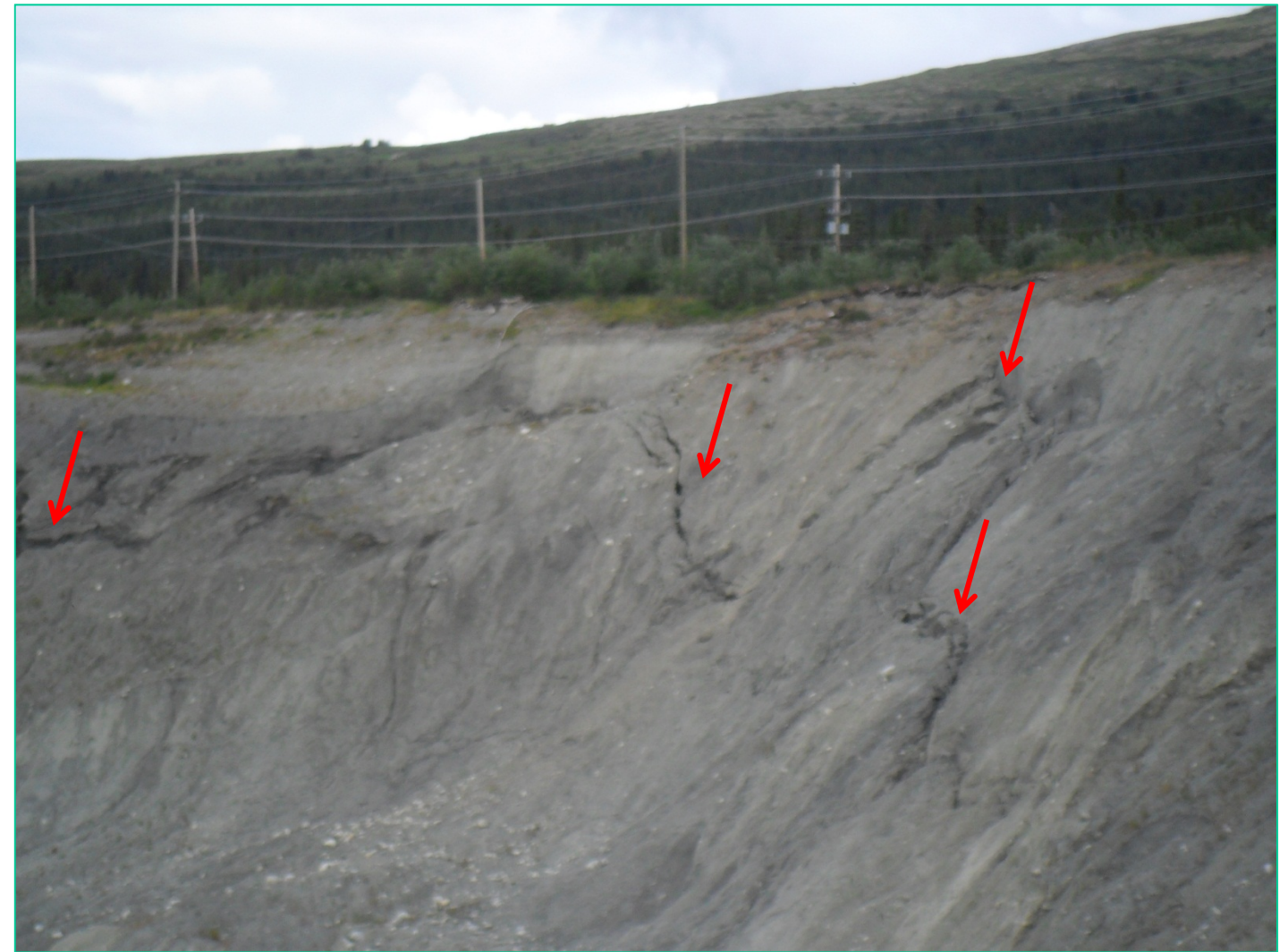
Photograph D-3 Grum Pit Instability Zone – new cracks reported in August 2012. View looking north.
