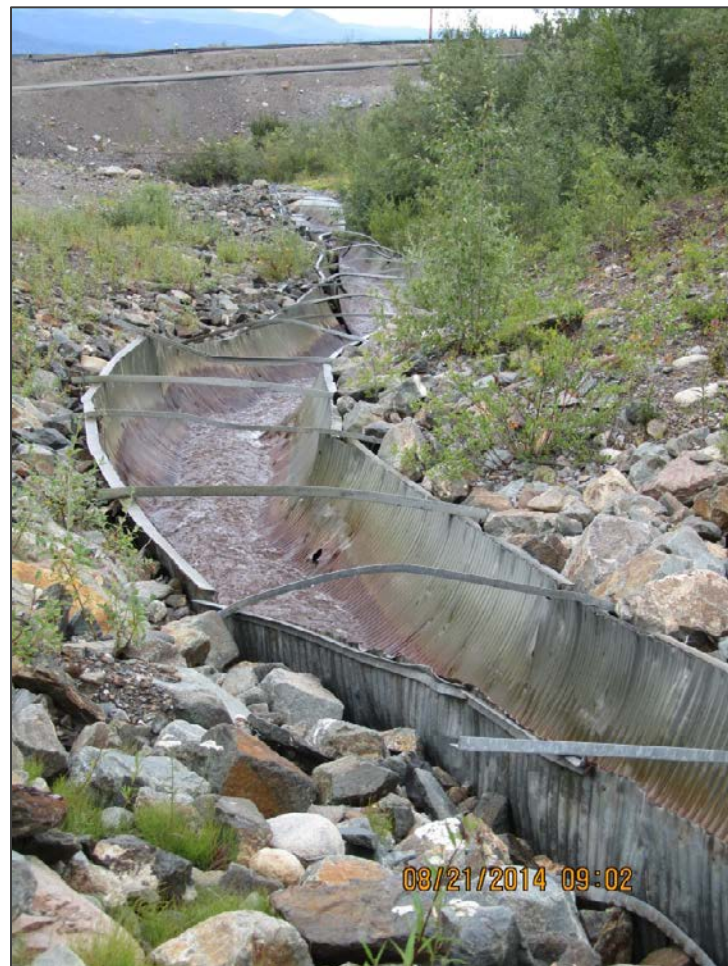
CONDITION OF VANGORDA FLUME
