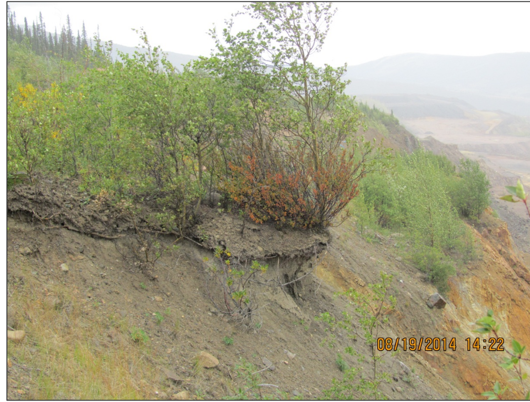
TILL SLOWLY ERODING AND RAVELING
