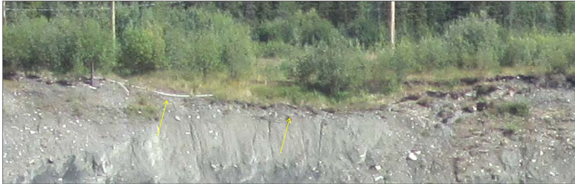
2014 PHOTOGRAPH OF CREST OF EAST WALL, BACKSCARP OF INSTABILITY ZONE, VIEW LOOKING EAST
