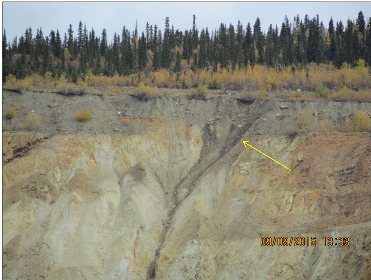
SEEPAGE AT TILL / BEDROCK CONTACT, EAST WALL, VIEW LOOKING EAST
