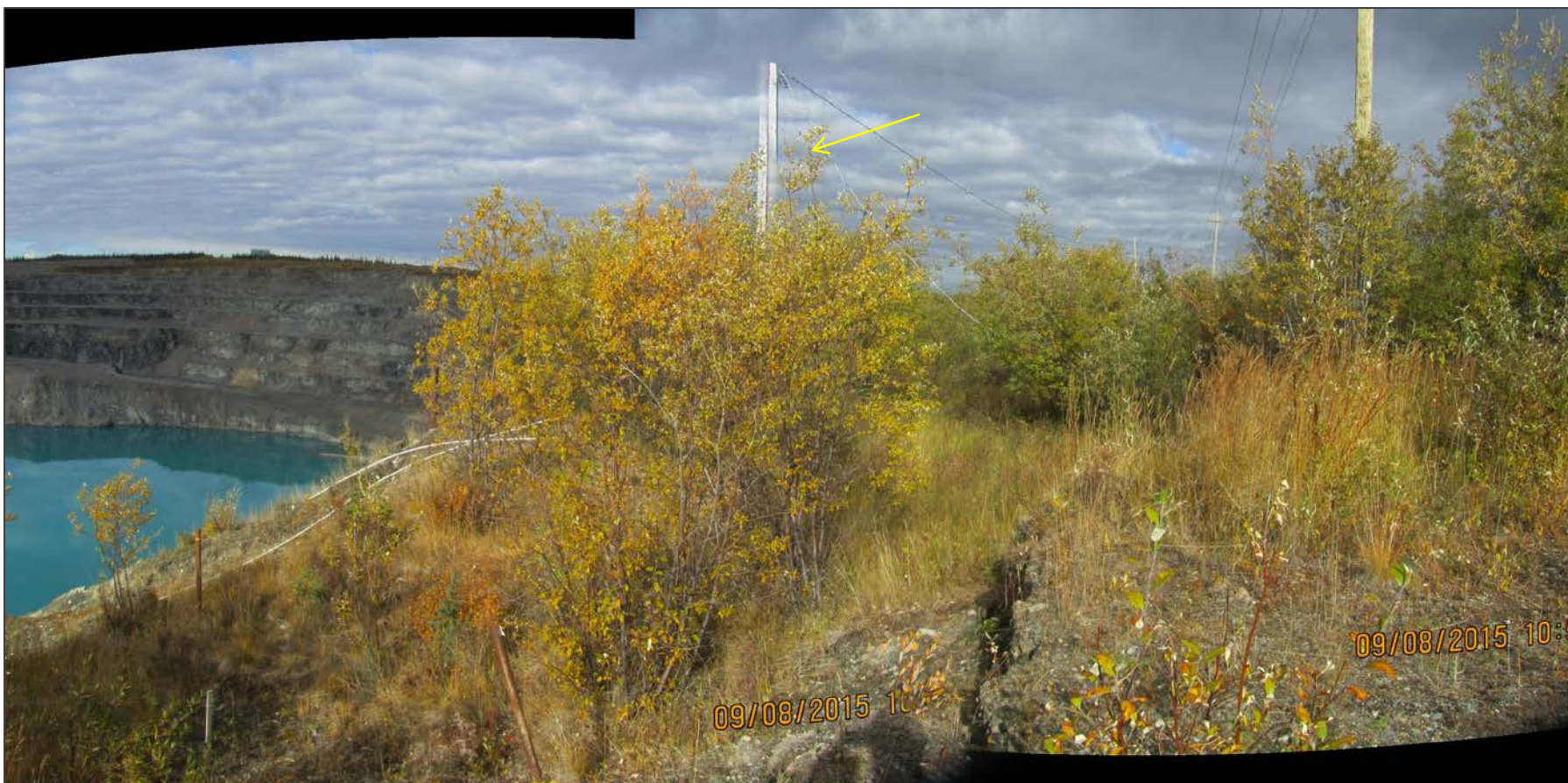
POWER POLE ON DROPPED SIDE OF SLUMP BLOCK, EAST WALL, VIEW LOOKING NORTH
