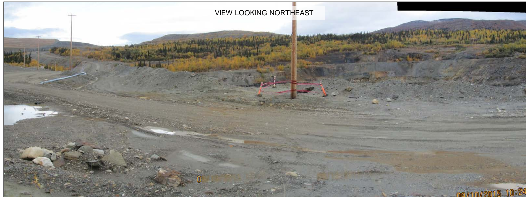
VIEWS OF SINKHOLE IN WEST WALL, TAKEN FROM THE SOUTH SIDE OF THE WALL AT THE CREST
