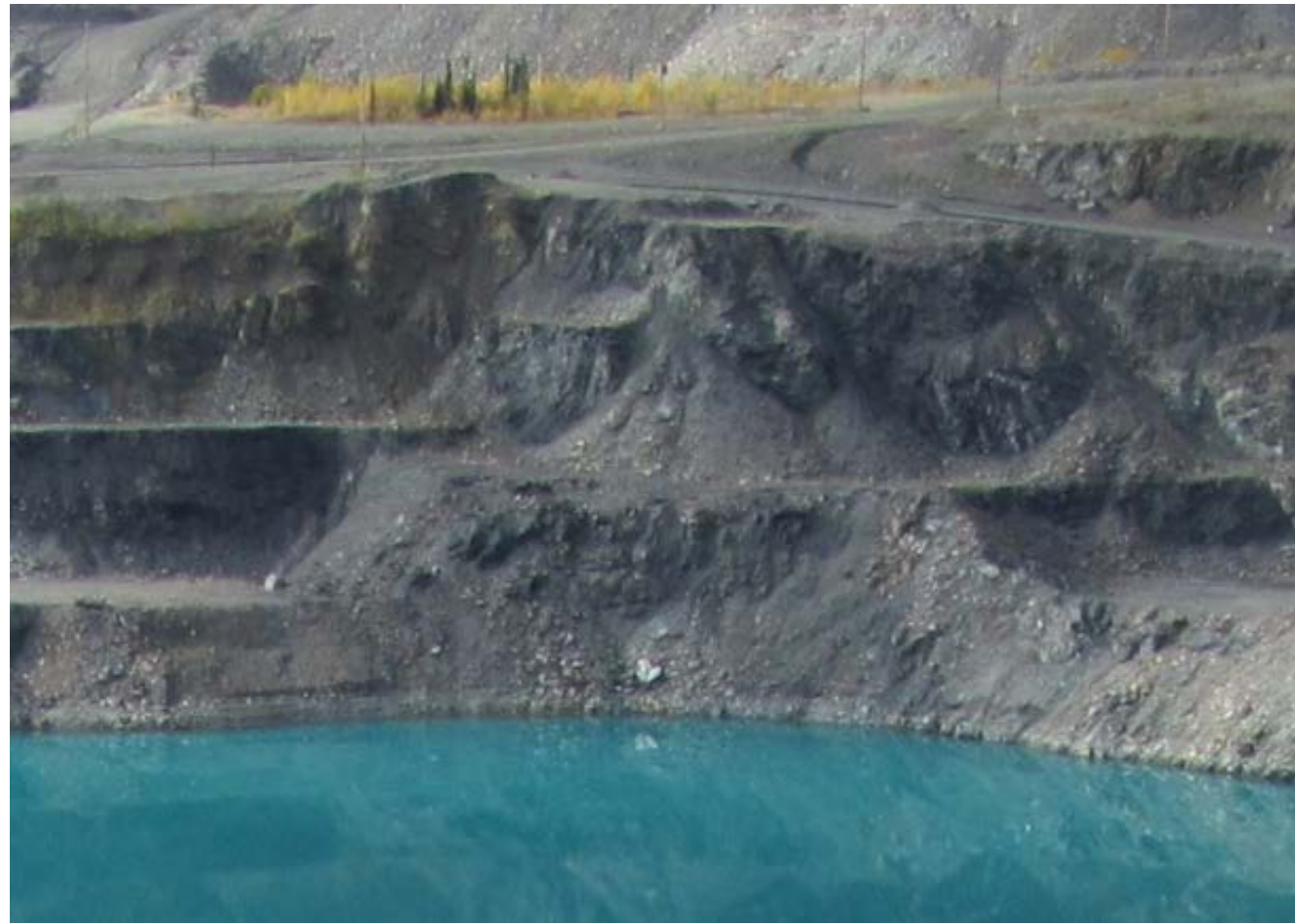
2015 PHOTOGRAPH OF ROCK SLOPE IN SOUTHWEST CORNER OF GRUM PIT. VIEW LOOKING SOUTHWEST.
