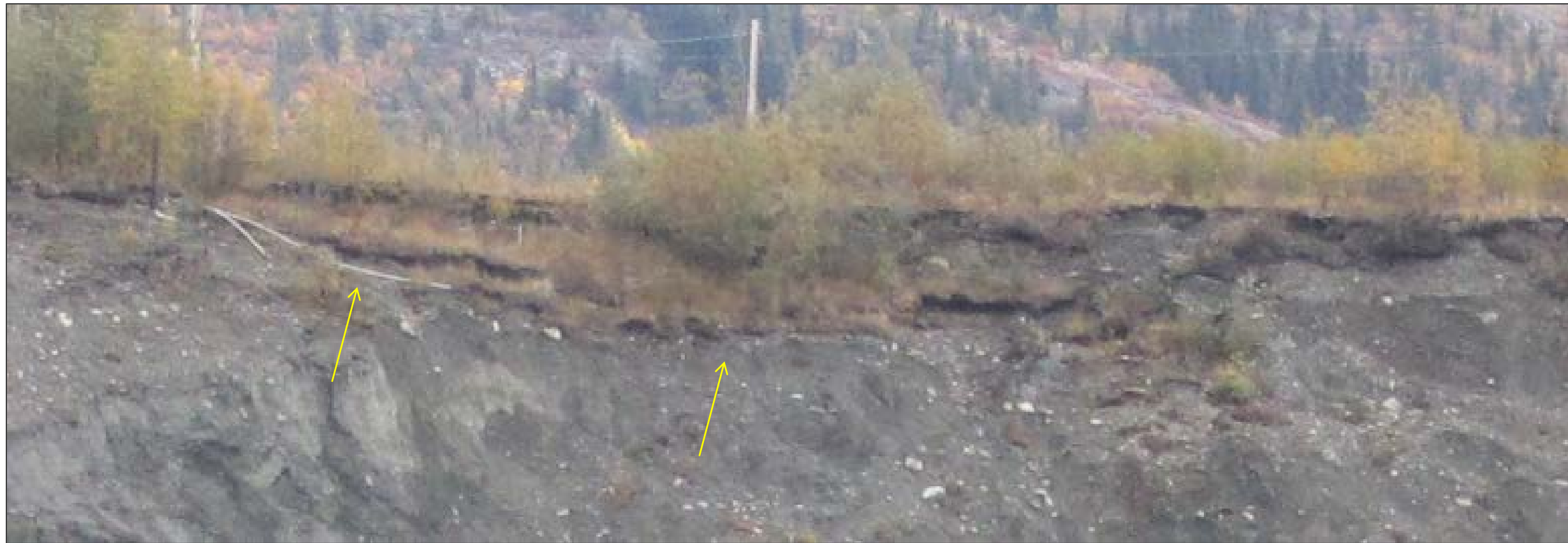
2015 PHOTOGRAPH OF CREST OF EAST WALL, BACKSCARP OF INSTABILITY ZONE, VIEW LOOKING EAST
