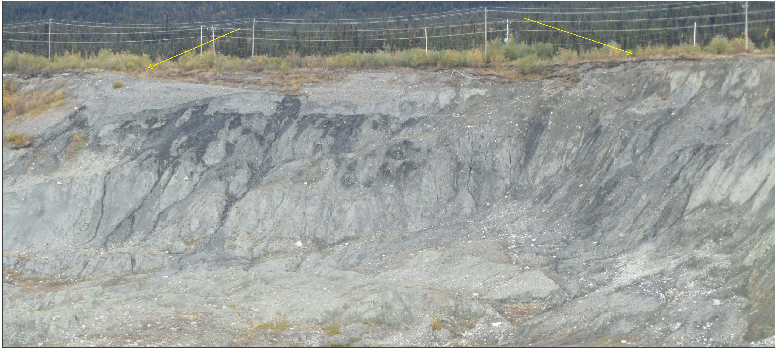
INSTABILITY ZONE, EAST WALL, VIEW LOOKING NORTHEAST
