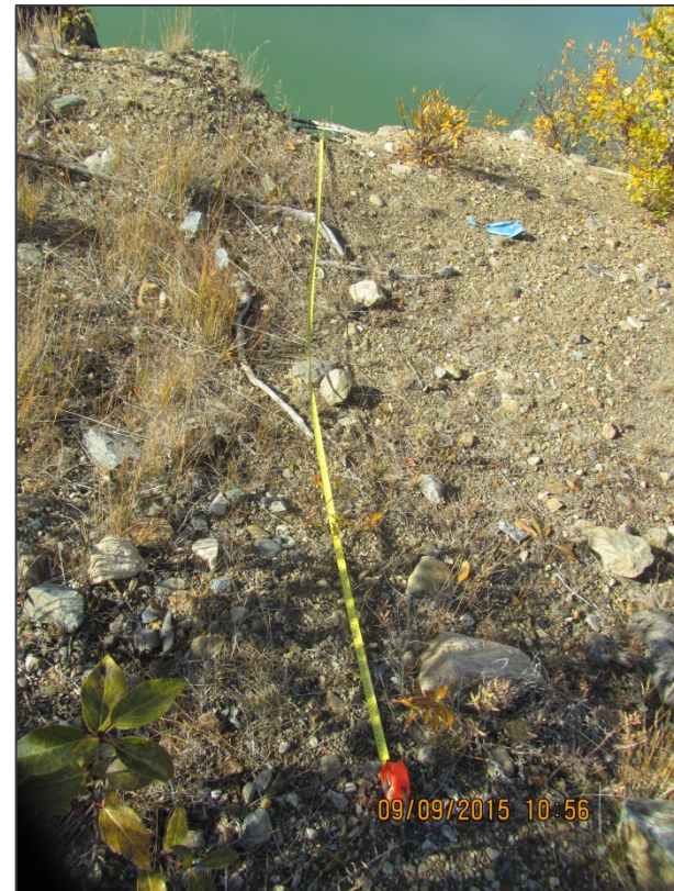
DISTANCE FROM CREST TO EDGE OF BERM IS APPROXIMATELY 3 METRES NEAR PIN 15742
