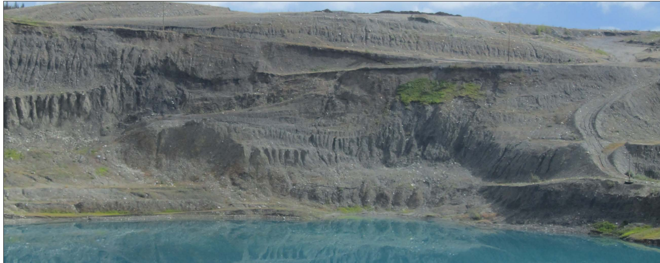
2014 PHOTOGRAPH OF INSTABILITY ZONE, VIEW LOOKING EAST
