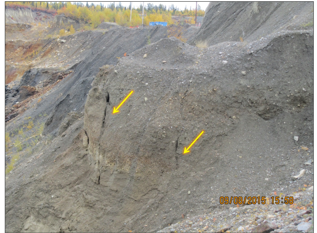
NORTH SIDE OF WEST WALL, VIEW LOOKING SOUTH FROM CREST ARROWS INDICATE CRACKS
