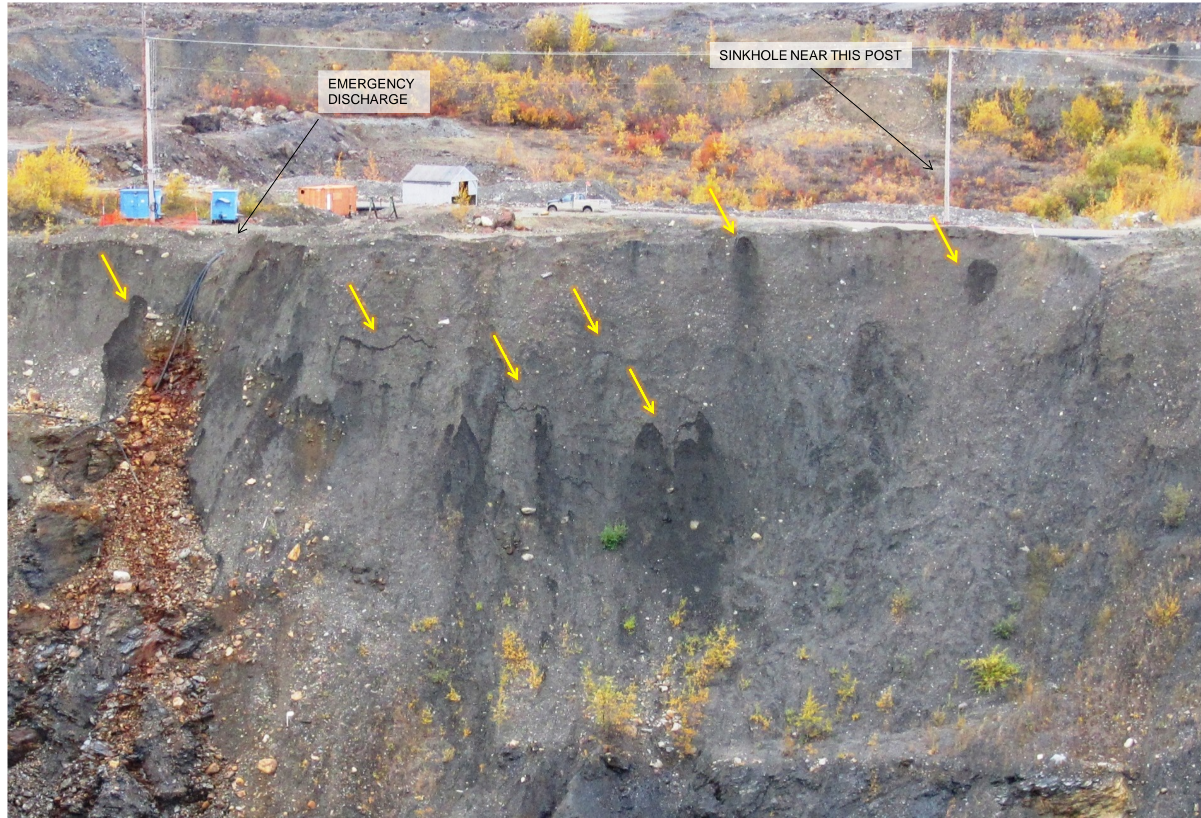
SOUTH SIDE OF UPPER WEST WALL, VIEW LOOKING WEST YELLOW ARROWS INDICATE CRACKS OR SLUMPED AREAS
