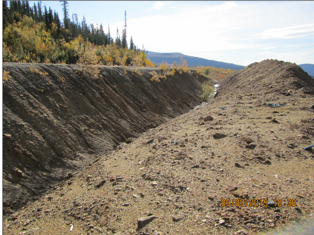
BERM AT CREST OF EAST WALL, ON WEST SIDE OF ROAD, VIEW LOOKING SOUTH
