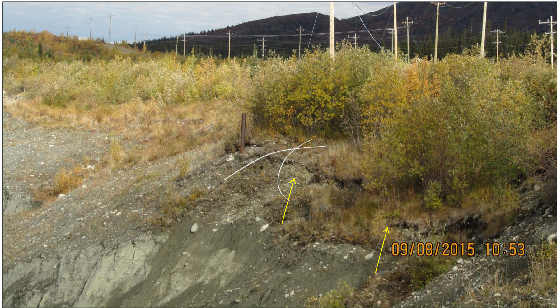
SECOND SET OF CRACKS LOWER DOWN ON CREST OF EAST WALL NEAR NORTH ARRAY, VIEW LOOKING NORTH
