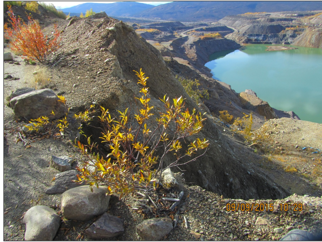
TILL SLOWLY ERODING AND RAVELING
