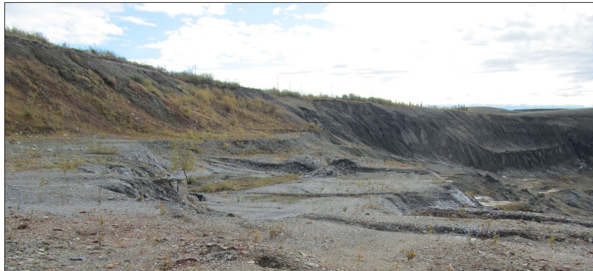
2015 PHOTOGRAPH OF ROCK BENCH TO THE NORTH OF THE INSTABILITY ZONE, EAST WALL, VIEW LOOKING SOUTH
