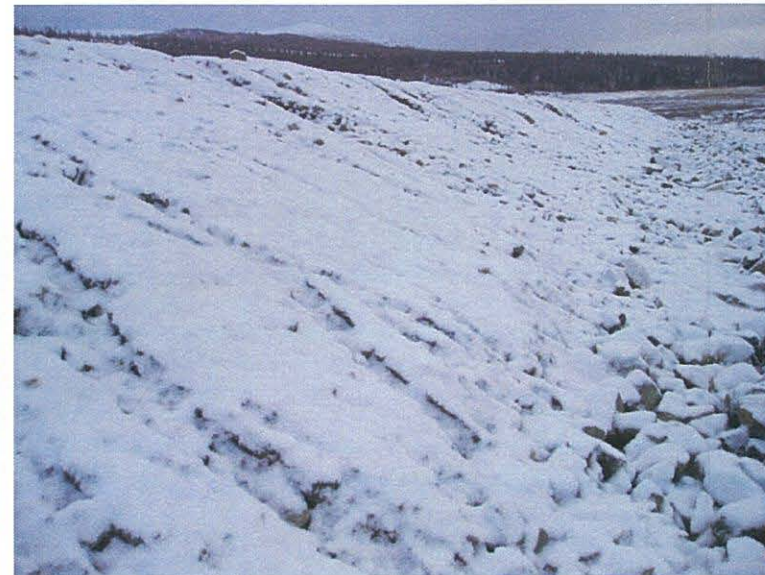
September: Shows a number of small erosional gullies which are formed higher up on the cut channel. The erosional gullies are relatively minor except for the occasional one which is perhaps 1 metre across by perhaps 1/3 to 1/2 metre deep.
