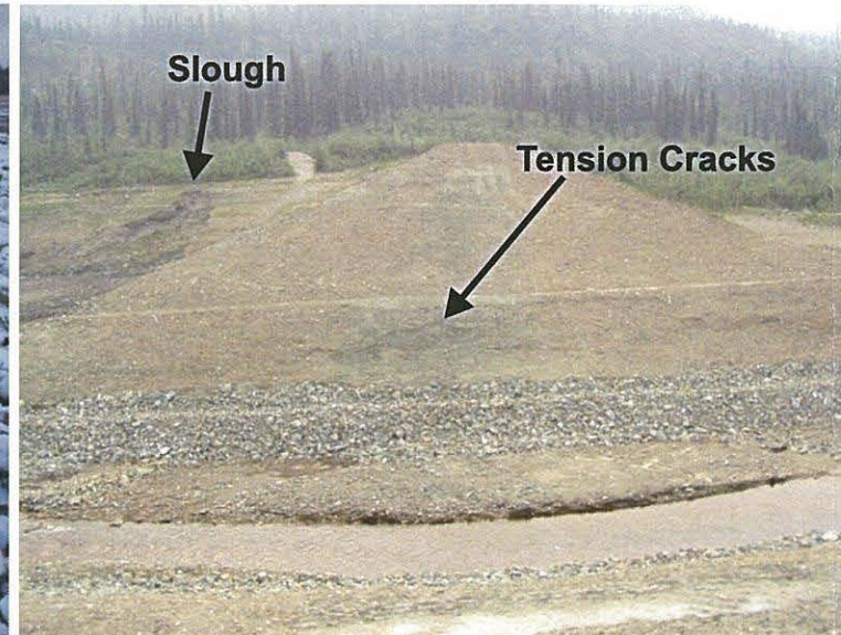
August: Shows a view of the cutslope on the south side of the breach. There is one scarp on this side of the channel, caused by some slumping of the material.
