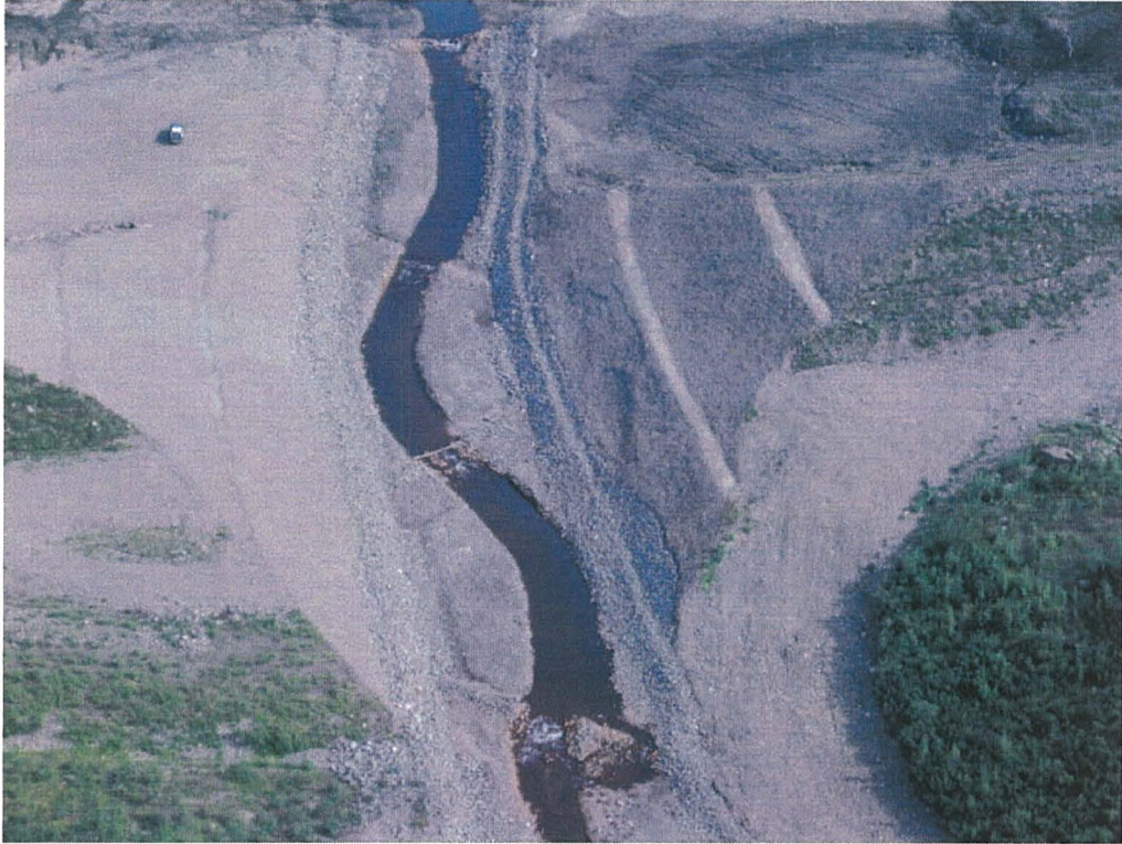
Photo #13: Aerial view for comparison from 2004 of the constructed channel within the breach.
