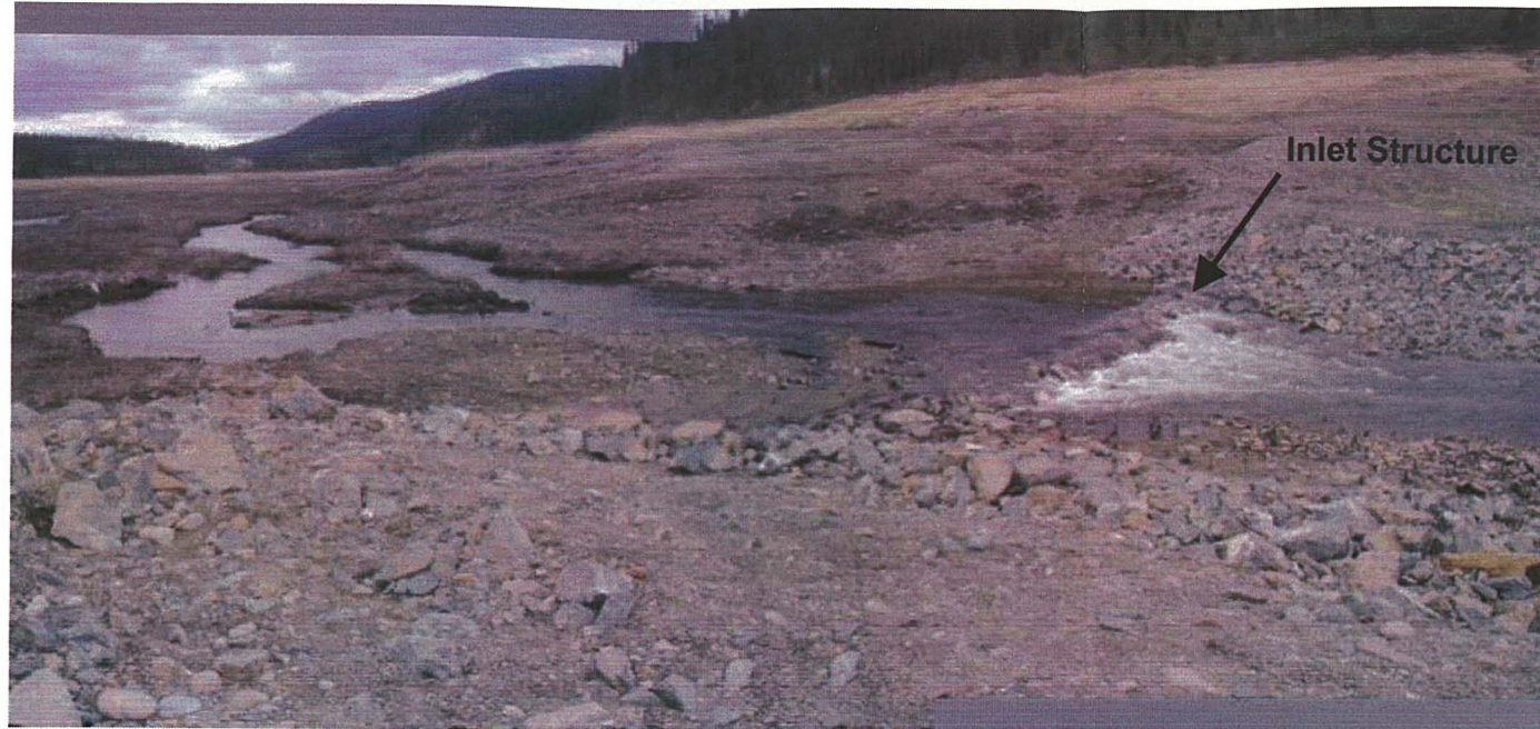
May: View of the inlet structure and the channel immediately upstream of the breach. The channel has formed into a braided stream upstream of the inlet structure.
