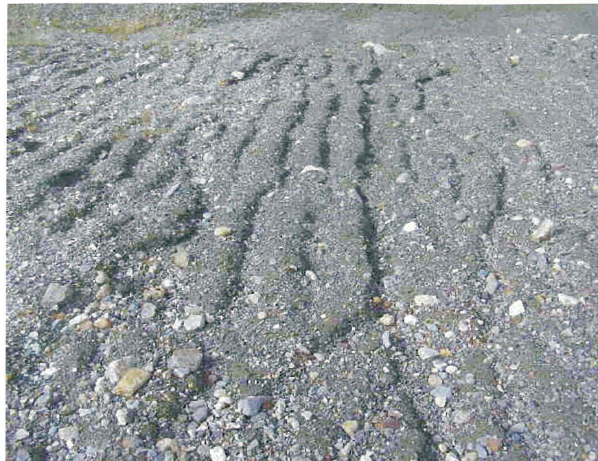
June 2007: A close-up view of some of the rill erosion that have been formed into the cut face of the dam.
