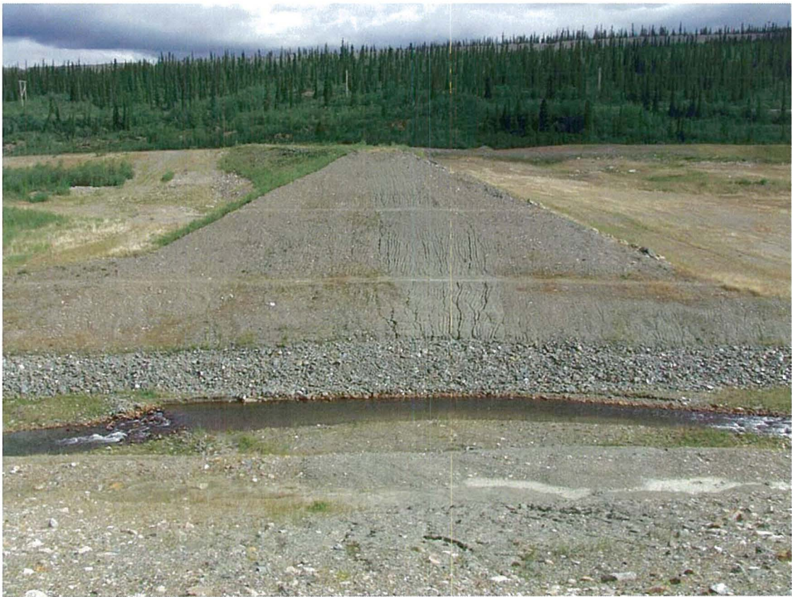
The north side of the dam breach has little vegetative cover and minor erosion channels are present on the steep compacted surface of the core.
