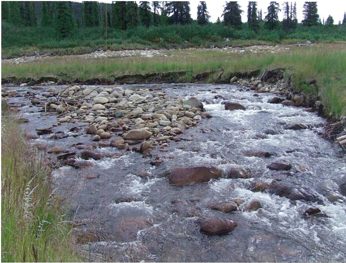
Photo #1: An area of bank erosion in Reach #1, July 25, 2006.
