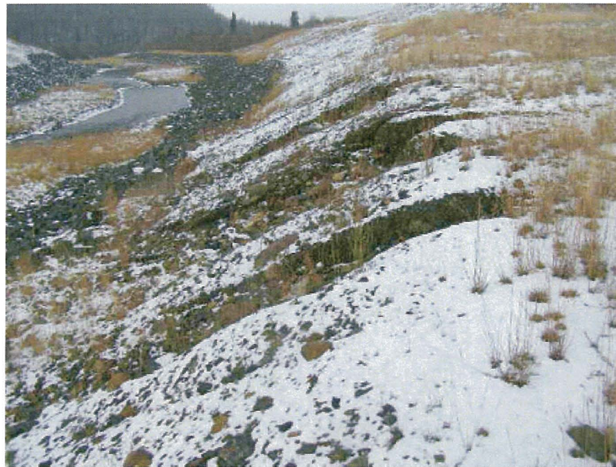
September 2007: View of the erosion gullies forming between the inlet structure and riffle on the right bank.
