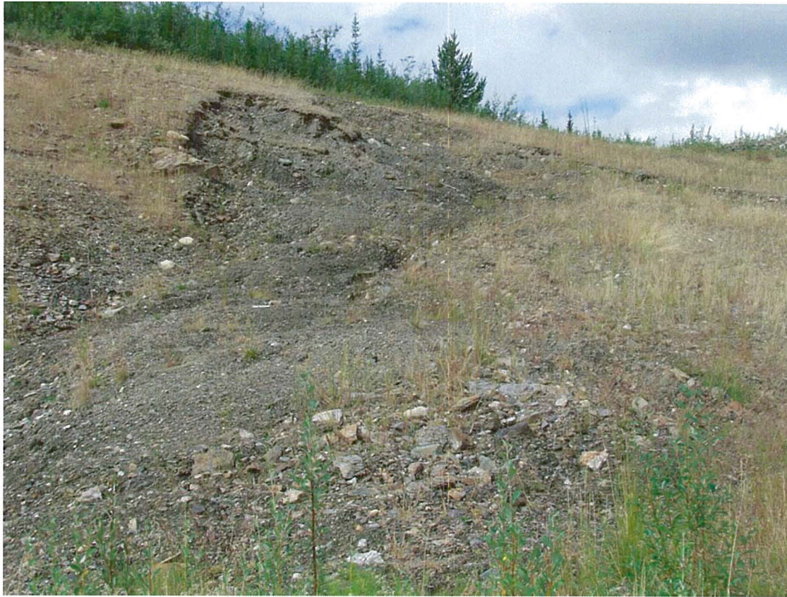
The eroded gully shows continued sign of revegetating naturally from the seeded species, and appears stable.
