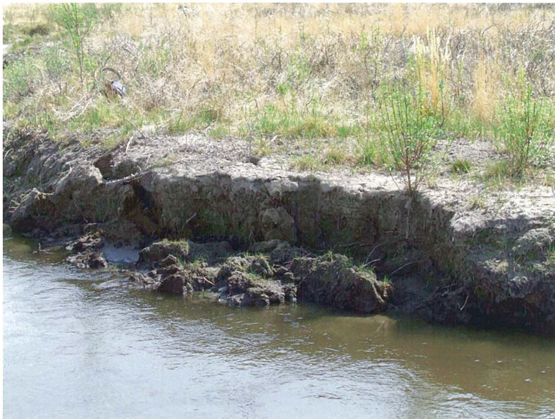
Photo # 8: Bank instability in Reach #3, June 5, 2007.
