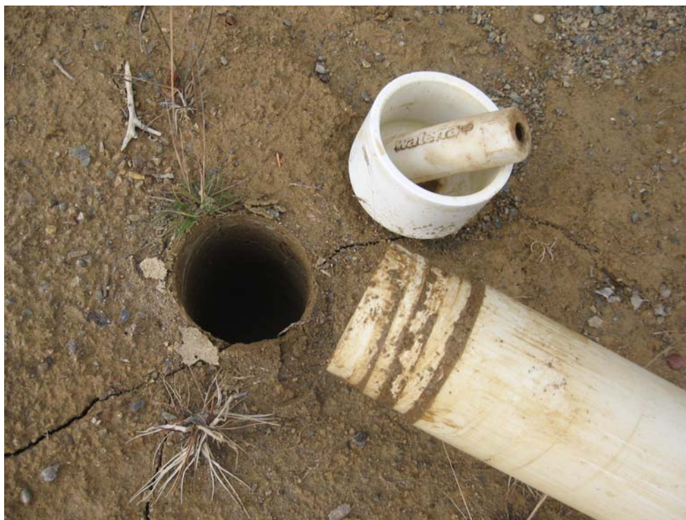
Photograph 4. Well BH7D after top section pulled out of ground leaving open hole down to well in ground. Foot valve clogged with soil.
