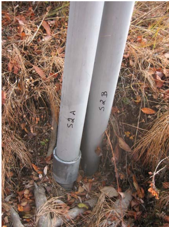
Photograph 8. Wells S2 A,B. Nested Wells. Well S2A has loose coupling at ground surface and top section of well can be removed
