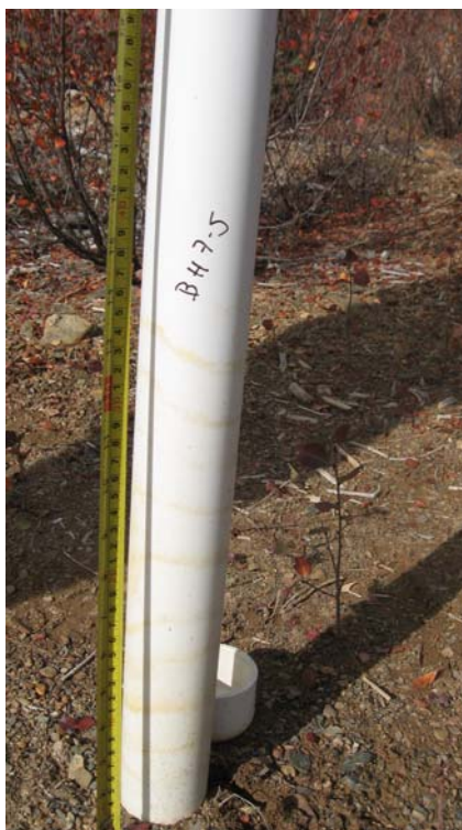
Photograph 6. Well BH7S showing frost jacking lines at base of well
