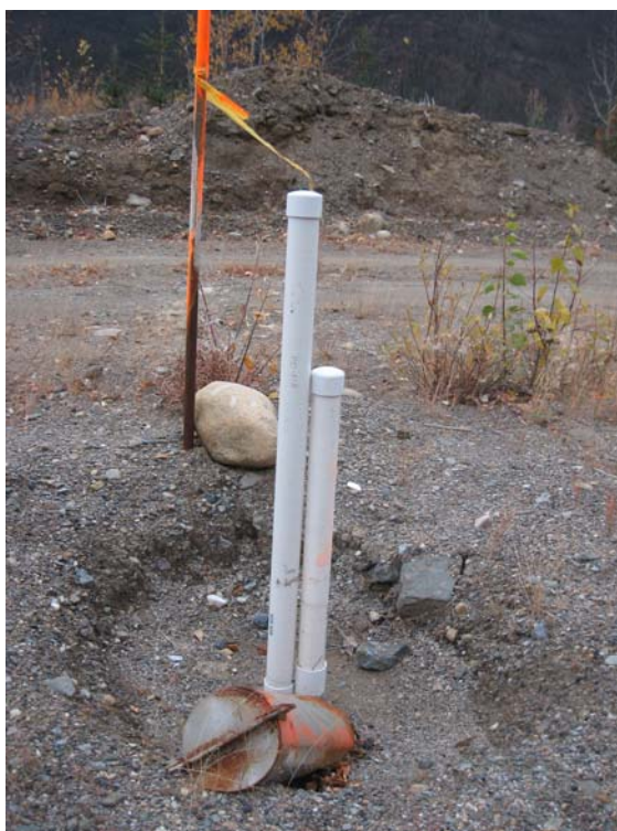
Photograph 14. Well P01-01A (shortest) and P01-01B (longest) prior to rehabilitation. (Sept. 2006)
