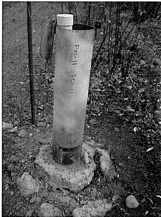
Photograph 2. Well P01-11 at base of Cross-Valley Dam. Concrete around base of well is broken, steel casing is loose and can be moved back and forth manually
