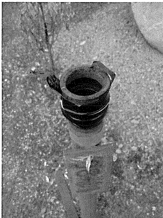
Photograph 13. Well TH86-17, 2" steel well with obstruction / joint at 10.17 m btoc which sometimes prevents lowering of sample tubing to bottom of well at 15.10 m btoc.
