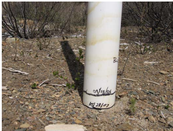
Photograph 1. Evidence of frost-jacking at BH7S over winter 2006-2007.
