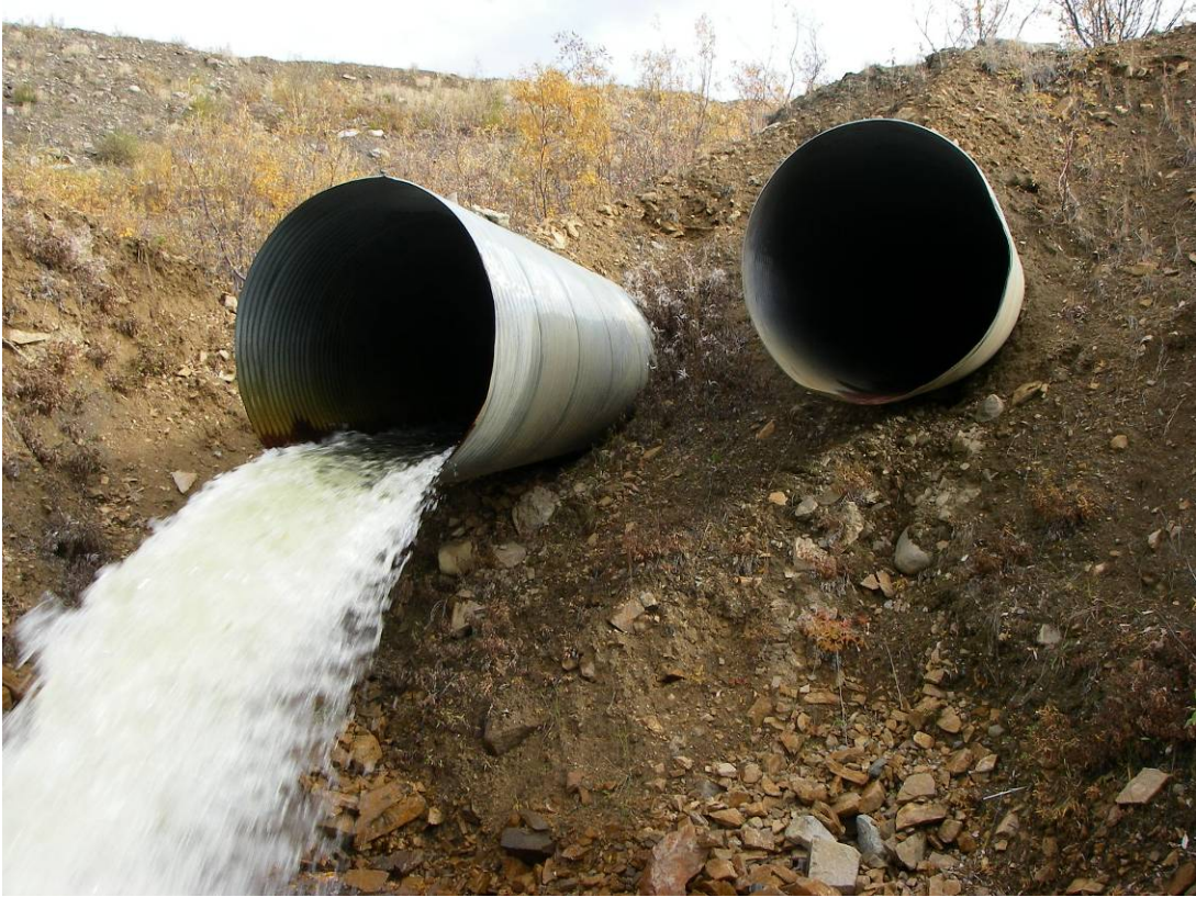
Photo 23: Discharge at outlet of HR-4 (Sept. 16, 2007).
