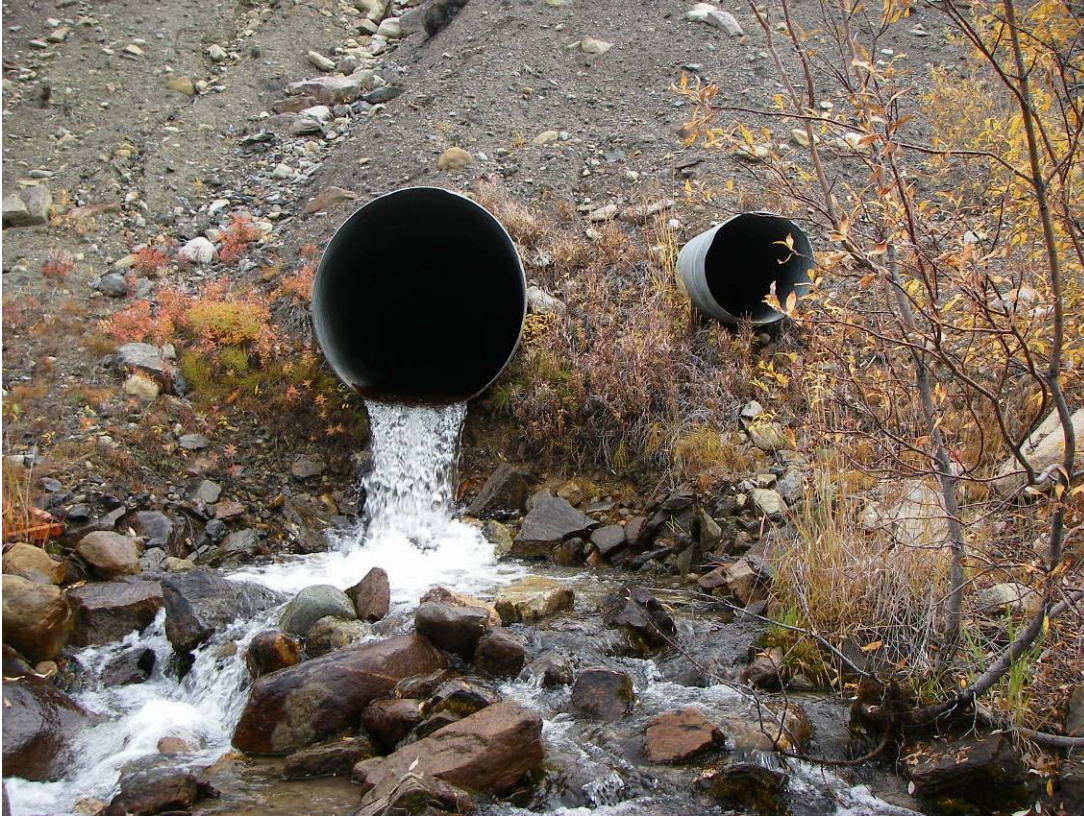
Photo 15: Discharge at outlet of HR-2 (Sept. 16, 2007).
