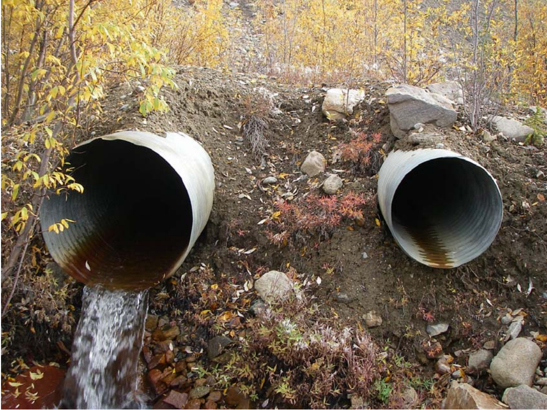
Photo 19: Discharge at outlet of HR-3 (Sept. 16, 2007).
