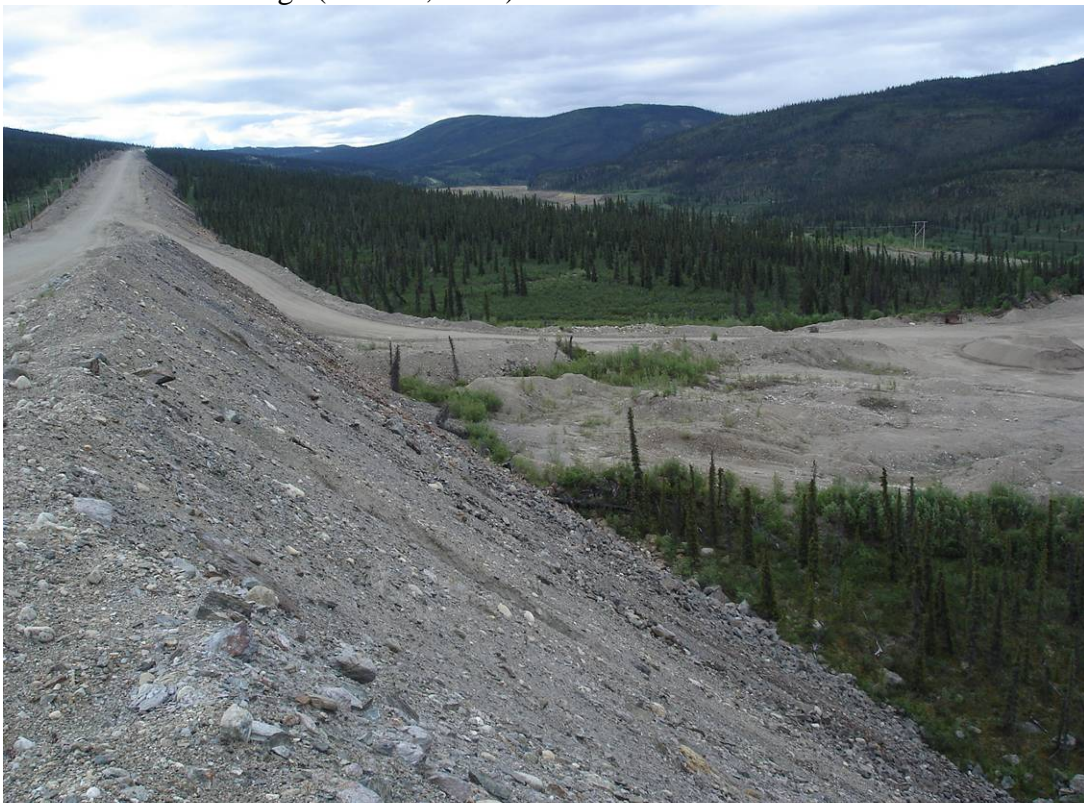
Photo 8: Area on the downstream side of the Haul Road, immediately east of the RC Drainage (June 22, 2006).
