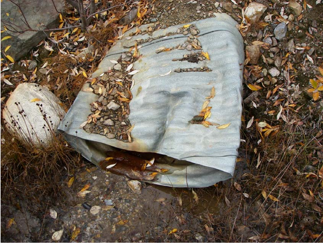
Photo 9: Corrugated pipe at the inlet of HR-1 (Sept. 16, 2007).
