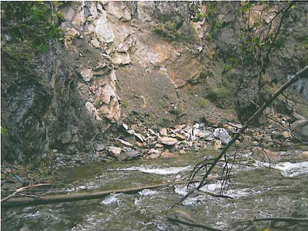
Photo 9: Rock slide at the upstream end of Vangorda Creek site V8 sample site during 2008. The materials that slid are surrounded by mineralized materials visible on the left side of the photo.
