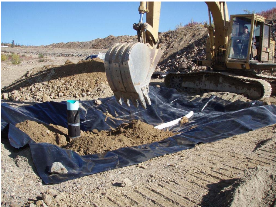
Photo 5a Lysimeter Installation, First Steps: i) sand and geofabric underlay, lysimeter L1; ii) backfilling over geomembrane liner at lysimeter L2, showing riser pipe and 10 cm diameter collection drainpipe.
