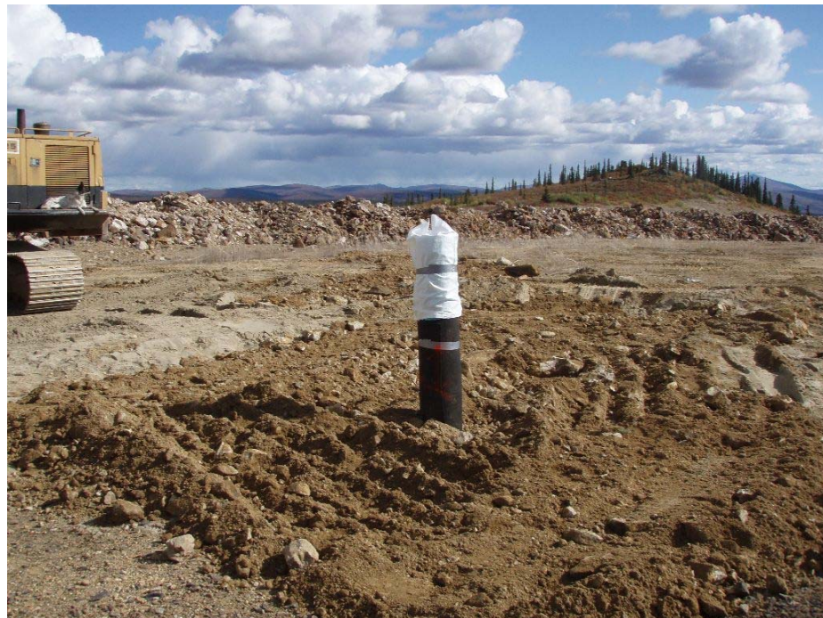
Photo 5b Lysimeter Installation, Final Steps: i) liner trimmed and backfilling partially complete, lysimeter L1; ii) installation complete, lysimeter L1.
