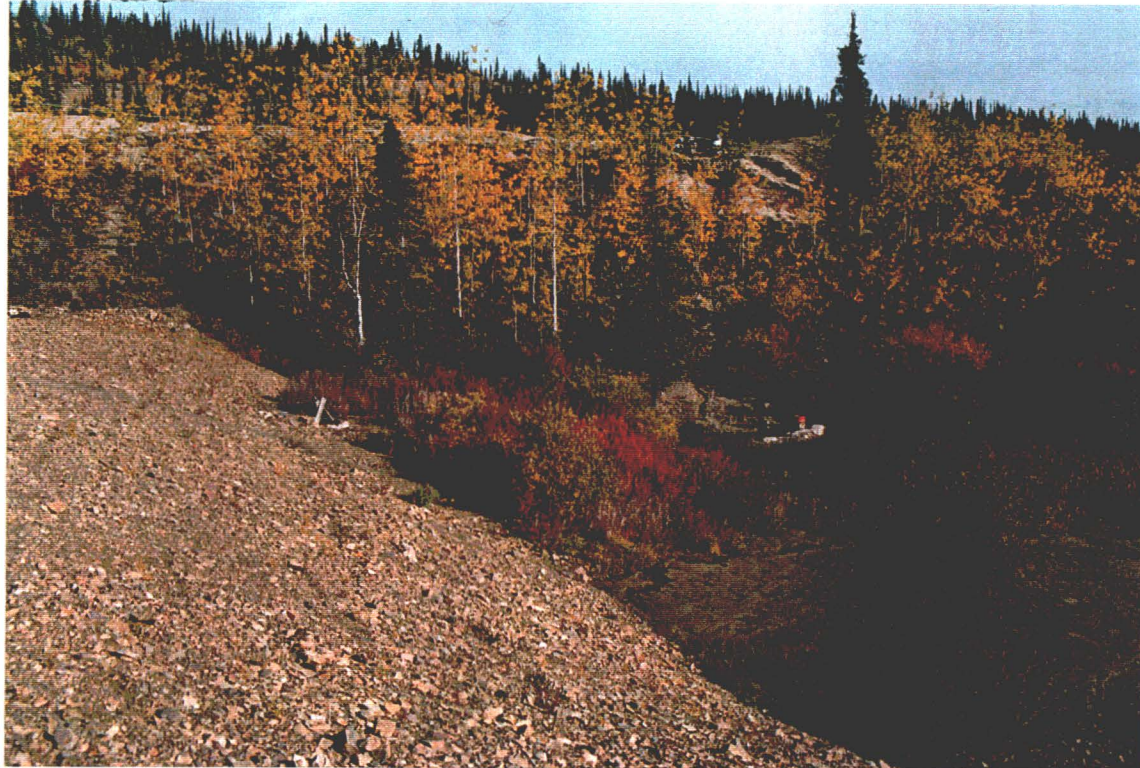
Photograph 9 Seepage Control Dam downstream slope - looking northeast (observable seepages exiting from the toe).
