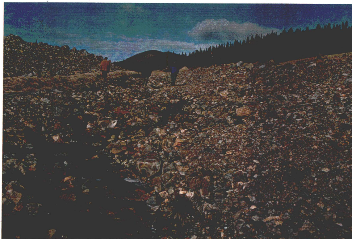
Photograph 10 Emergency Spillway Channel - lower segment (used also for conveying water from North Diversion Ditch).
