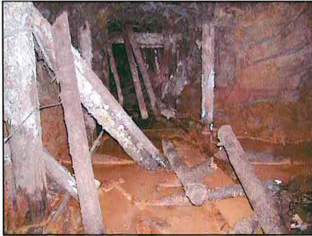
Plate 18 – Collapsed timbers in underground workings of G300 level
