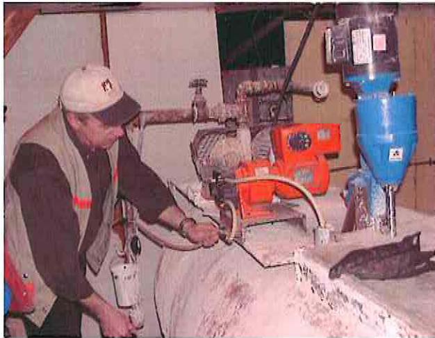
Plate 4 - Lime slurry mixing-tank and peristaltic delivery pump at Silver King 100 treatment site
