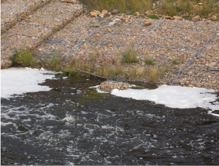
Photo 32: Vertically displaced gabion basket at DS3 looking north.
