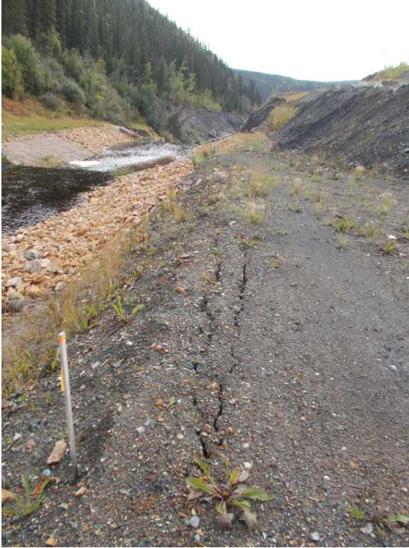
Photo 26: Tension cracks located along south bank of DS1 looking east (downstream).
