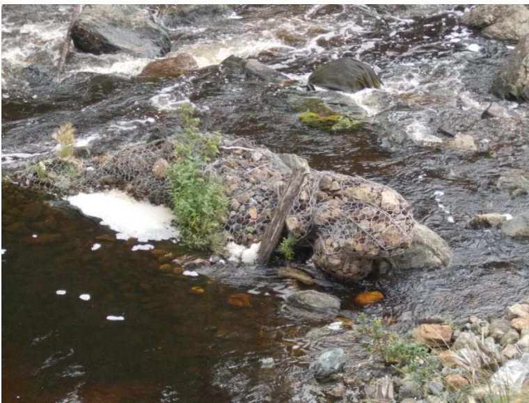
Photo 35: Failed gabion basket downstream (east) of DS4.
