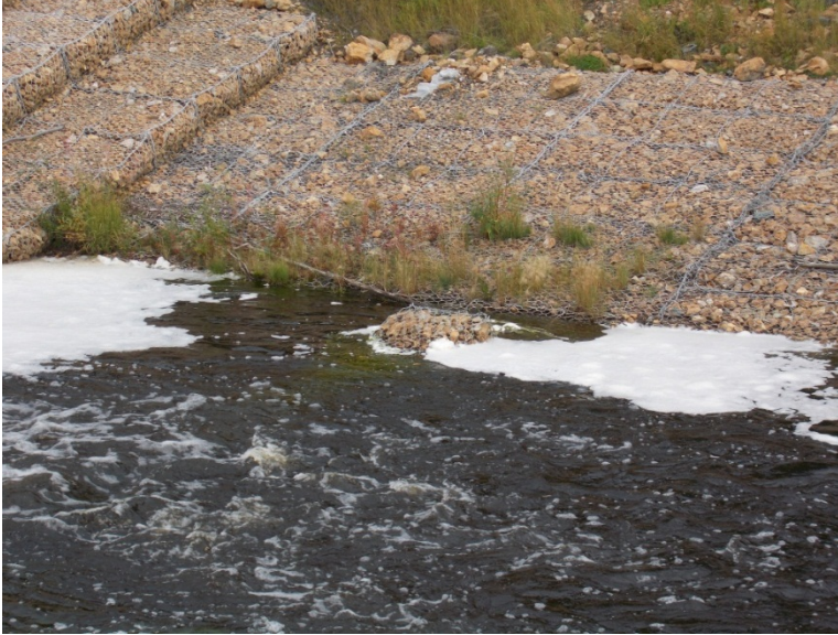
Photo 32: Vertically displaced gabion basket at DS3 looking north.
