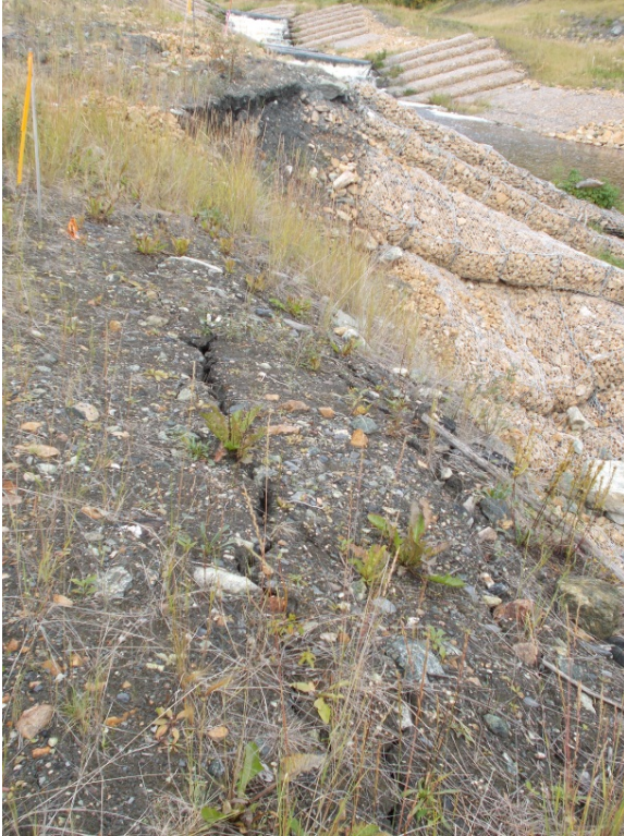
Photo 36: Tension cracks along south bank of DS4 looking west (upstream).
