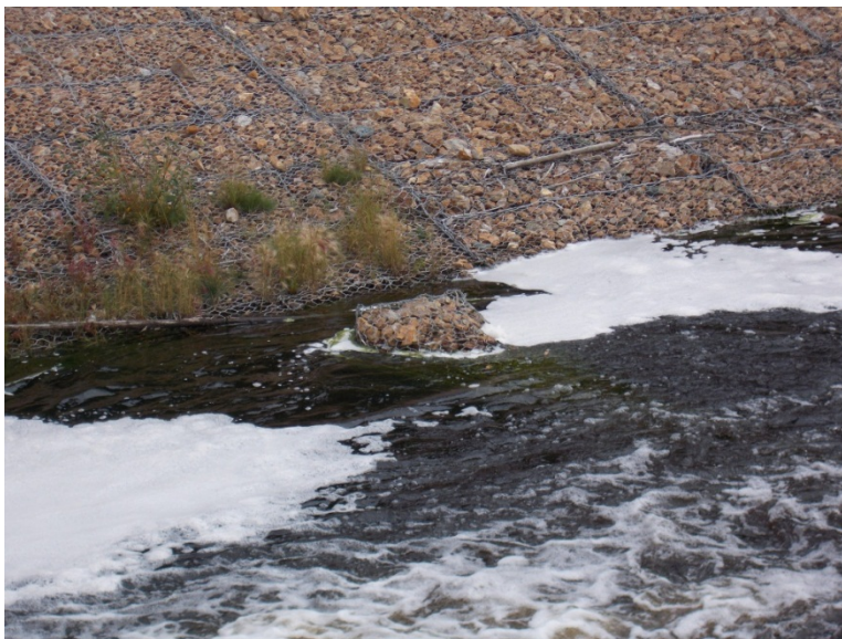
Photo 29: Vertically displaced gabion basket at DS3 looking northeast.
