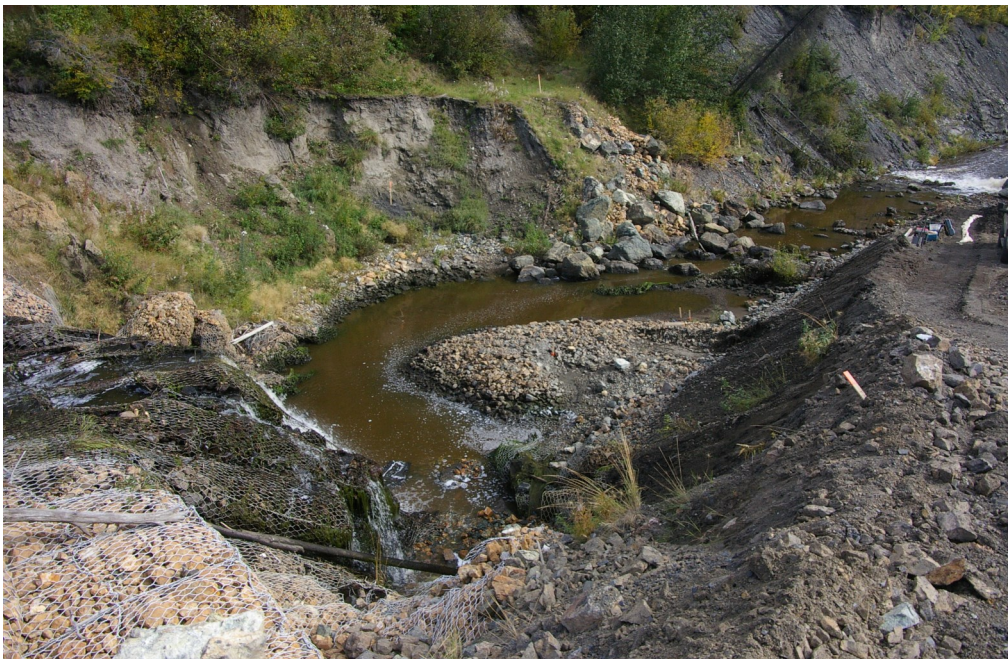
Photo 4: View of the instream work area below drop structure 4 following the full closure of the Hudgeon Lake outlet (all water flowing through diversion). Fish salvage was underway at the time of the photo. Photo taken September 2, 2015.
