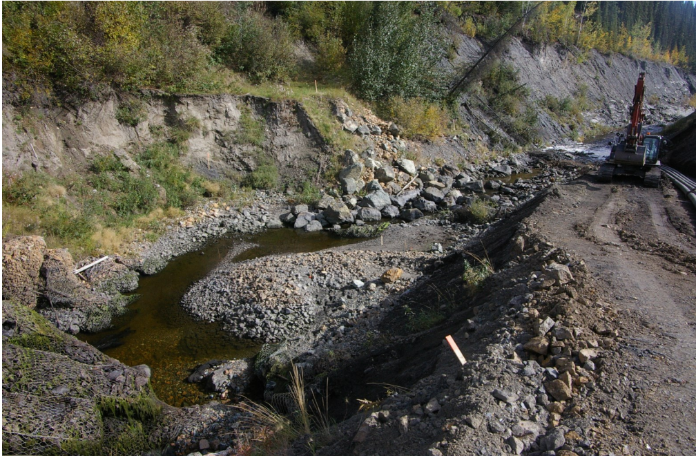
Photo 5: View of the instream work area below drop structure 4 on September 3, 2015, after all drop structures had dewatered for 24 hours. Salvage had been completed at the time of this photograph.
