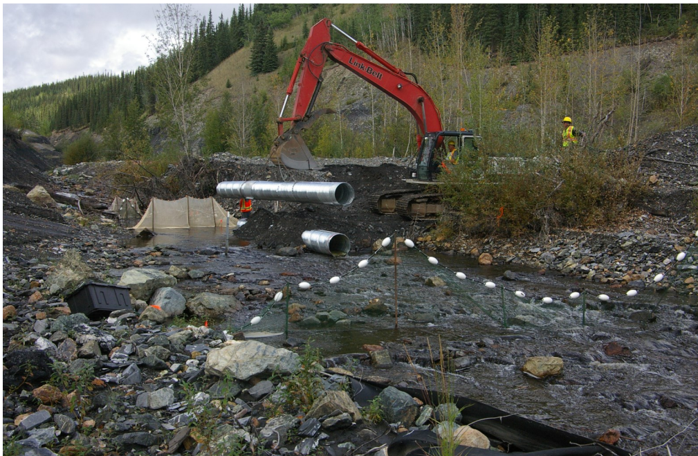
Photo 2: View of the isolated and salvaged area at the Clinton Creek ford crossing location during culvert installation. Note the original extent of isolation (upper left net in background) and the revised smaller area (closer net in upper left). Photo taken August 10, 2015.
