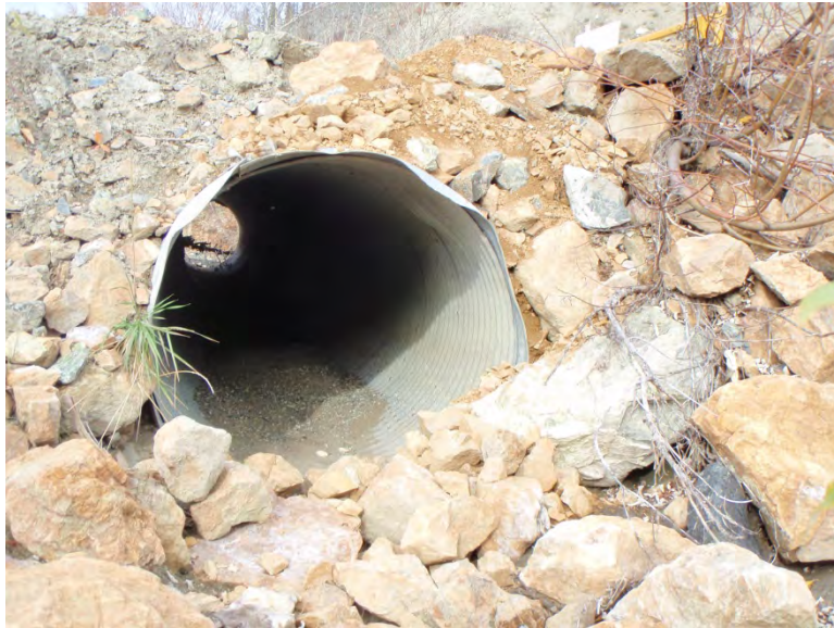
Photo 49: Wolverine Creek high flow culvert outlet looking north.
