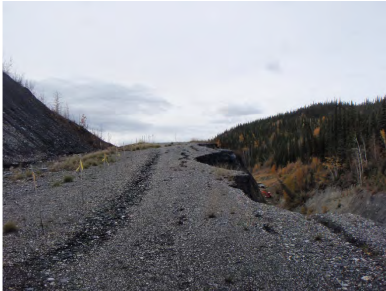
Photo 13: Closed portion of access road top of bank looking west.
