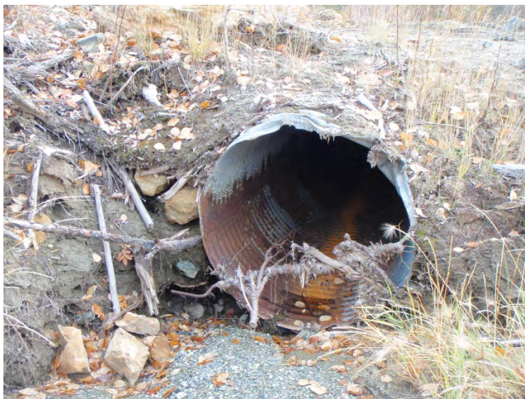
Photo 50: Wolverine Creek high flow culvert inlet looking south.
