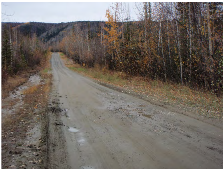
Photo 2: Access road washboarding between Fortymile Bridge and site gate looking northeast.
