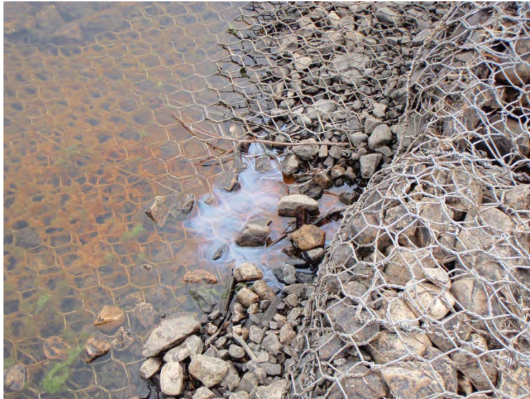
Photo 25: Drop Structure No. 2 unknown substance in downstream pool looking southeast.
