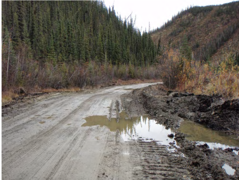
Photo 1: Access road low spot between Fortymile Bridge and site gate looking east.
