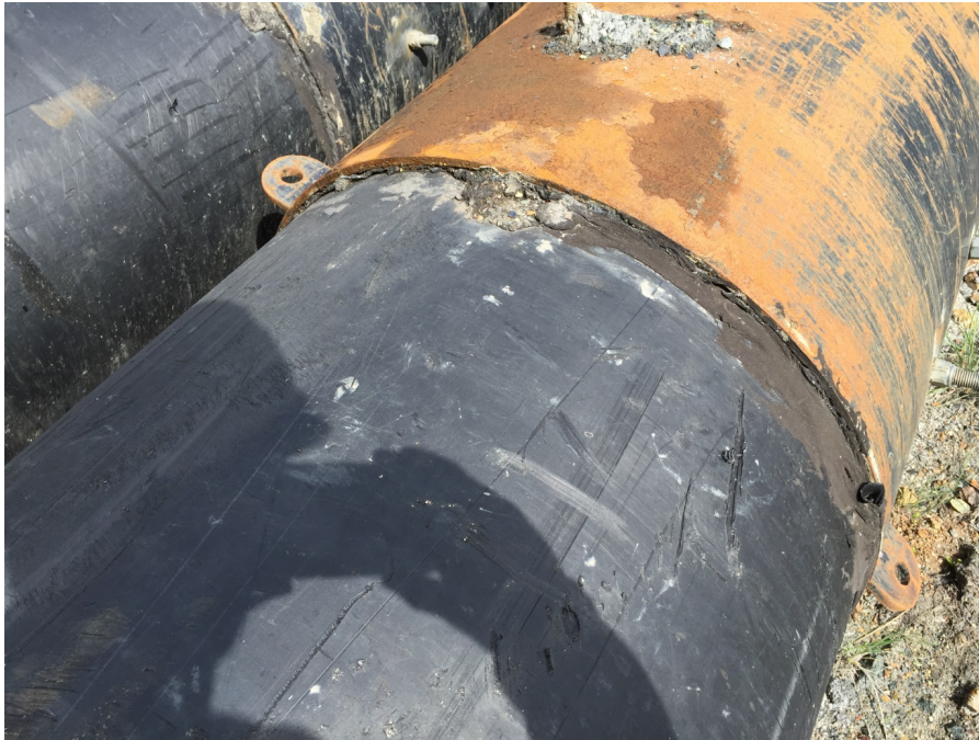
Photo 16 Log Boom End – Cracking Seal
