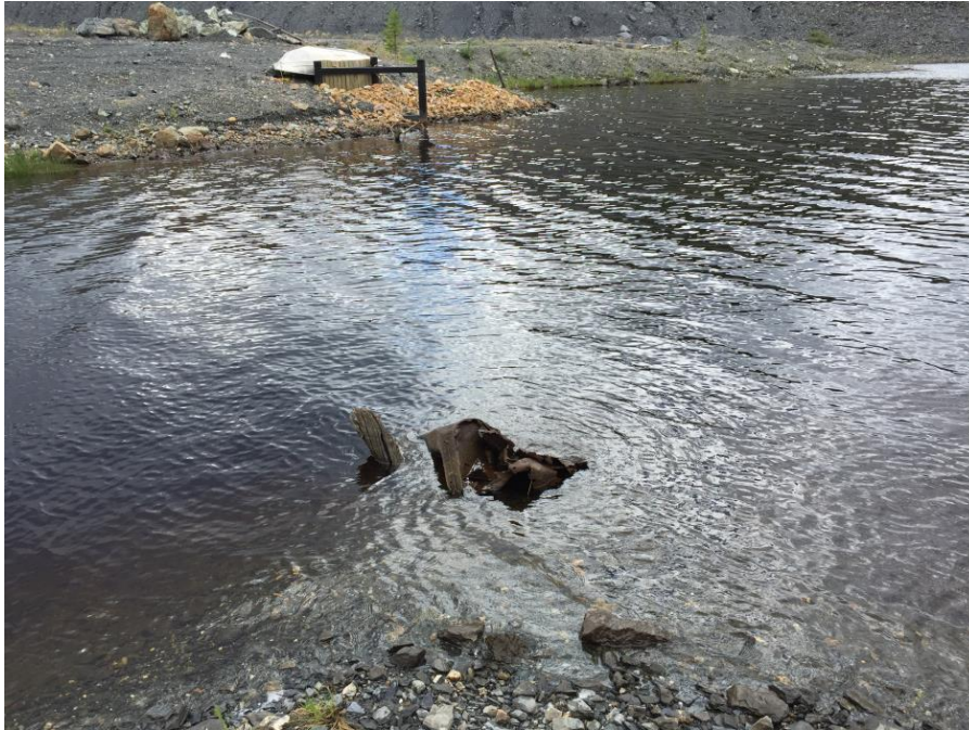
Photo 10 Rusted Metal at Lake Outlet
