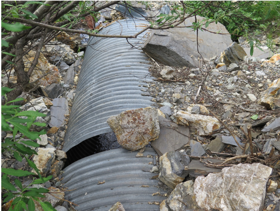
Photo 4 Washed out Culvert (looking at outlet) 5 km from the Forty Mile Bridge
