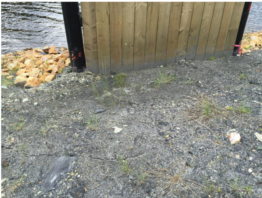
Photo 13 North Boom Abutment, cracks in soil around abutment
