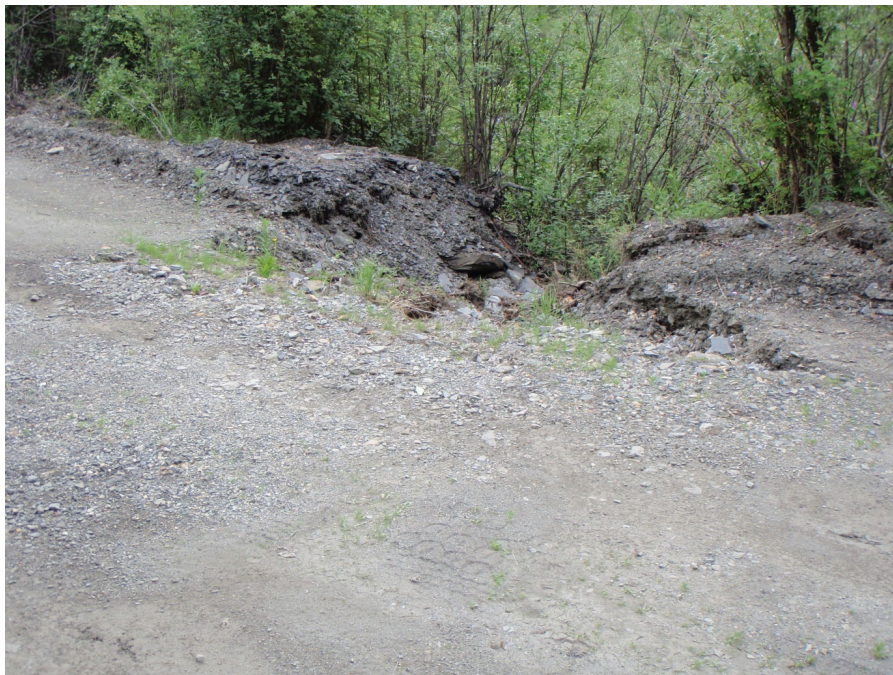
Photo 3 Washed out Culvert (looking at outlet) 5 km from the Forty Mile Bridge
