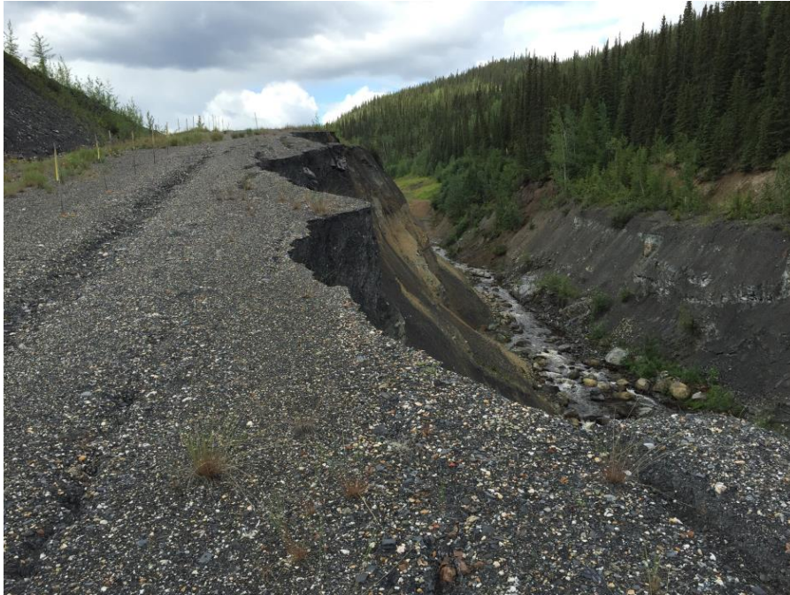
Photo 9 Closed access road looking west – slope continues to slide into Clinton Creek
