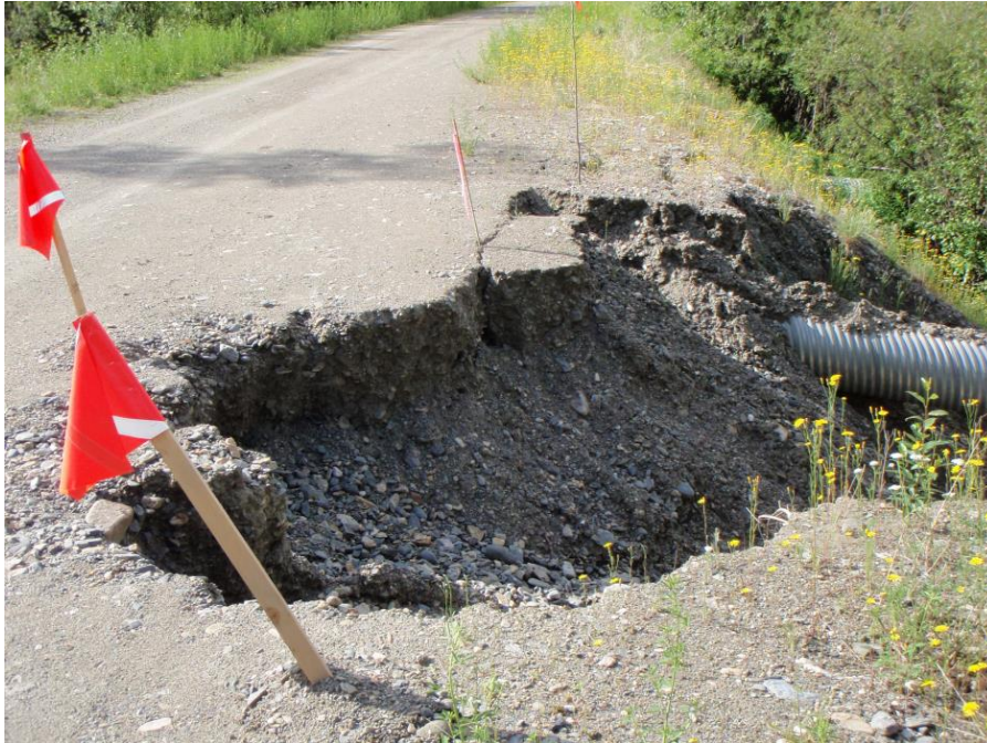
Photo 1 Washed out Culvert (looking at outlet) 500 m south of Forty Mile Bridge
