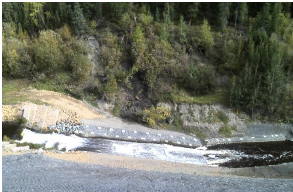
Photo G Landslide near DS4, looking north (August 31, 2016)
