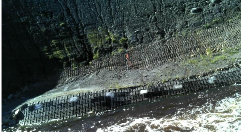
Photo F Erosion of waste rock toe near DS4, looking south (September 3, 2016)
