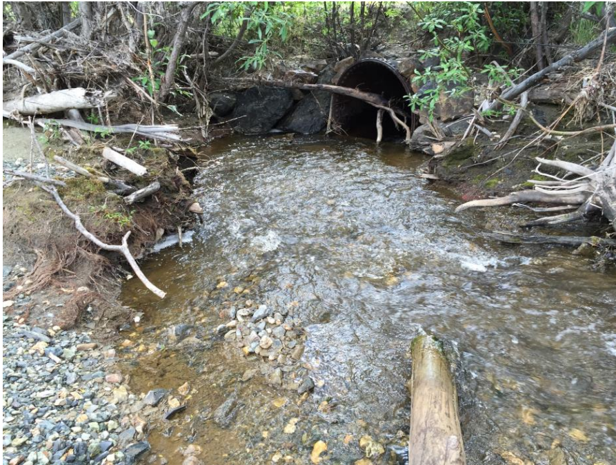
Photo 7 Wolverine Creek low flow culvert, inlet – lodged debris
