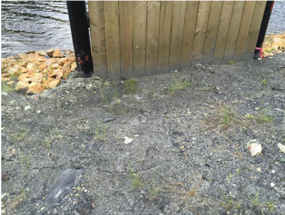
Photo D North Boom Abutment, cracks in soil around abutment (June 21, 2016)
