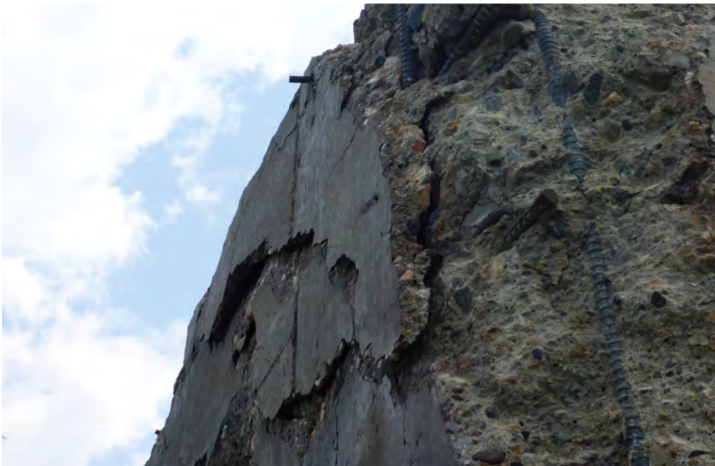
Photo 4: View of a corner of a concrete foundation in the mill area. It's believed that the cracks in the concrete have the potential to provide roosting habitat for bats although no evidence of bat use of these structures was observed. Photo taken on June 25, 2019.
