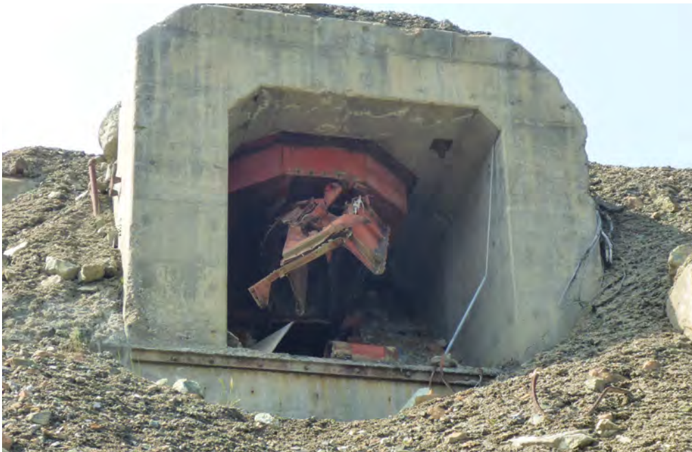
Photo 8: View of a concrete foundation at the edge of the waste rock. No evidence was found that bats were using the structure but it is believed that birds (Say's Phoebe) were nesting within the structure. Photo taken on June 25, 2019.
