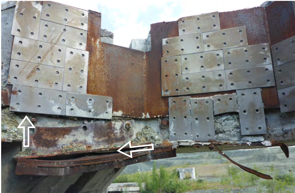
Photo 5: View of the inside one of the concrete foundations in the mill area. It's believed that parts of the structure have the potential to provide roosting habitat for bats (arrows) although no evidence of bat use of the structure was observed. Photo taken on June 25, 2019.
