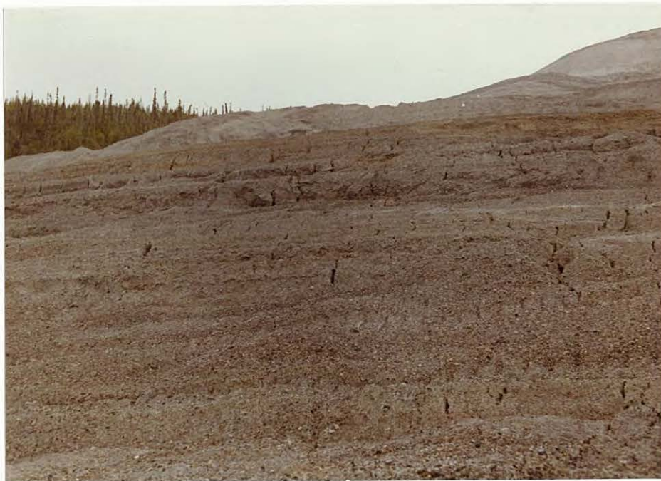
Photo 12: Extensive cracks within the toe area of the south lobe indicate bulging of toe material.
