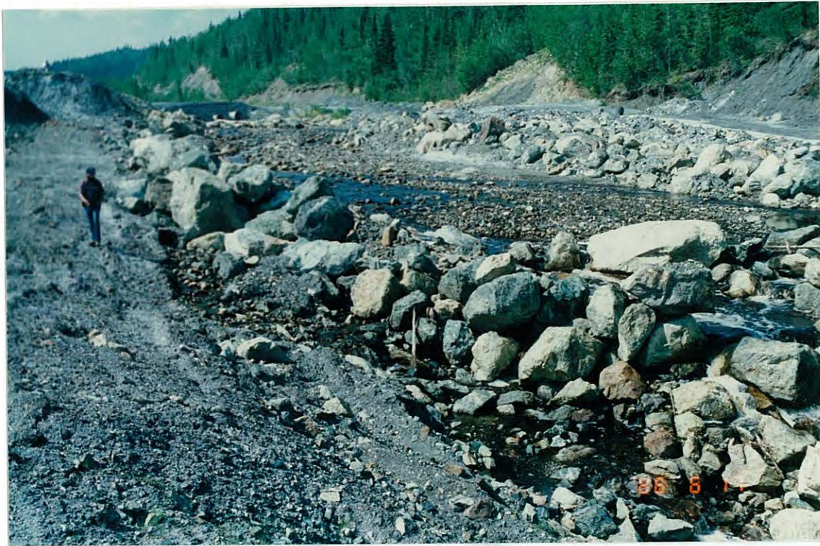
Photo 5: Rock weir constructed in 1984 shows deterioration and erosion along the south bank.
