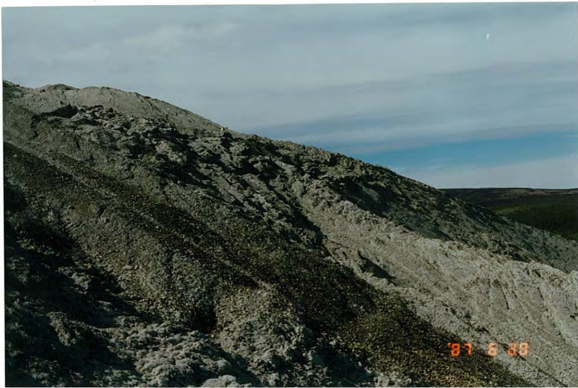
Photo 16: Middle sector of the north pile exhibits extensive deformations and the rate of movement continues to be high.
