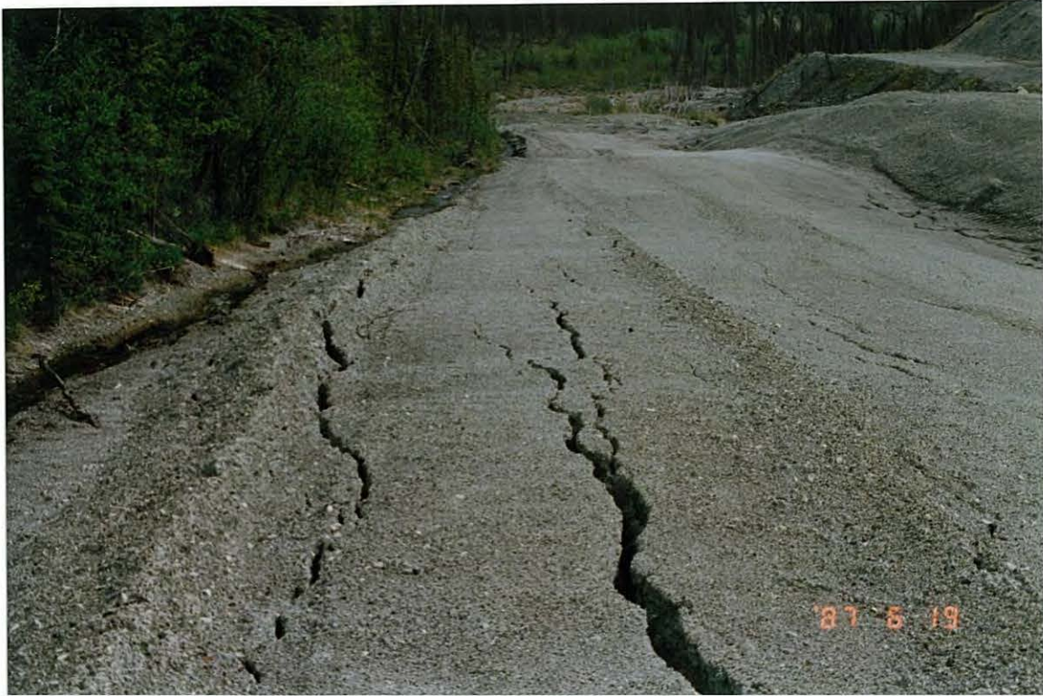
Photo 18: View of tension cracks developed between the armoured channel and secondary channel.
