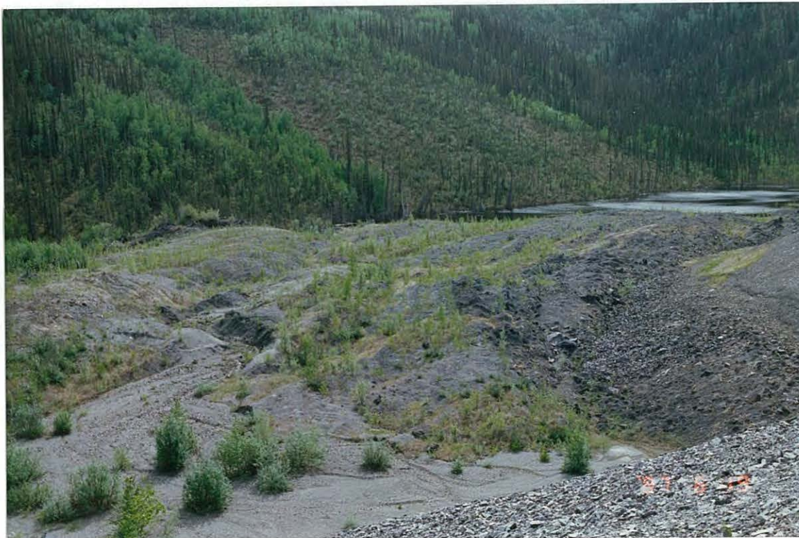
Photo 9: View of the heaved valley floor and bulged waste along the upstream toe of the Porcupine dump. Note an overflow channel directing flow into the dump.
