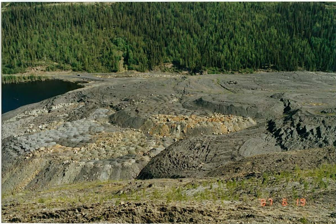
Photo 2: Waste dump - N.W. sector of toe area. Tension cracks run perpendicular to the creek. Recent slumping occurred on the lakeside.
