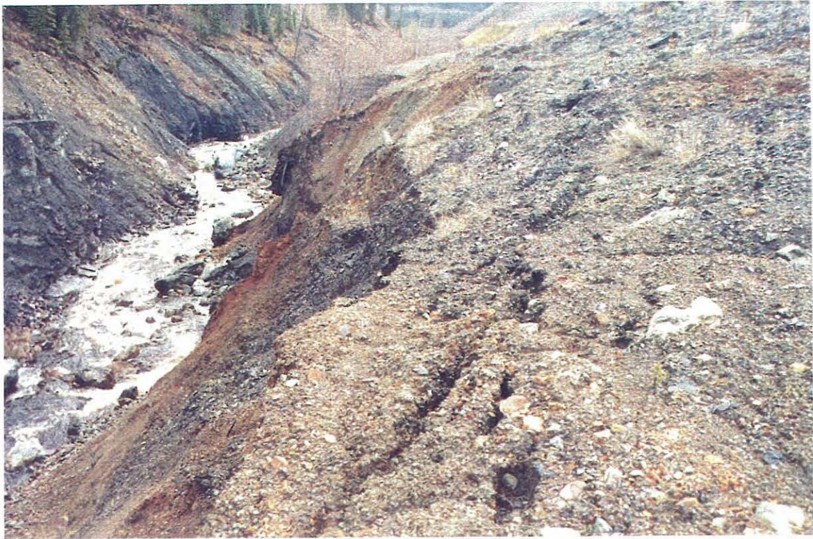
Photo 9: View of the middle segment of the creek channel. Note sloughing of the bank formed by the waste material.
