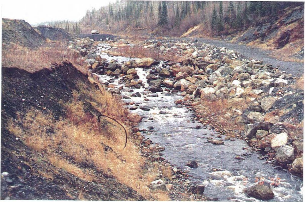
Photo 7: View of the armoured section of the Clinton Creek channel. Refer to photos 5 and 6 of the 1988 report.
