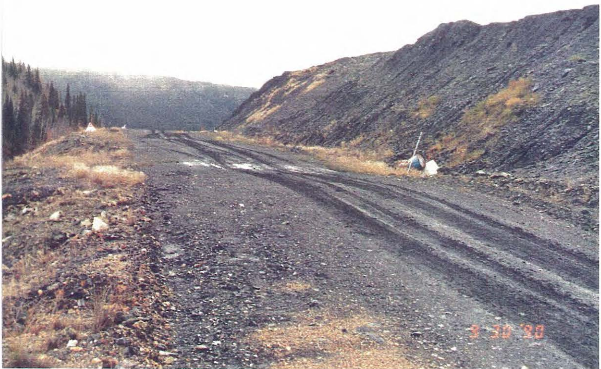
Photo 6: Uneven surface of the access road paralleling the Clinton Creek channel is indicative of ongoing movements.
