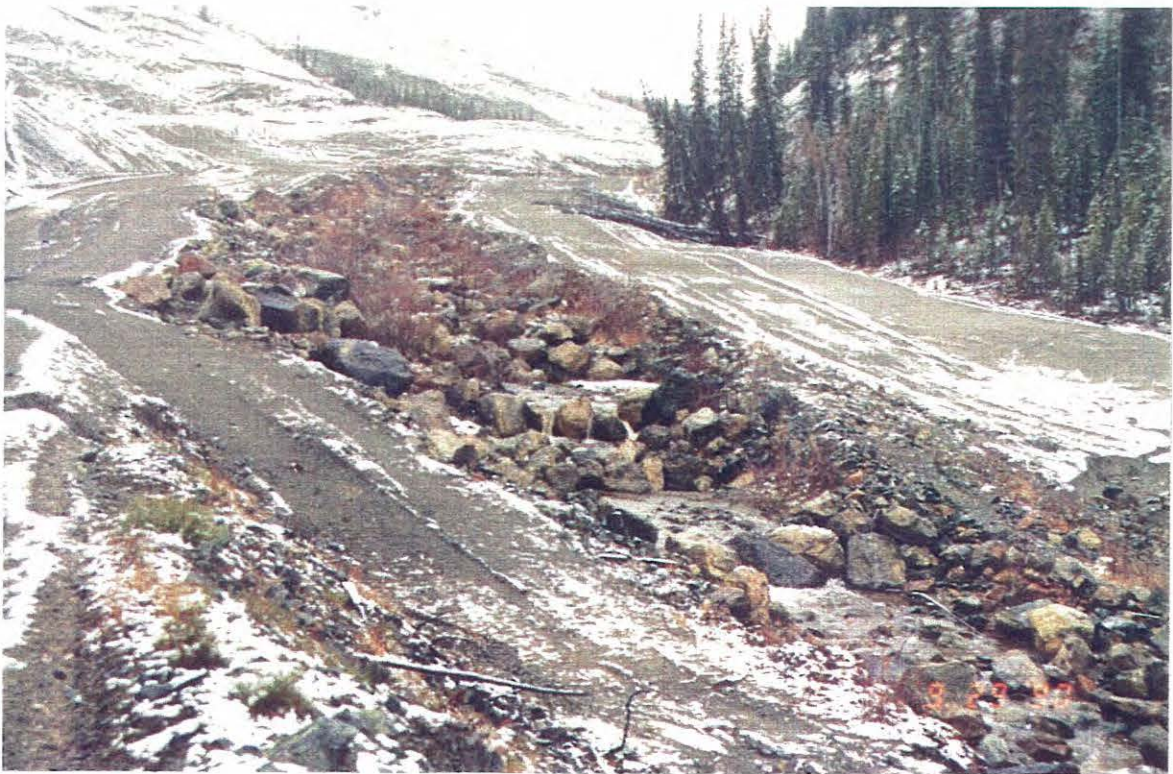
Photo 20: View of the armoured Wolverine Creek spillway. Refer to Photo 22 of the 1988 report.
