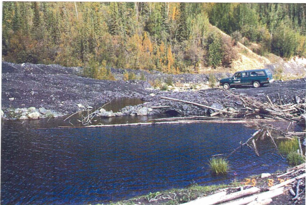
Photo 6: Modified Hudgeon Lake outlet; two culverts have been removed and an overflow channel excavated. The remaining two culverts are partially blocked.
