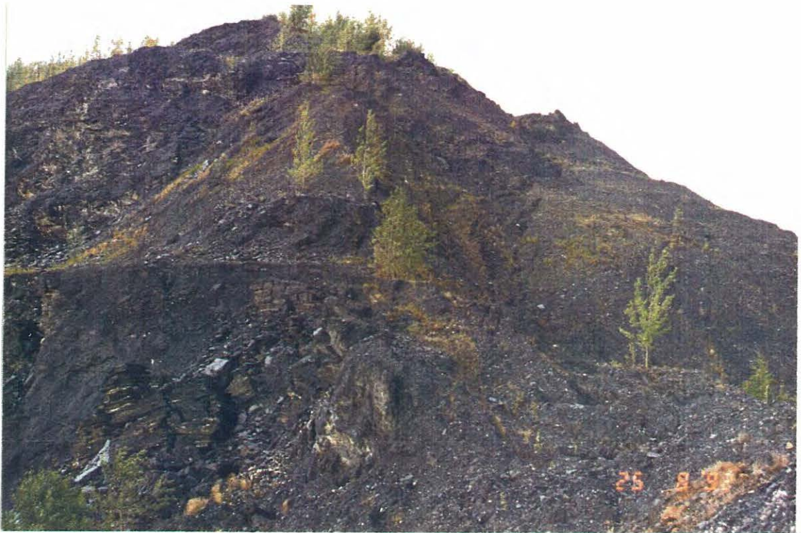
Photo 3: View of a ridge between the Porcupine pit and Clinton Creek waste dump. Slides from the pit wall extend into the dump material.
