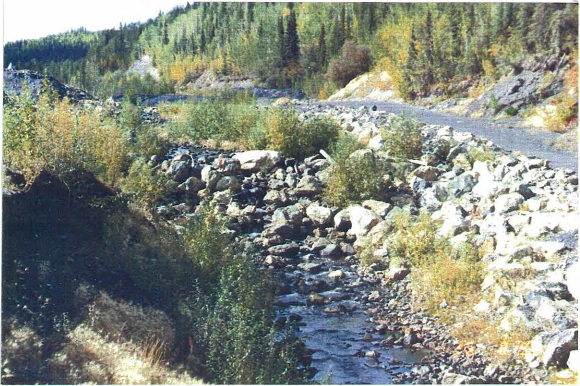
Photo 7: A notch was eroded into the armoured channel plug (left from the big boulder) since 1990.
