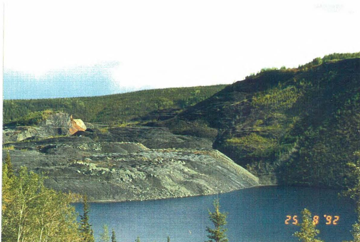
Photo 1: Clinton Creek waste dump and Hudgeon Lake in the foreground. While the general configuration appears to be similar as in 1990, cracks and scarps confirm ongoing movement.
