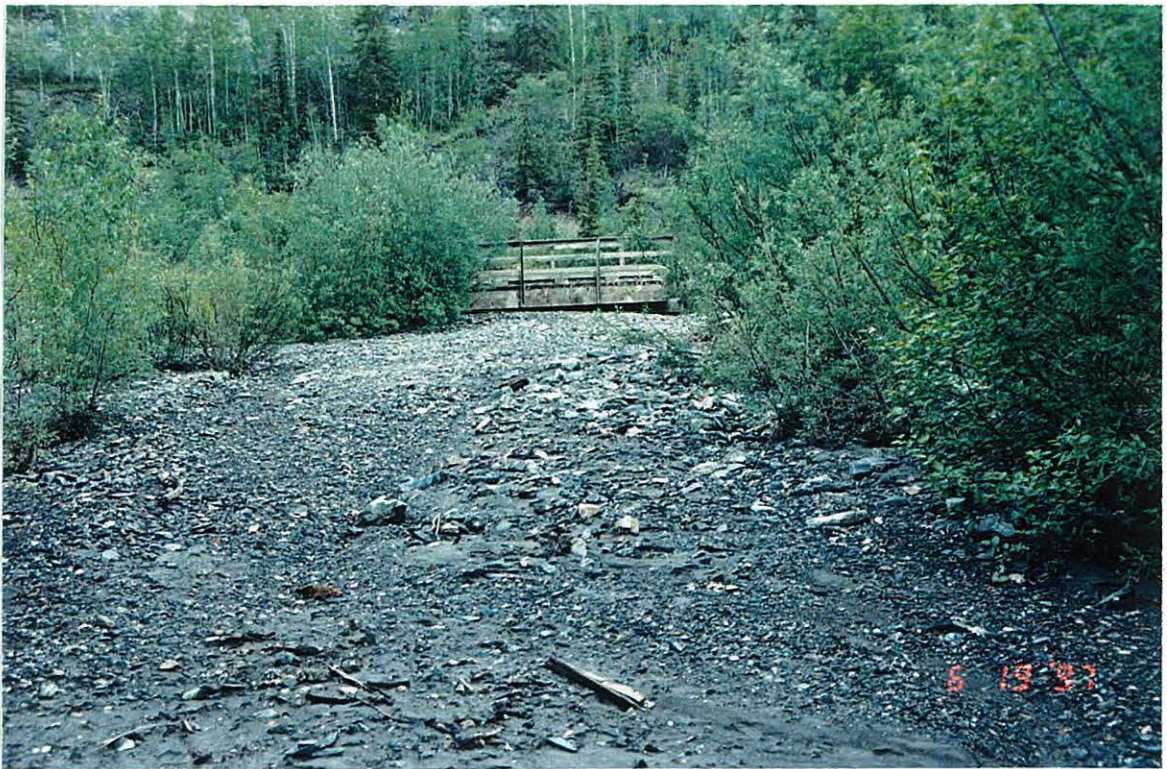
Photo 2: Original creek channel completely filled with debris; note the bridge.
