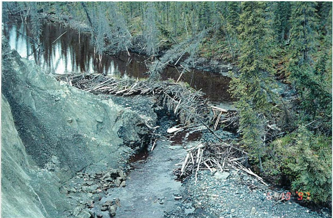
Photo 12: View of heaved creek bottom at the upstream end of the south tailings pile lobe.
