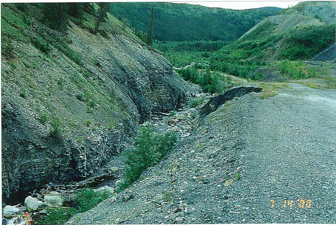
Photo 6: View of the downstream segment of the Clinton Creek channel. Note ongoing erosion of both channel banks.
