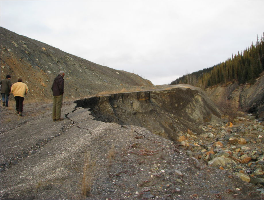
Erosion of road leading to lake outlet
