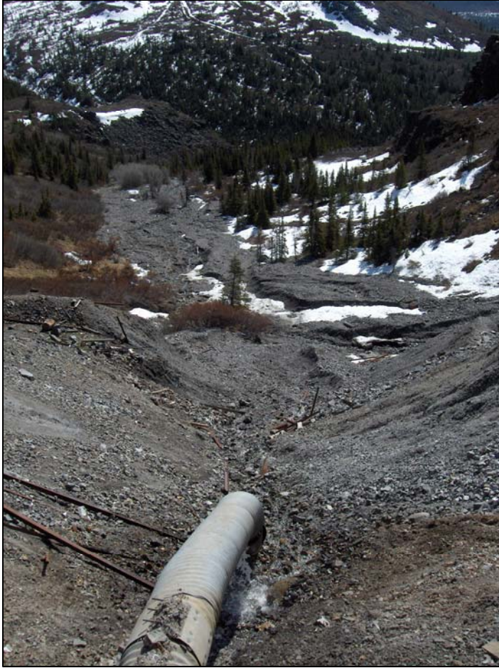
Plate 25: Keno 700 discharge path
