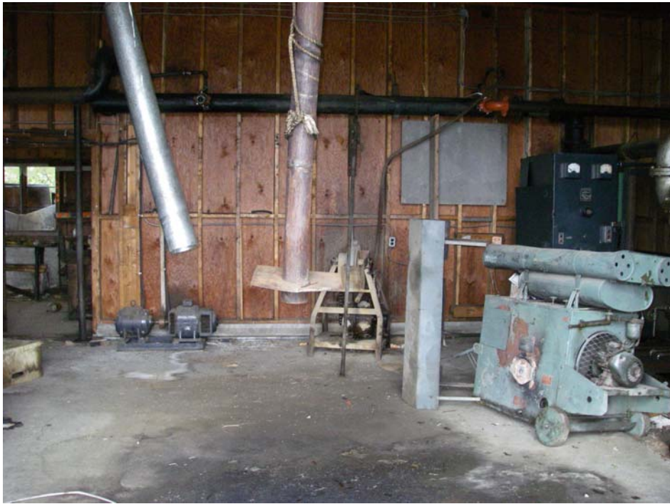
Photo #16: Concrete floor staining at Ruby 400
