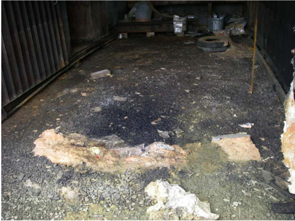
Photo #15: Interior floor staining at Dixie
