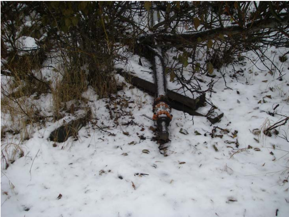
Photo #4: Fill pipe for AST at end of houses
