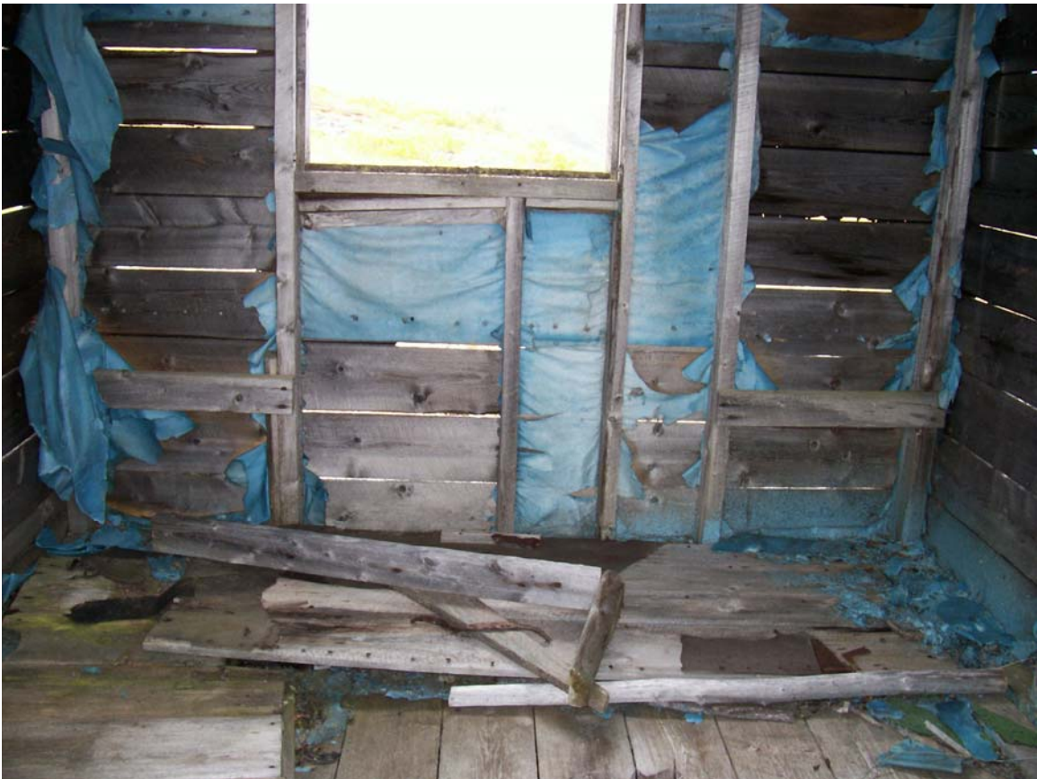
Possible building contamination at Main Fault & Nabob site.
