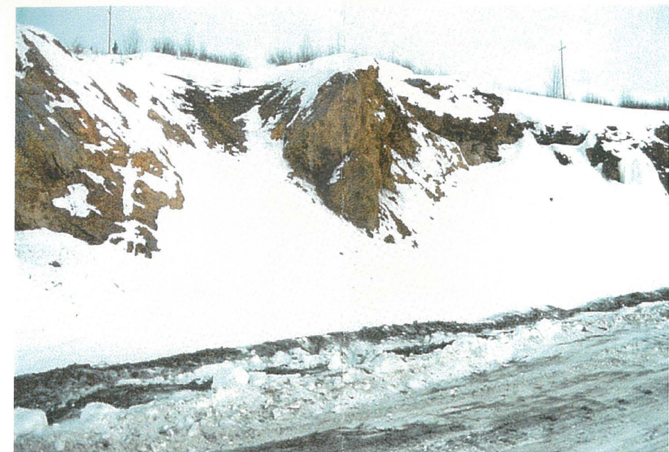
(February 12, 2001) Area to be excavated by trimming - prior to start of work.
