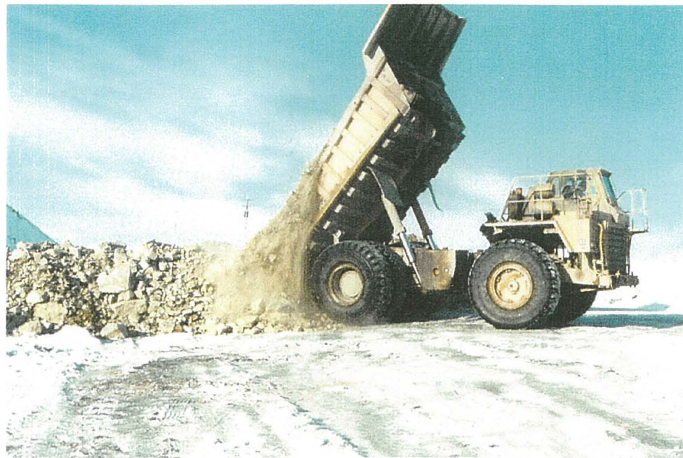
(February 15, 2001) Dumping riprap into stockpile, next to Grum Pit, on Vangorda Haul road.
