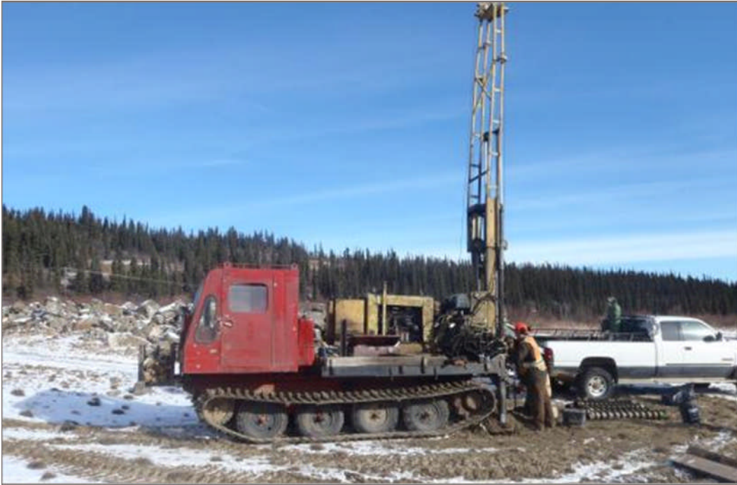
Photo 1: Nodwell mounted CME75 drill rig equipped with hollow stem augers Facing north (October 2, 2012)
