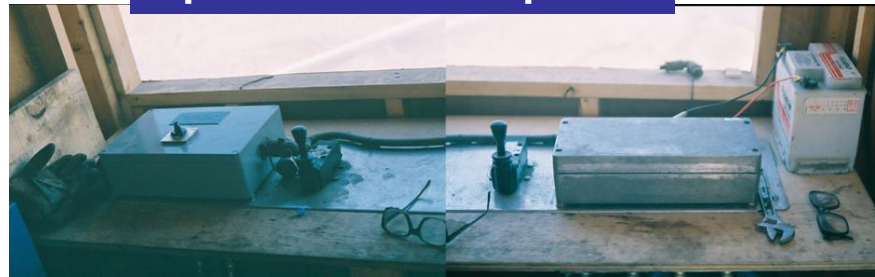
Operators control panel
