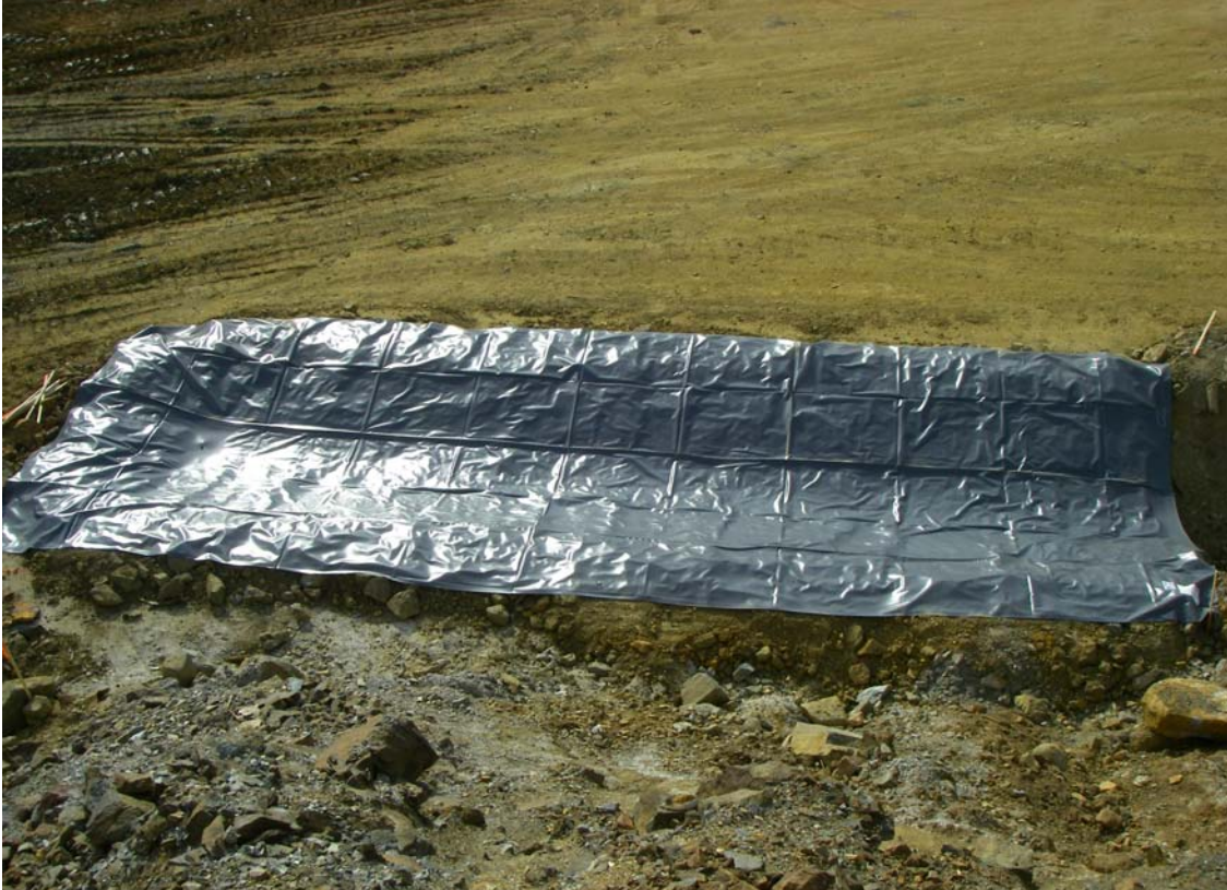
Photo 13: PVC liner placed on Test Pad 1. The drainage point is located in the right side of the photo.
