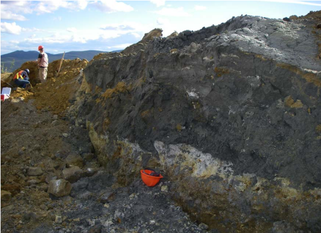
Photo1: The white colour band on the right side of the photo indicates the presence of precipitated acid salts at the waste-subgrade interface; 0.5 meter overexcavation evident. Students sampling the subgrade in the left side of the photo.
