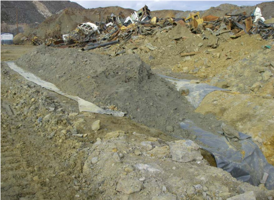
Photo 19: Flap of the PVC liner extended over the collection point of Test Pad 2. Each test pad had a 20 litre bucket installed at the collection point, and was covered with flaps of PVC liner to eliminate contamination of the drainage sample with dust or dilution with rain water.
