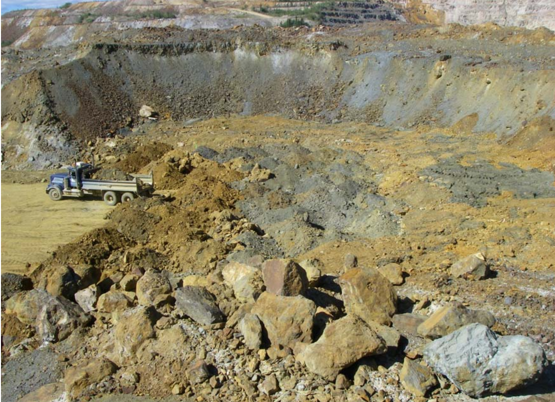
Photo 3: Relocated waste rock from S/P2 “bubble dumped” at the repository site on day 5. Material hauled on previous days pushed up and levelled in a bench against the original slope of LGSP‘C’.
