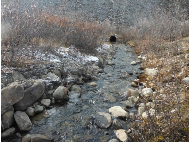
Photo 1. West Fork Vangorda Creek upstream of Haul Road ( VR ), looking downstream to Haul Road culvert.
