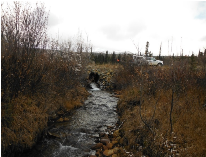
Photo 5. West Fork Vangorda Creek downstream of AEX Creek ( VW3 ), looking upstream to auxiliary road culvert.
